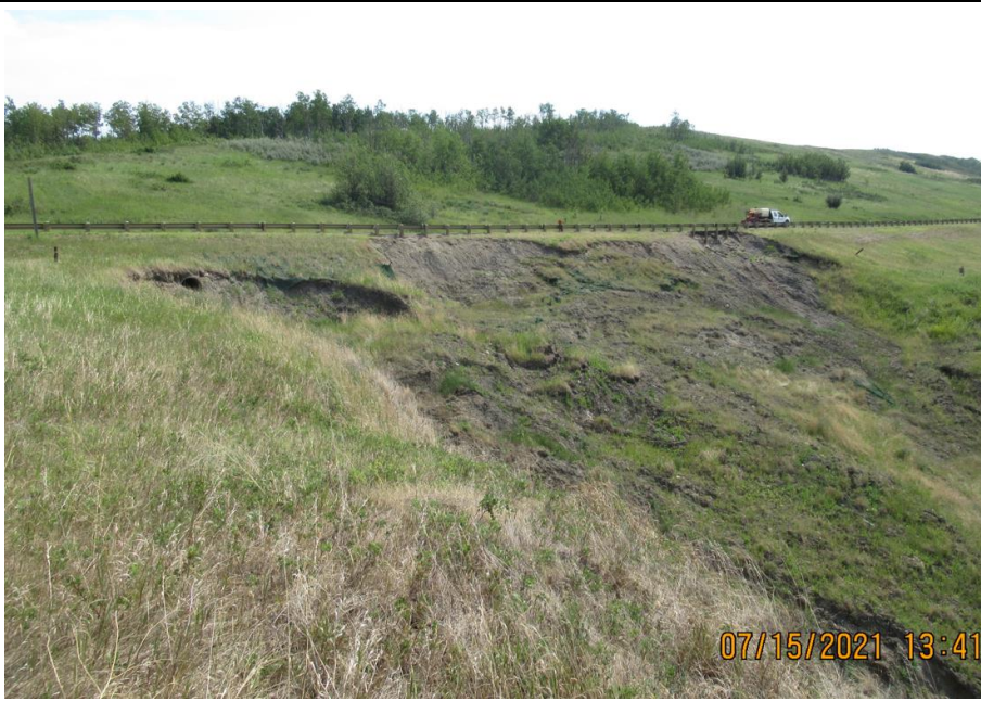
Photo 12. Looking southeast towards the 1+400 slide. The slide has further retrogressed towards the highway, is wider than in 2020 and there is a 5 m to 7.5 m drop below the guardrail.
