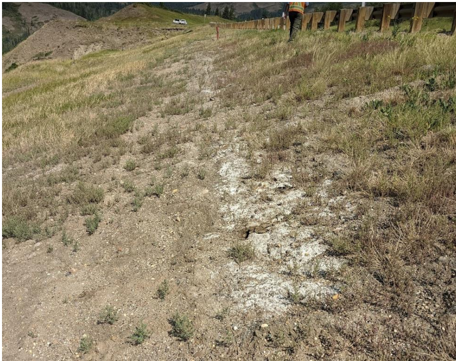
Photo 8. Looking north near Sta. 1+550 at rough area (drill access bench) with some seepage and tension cracks
