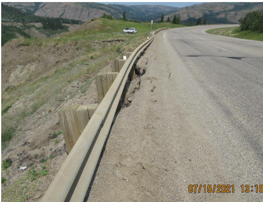
Photo 10. Looking north from Sta. 1+450 backscarp. The slide scarp has retrogressed since 2020 and cracks are now 0.1 m west of the white line.
