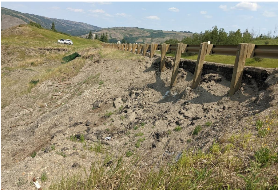
Photo 9. Looking northwest across soil matting and nails which were installed in August 2010 at Sta. 1+450 slide. Backscarp (5 m to 7.5 m high) continues to retrogress and is now impacting the highway. Two guardrail posts are hanging and other two posts are partially exposed.
