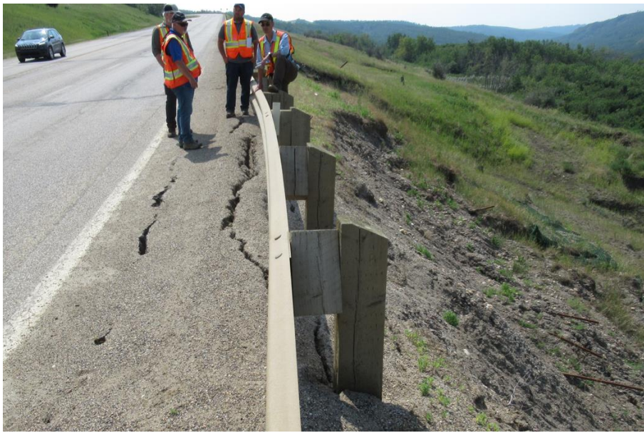
Photo 11. Looking south from Sta. 1+390 at the backscarp of the 1+400 slide which is impacting the highway shoulder. Slide crack is 60 mm wide and is 0.3 m from white line plus two other cracks closer to the guardrail
