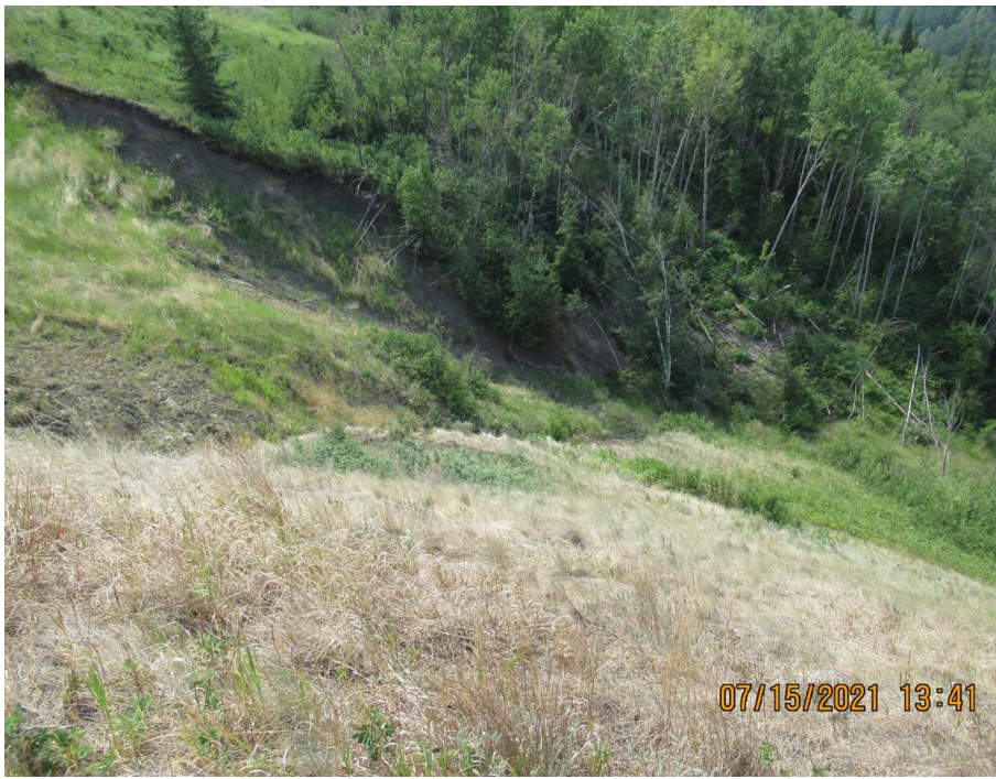
Photo 13. Looking south at the fresh slump slide that is impacting the highway at Sta. 1+400.
