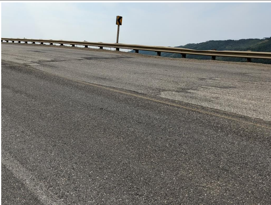
Photo 6. Looking northeast across the dip in the highway at the south end of the 1+800 slide.
