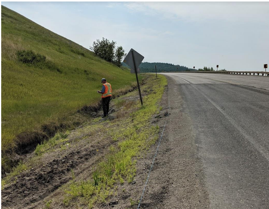
Photo 5. Looking south from Sta. 1+800 at the new ACP patch placed in 2020 and the erosion gully developed on the ditch up to 1.6 m wide and 0.6 m deep.
