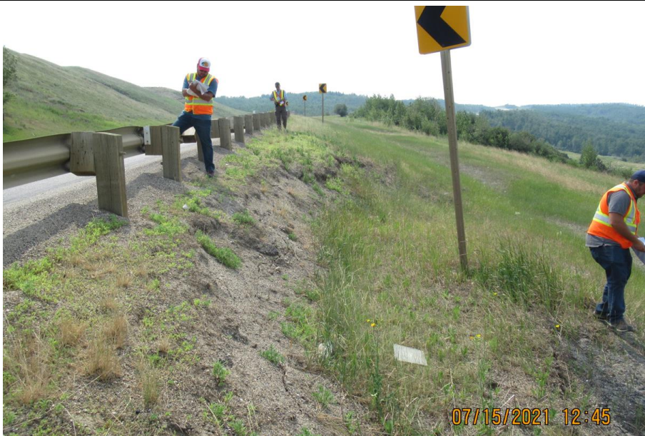
Photo 4. Looking south from Sta. 1+890 at the slump in the sideslope of the SBL. The scarp is 1.1 m high and 0.8 m from the guardrail.
