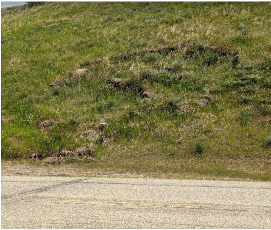
Photo 3. Looking east at backslope skin failure at Sta. 1+900 (More movement since 2020).
