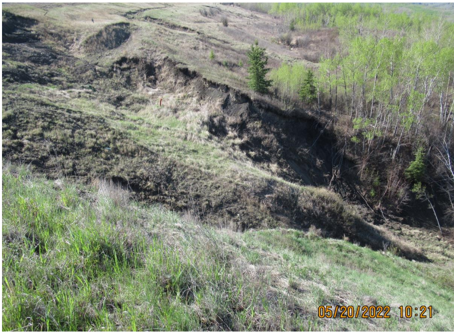
Photo 13. Looking south at the fresh slump slide that is impacting the highway at Sta. 1+400.
