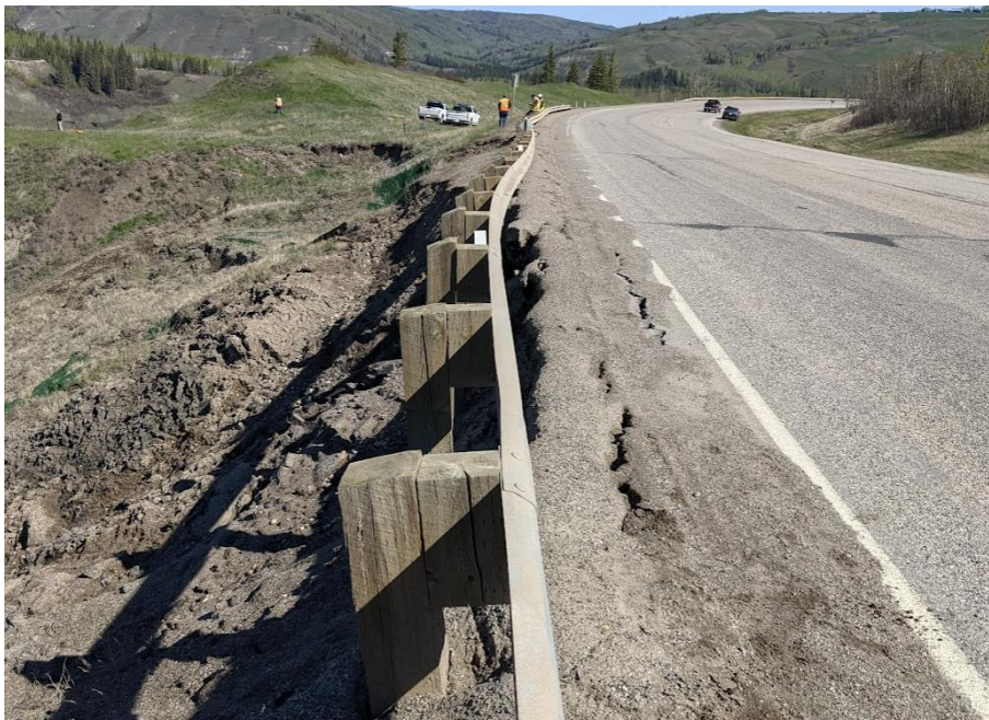
Photo 10. Looking north from Sta. 1+450 backscarp. The slide scarp cracks up to 200 mm wide just west of the white line.
