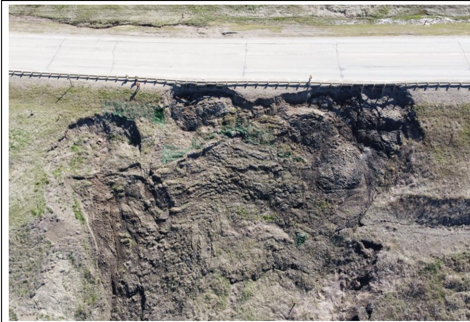
Photo 15. Drone photo of the backscarp of the 1+400 slide impacting the highway shoulder.
