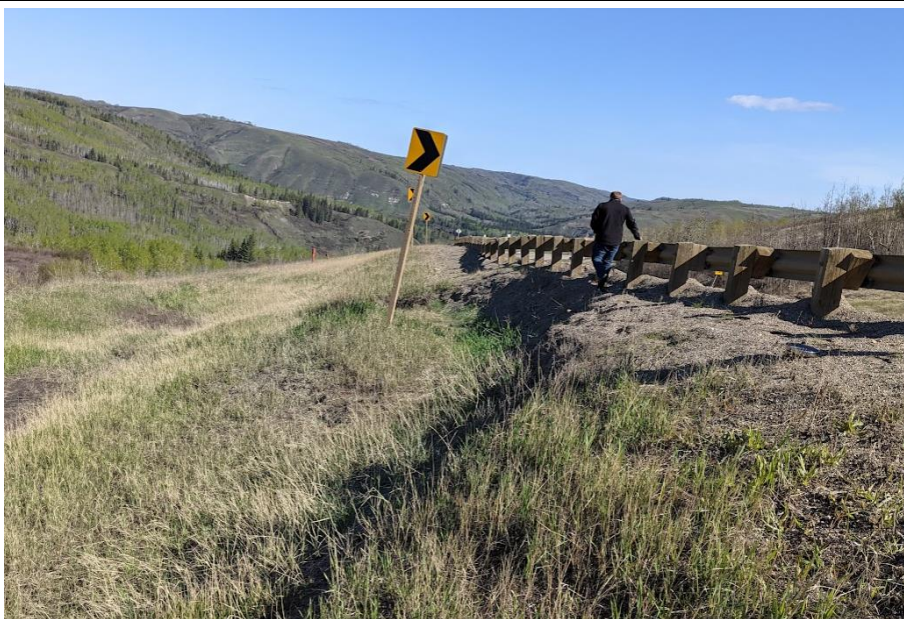
Photo 4. Looking north from Sta. 1+890 at the slump in the sideslope of the SBL. The scarp is 1.1 m high and 0.8 m from the guardrail.
