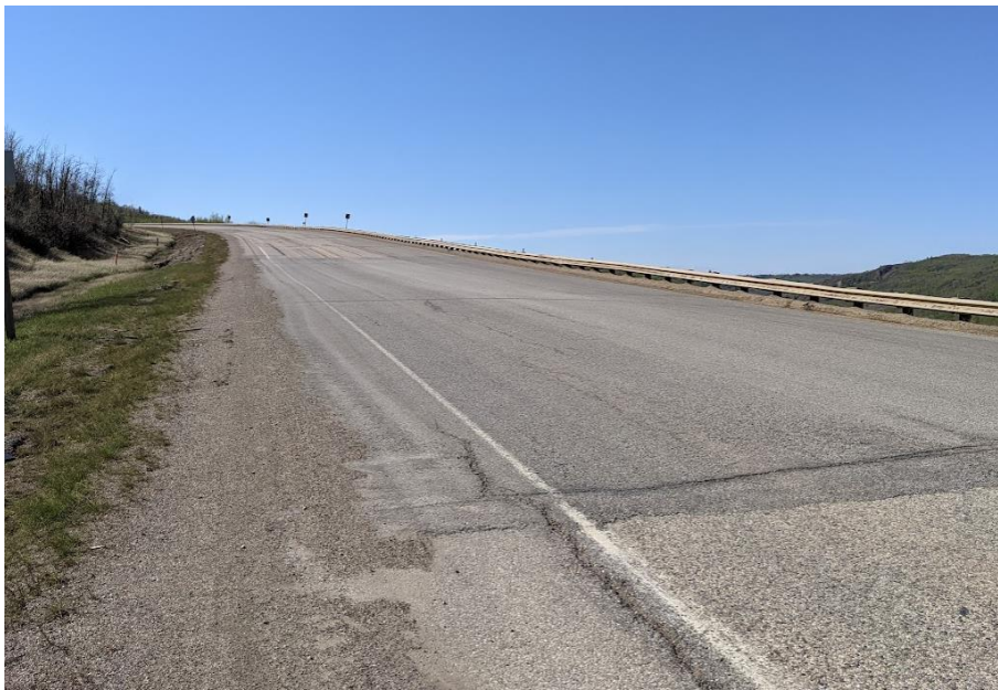
Photo 7. Looking from the shoulder of the SBL at Sta. 1+660 across the dip in the highway at the north end of the 1+800 slide.
