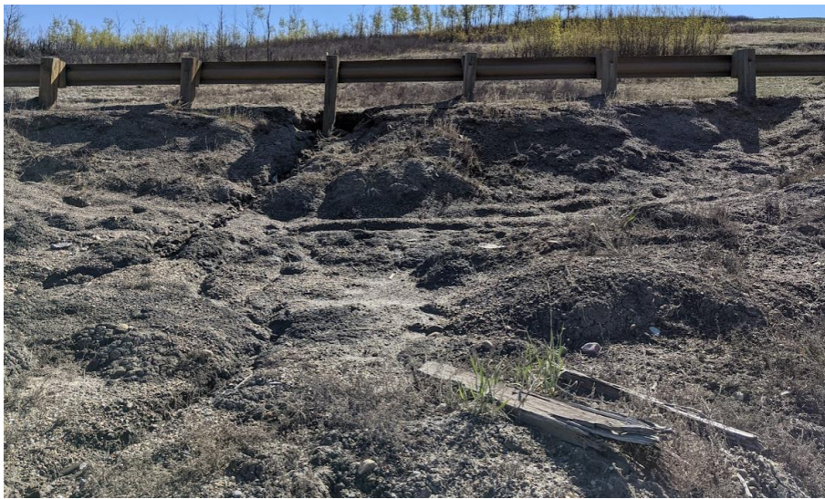
Photo 9. Looking west across soil matting and nails which were installed in August 2010 at Sta. 1+450 slide. Backscarp (5 m to 7.5 m high) continues to retrogress and is now impacting the highway. Two guardrail posts are hanging and other two posts are partially exposed.
