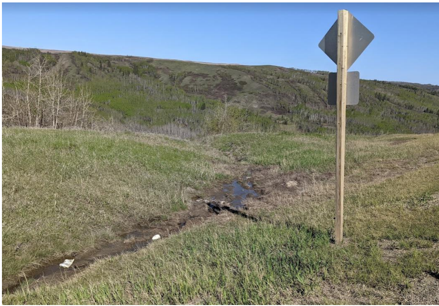
Photo 1. Looking northwest from Sta. 2+000 at erosion gully in SBL ditch south of ditch block
