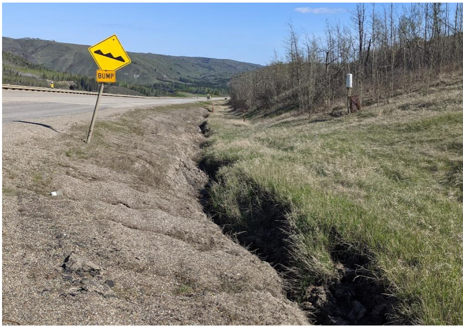
Photo 5. Looking north from Sta. 1+800 at the erosion gully developed on the ditch up to 3.3 m wide and 0.8 m deep. Erosion gully wider and deeper than noted at the 2021 inspection
