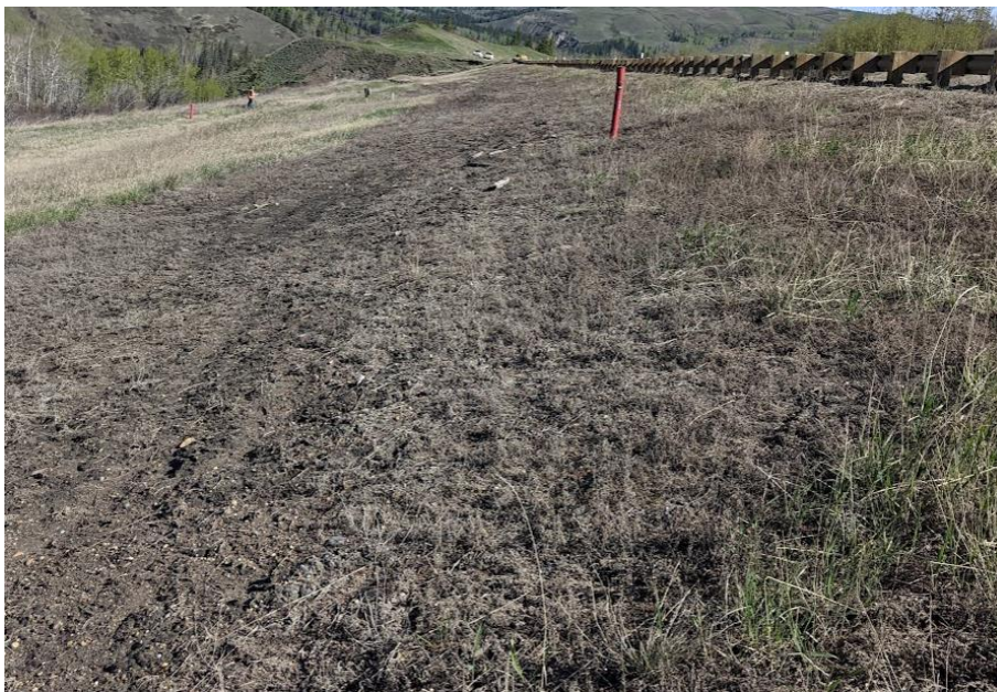
Photo 8. Looking north near Sta. 1+550 at rough area (drill access bench) with some seepage and tension cracks
