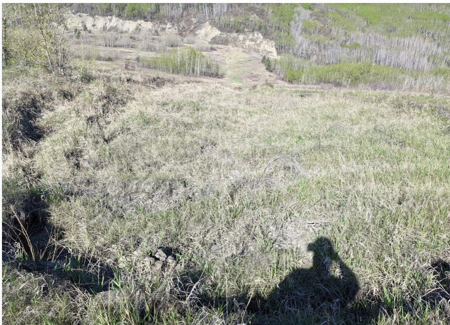
Photo 2. Looking west from Sta. 1+980 below the SBL highway. More movement noted in 2022
