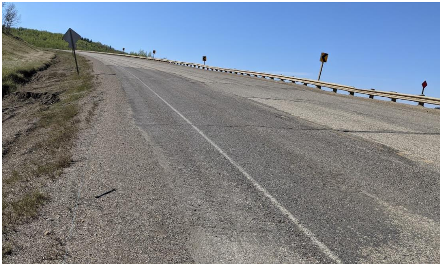
Photo 6. Looking northeast across the dip in the highway at the south end of the 1+800 slide.
