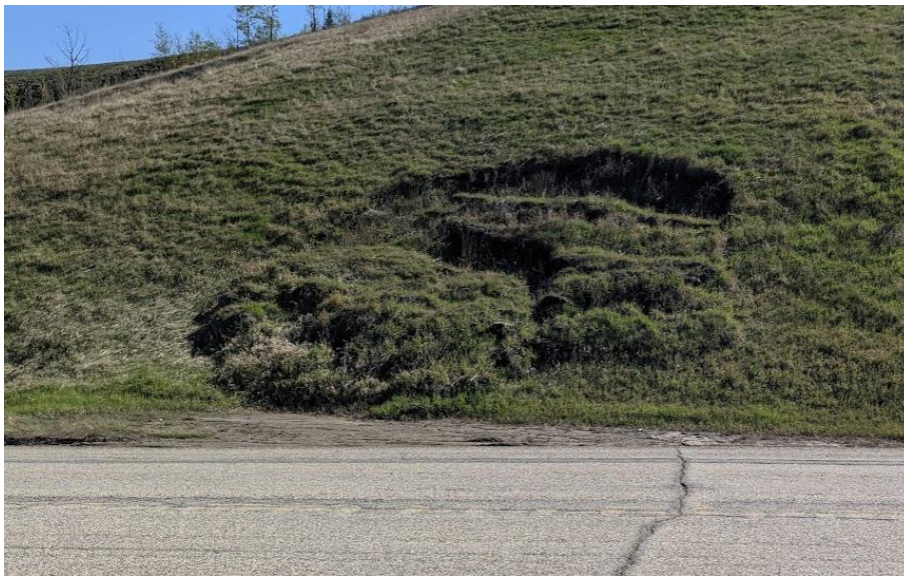
Photo 3. Looking east at backslope skin failure at Sta. 1+900 (More movement since 2021).
