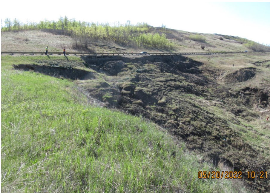
Photo 12. Looking southeast towards the 1+400 slide. The slide has further retrogressed towards the highway, is wider than in 2021 and there is a 5 m to 7.5 m drop below the guardrail.
