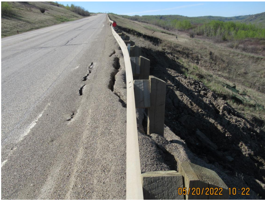
Photo 11. Looking south from Sta. 1+390 at the backscarp of the 1+400 slide which is impacting the highway shoulder. Slide cracks are wider and closer to the white line
