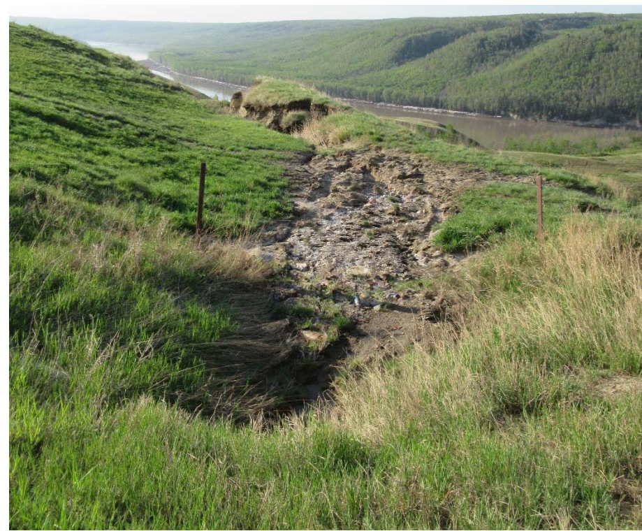
Photo 9. Looking southeast from north of the centerline culvert outlet towards the scour channel. No significant change since 2017.
