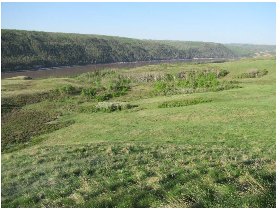
Photo 16. Looking southwest downslope of the Dunvegan North landslide repair. The grass catch is still good downslope of the repair. No significant change since 2017.
