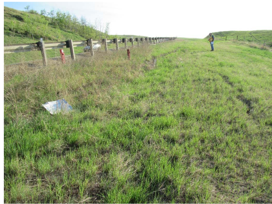
Photo 6. Looking northeast along the graben forming in the passive bench below the pile wall. The graben varies in width from 4 m at the west end to 1.5 m at the east end of the pile wall.
