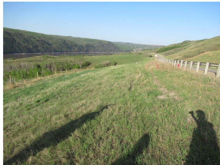
Photo 5. Looking southwest along the buried cantilever pile wall built in 2015. The graben in the passive bench below the wall is more apparent since 2017 with cracks open to 180 mm with a 200 mm drop.
