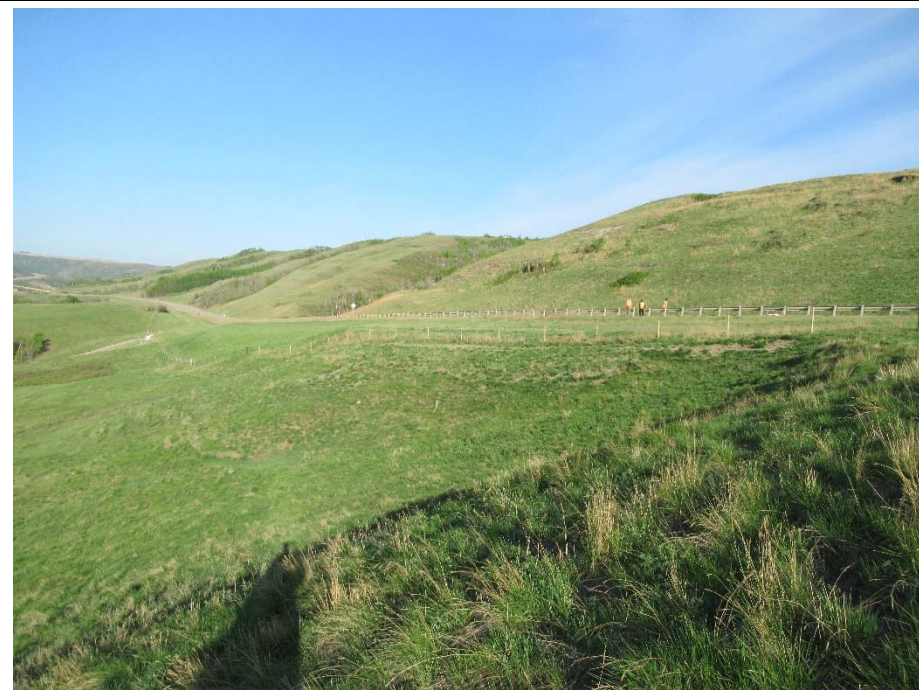
Photo 14. Looking west towards the Dunvegan North landslide repair. The grass catch is still good downslope of the repair.
