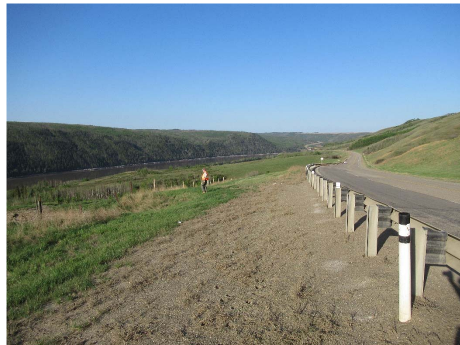
Photo 3. Looking southwest from east of the new pile wall built in 2015/2016. The pile wall is buried below ground. Grass catch is sparse east of the pile wall (foreground).
