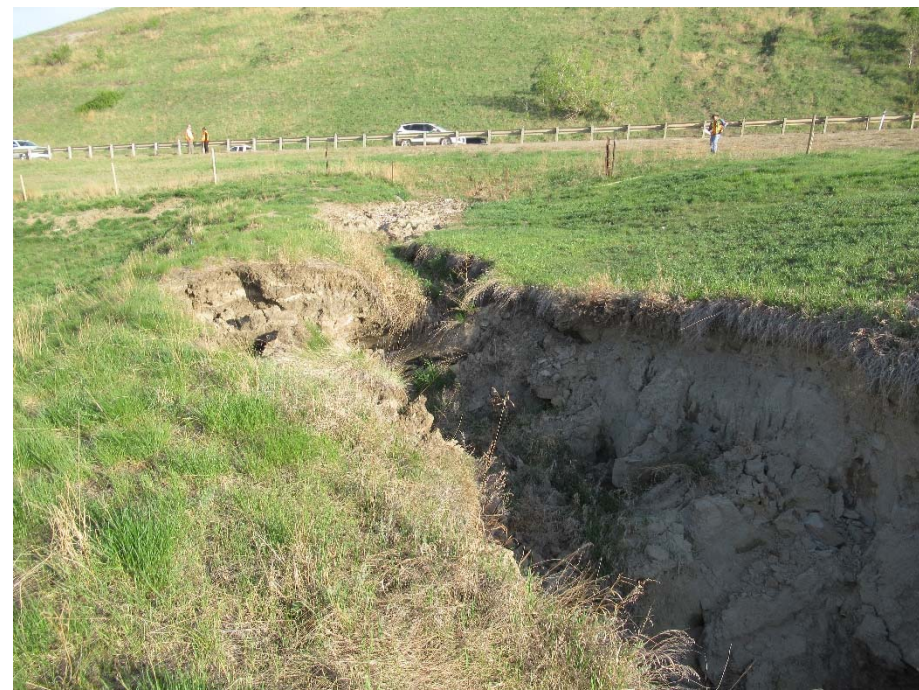
Photo 13. Looking northwest from the north end of the scour channel towards the outlet of the centerline culvert.
