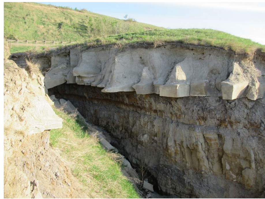
Photo 11. Looking north from the west side of the scour channel that is situated below the outlet of the centerline culvert.
