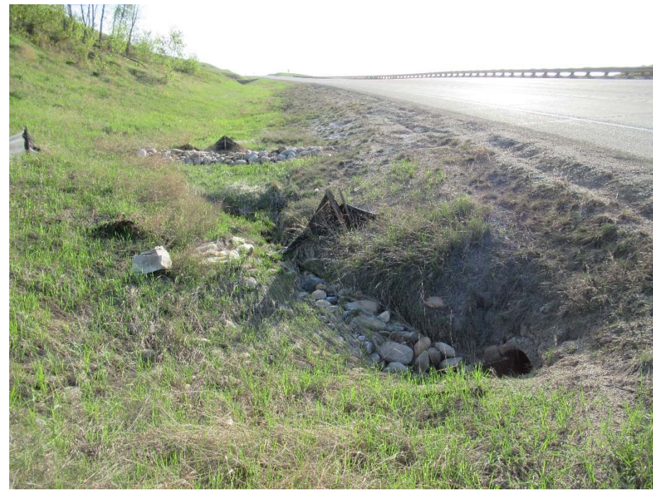
Photo 2. Looking northeast at inlet to 600 mm diameter CSP and rock berm. No significant change since 2017.
