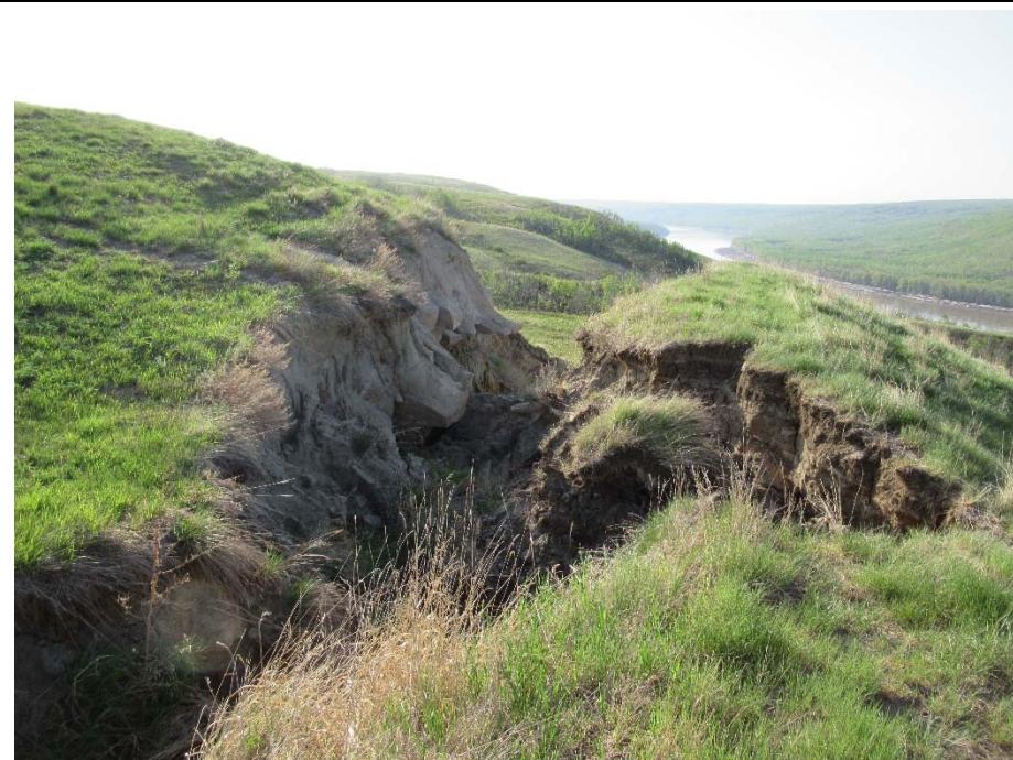
Photo 10. Looking southeast from the north end of the scour channel that has developed below the outlet of the centerline culvert. The scour is slightly wider and there are no signs of retrogression towards the highway since 2017.
