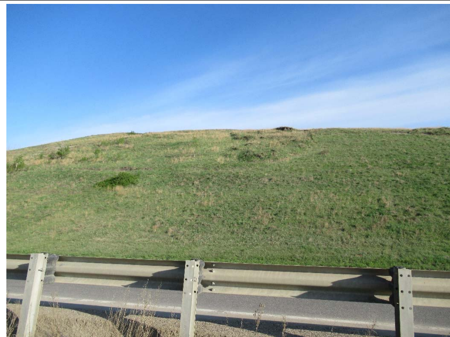
Photo 8. Looking northwest from the new pile wall at the skin failures in the backslope above the highway.
