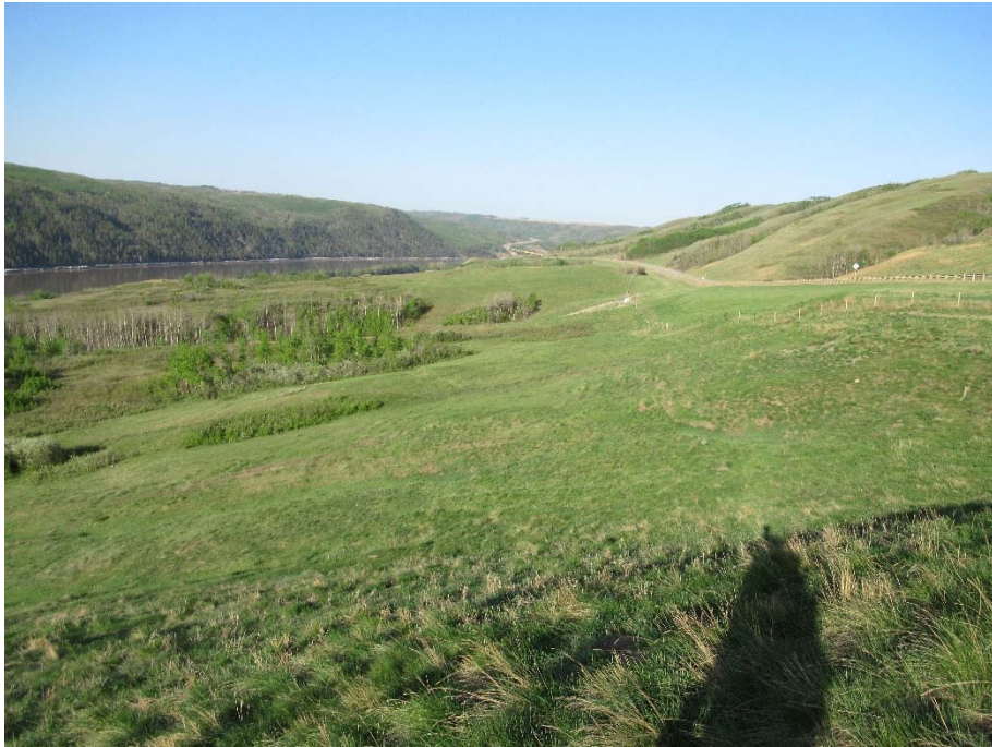
Photo 15. Looking southwest towards the Dunvegan North landslide repair. The grass catch is good downslope of the repair. The old toe bulge is still distinct.
