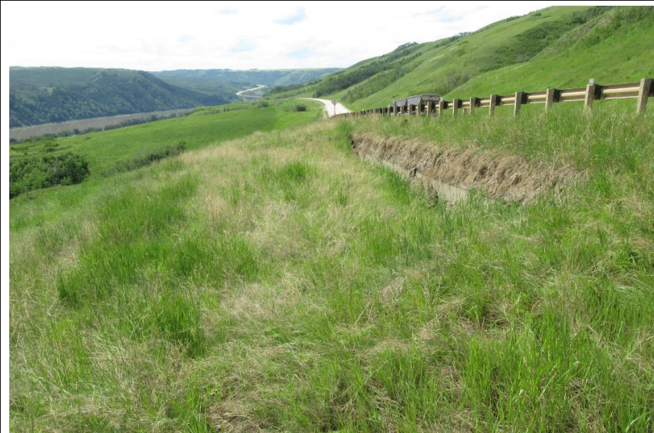
Photo 2. Looking southwest along the pile wall built in 2015/2016. The soil below the pile wall is slumping, exposed a portion of the pile wall, and created a well-defined graben bench.
