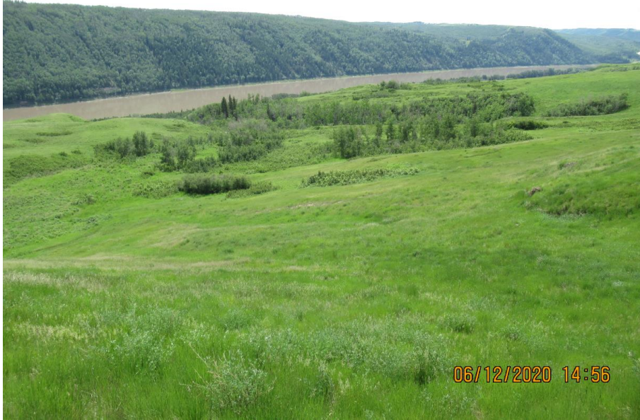
Photo 5. Looking south towards the Dunvegan North landslide repair. The grass catch is still good downslope of the repair.
