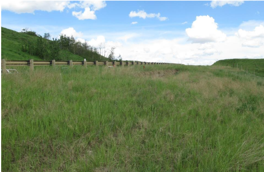
Photo 3. Looking northeast along the graben formed in the passive bench below the pile wall.
