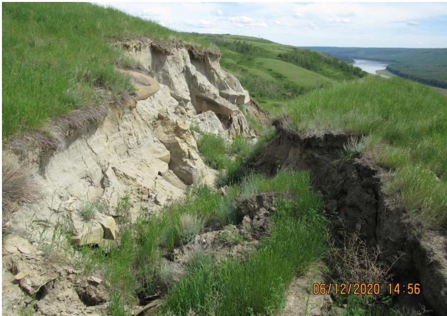
Photo 8. Looking southeast from the north end of the scour channel that has developed below the outlet of the centerline culvert. The scour is slightly wider and is retrogressing towards the highway since 2018.
