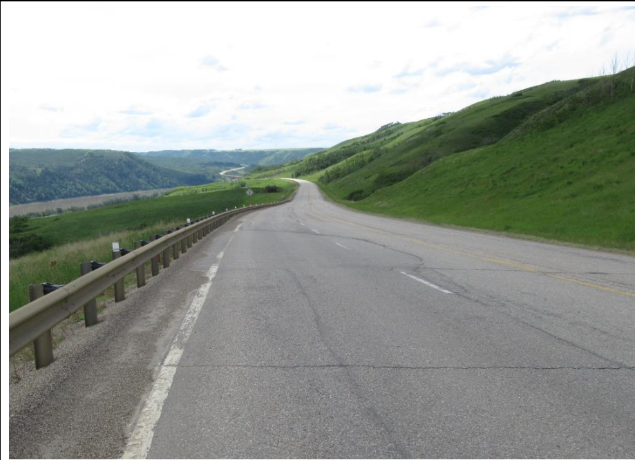
Photo 1. Looking SW from the NBL of Hwy 2:68 towards the 2015/2016 landslide repair under Alberta Transportation Contract CON0017398. Reflective cracks became visible.
