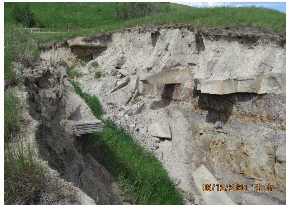
Photo 11. Looking northwest from the north end of the scour channel towards the outlet of the centerline culvert. Note grass growing at the bottom of the gully and bird burrows on the upper weathered sandstone layer
