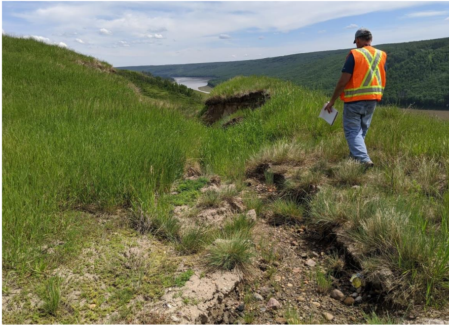
Photo 7. Looking southeast from north of the centerline culvert outlet towards the scour channel.
