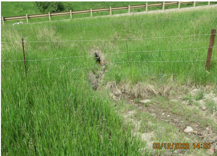
Photo 6. Looking at the 600 mm centre line culvert outlet. Erosion downstream of the outlet is still occurring
