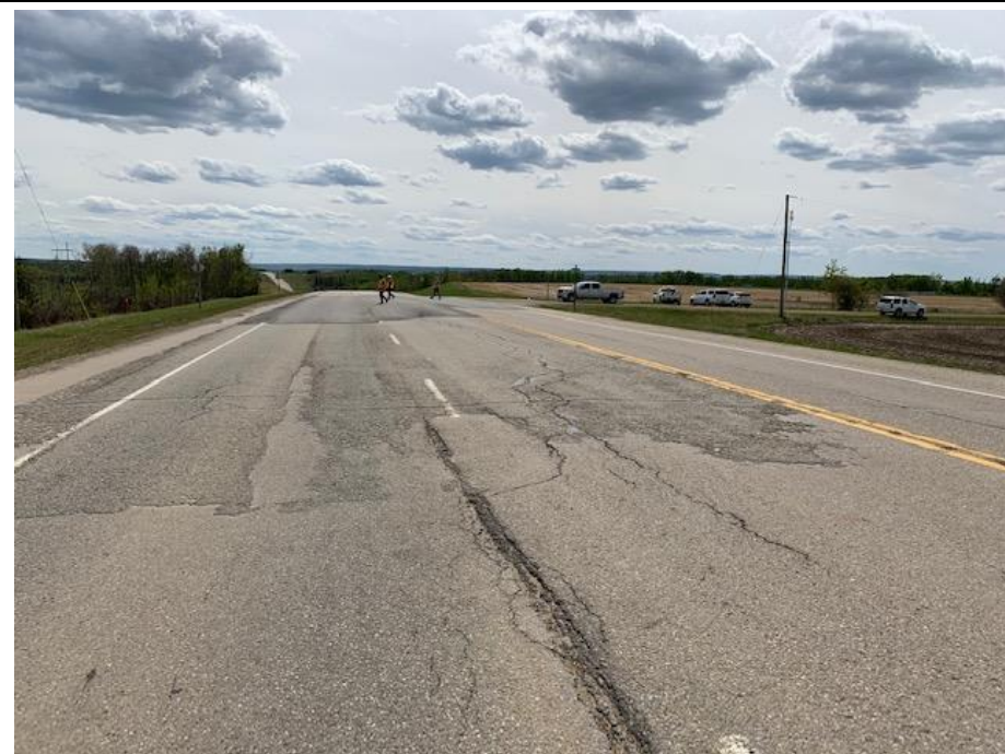
Photo 2. Looking closer at cracks in northeast inner NB passing lane at cracks in ACP patch.
