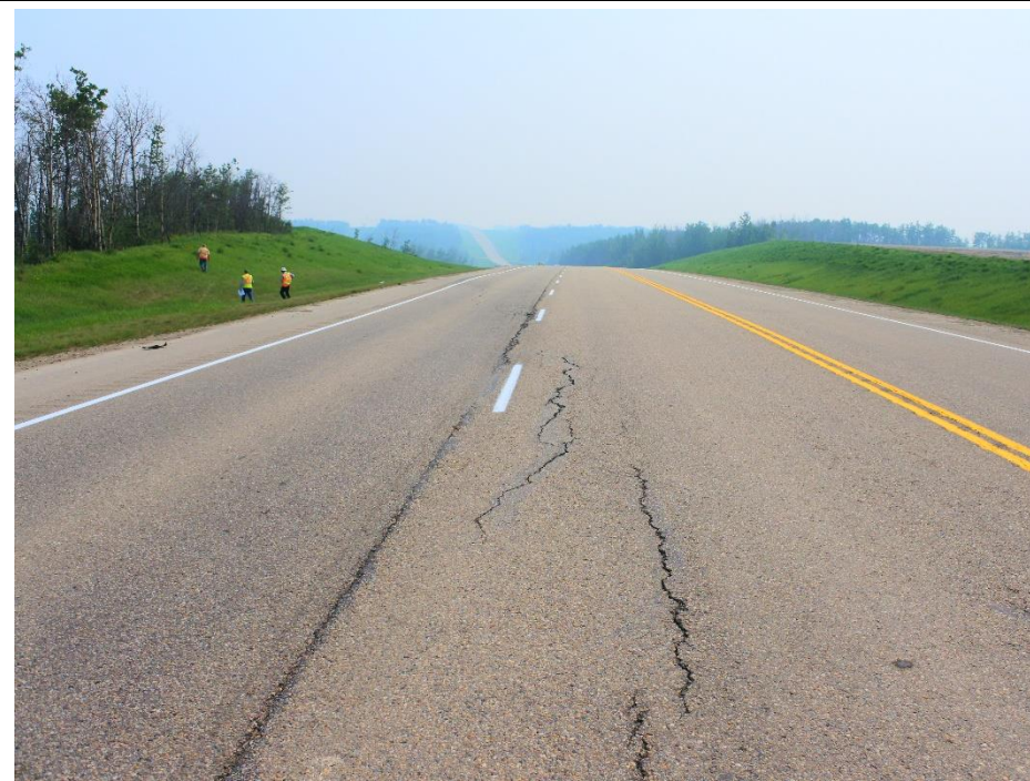
Photo 8. New cracks observed crossing both NBL.
