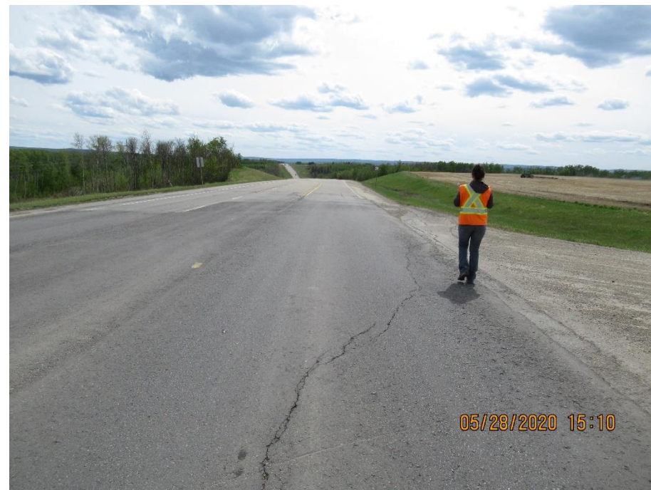
Photo 3. Looking south standing near Township Road 771 looking at crack in the SBL.
