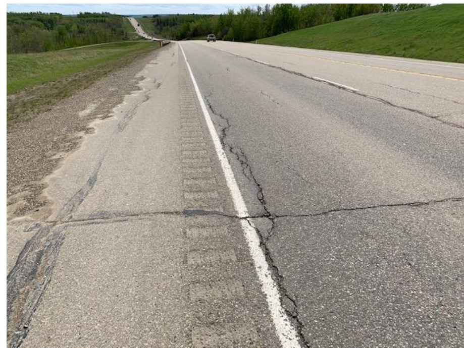
Photo 5. New cracks observed crossing both NBL and extending into the shoulder.
