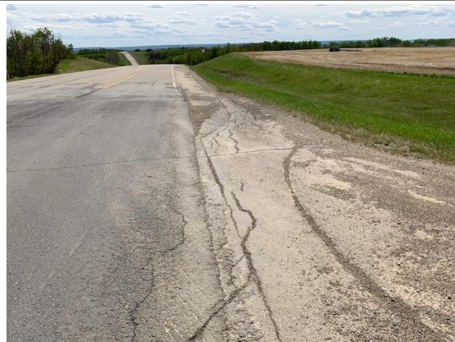
Photo 4. Looking south at the cracks in the SBL shoulder just south of Township Road 771.
