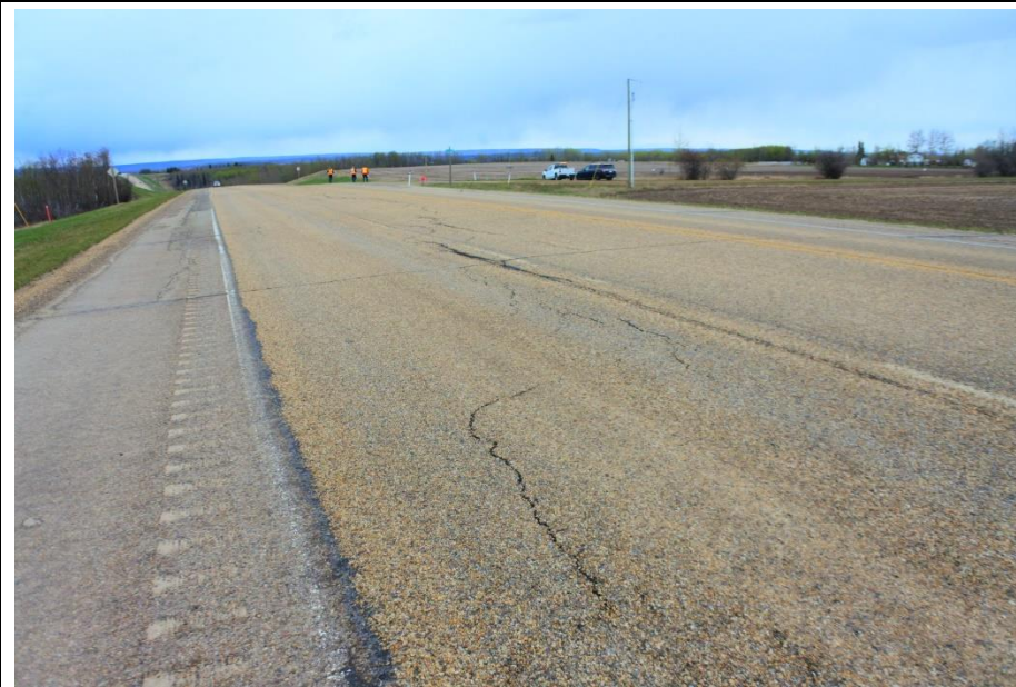
Photo 2. Looking at cracks in ACP patch in the northeast outer NB passing lane.
