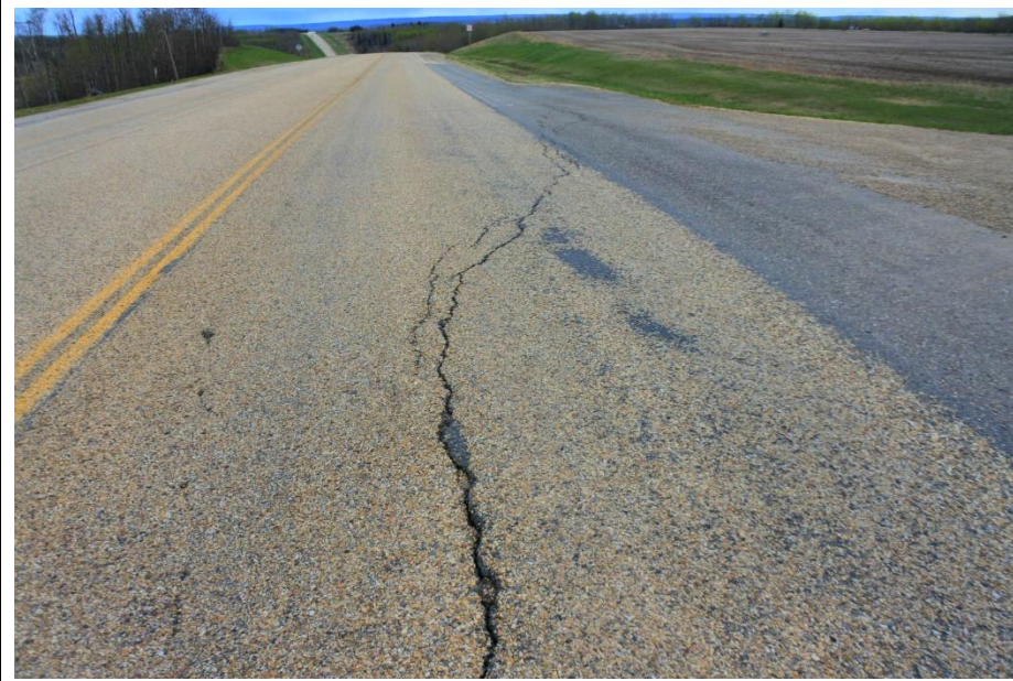
Photo 3. Looking south standing near Township Road 771 looking at crack in the SBL.
