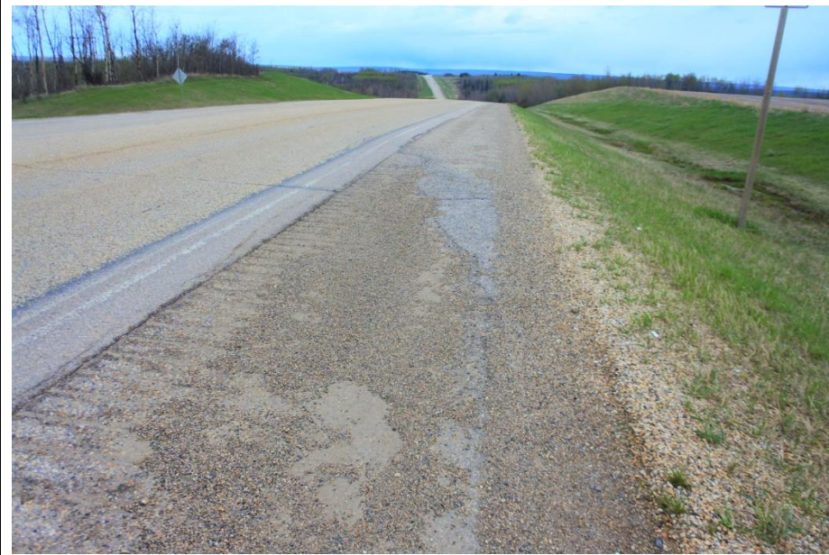
Photo 4. Looking south at the cracks in the SBL shoulder just south of Township Road 771.
