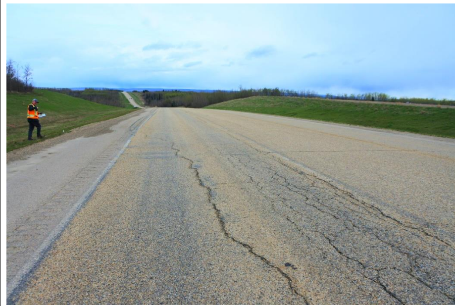
Photo 5. Looking south at cracks observed crossing both NBL and extending into the shoulder.
