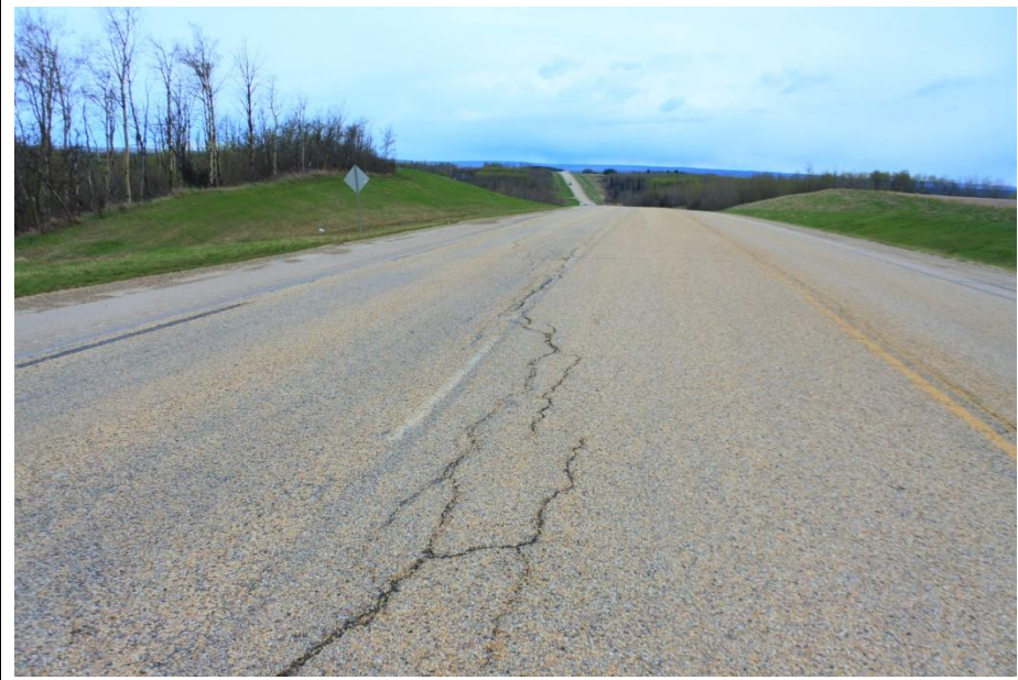
Photo 8. Looking south at cracks observed crossing both NBL.
