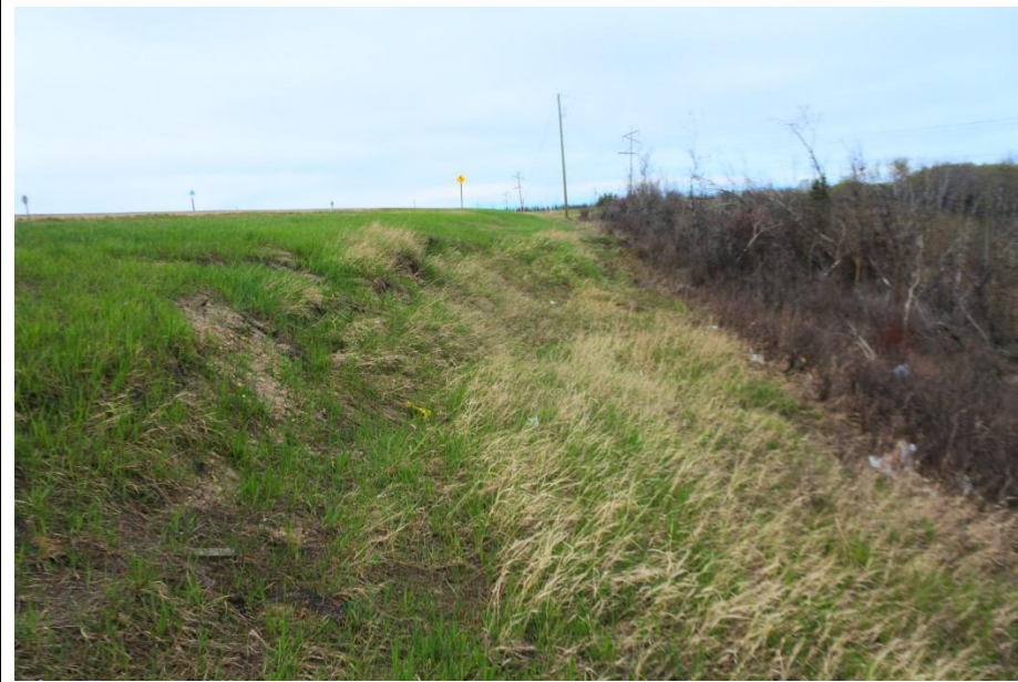
Photo 6. Looking north from highway embankment to the east where scarp crack was observed and was slightly more grown over in 2022.
