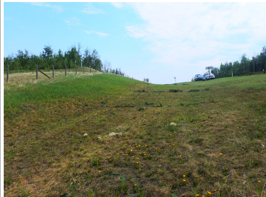
Photo 5. Looking southeast at water dissipation barriers that are tattered and in poor condition.
