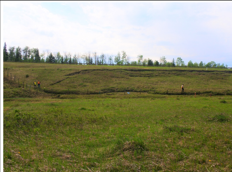
Photo 3. Looking southwest towards the landslide in the toe berm.
