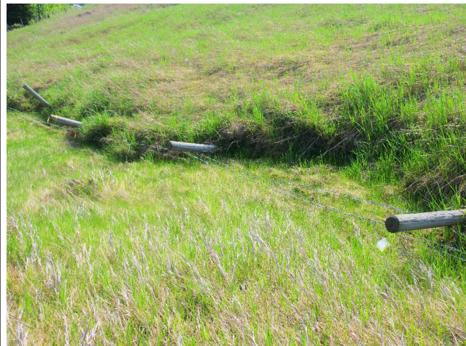
Photo 7. Looking at the toe bulge and bent over posts
