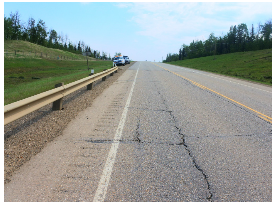
Photo 2. Looking southeast from the northbound lane at cracking in pavement.
