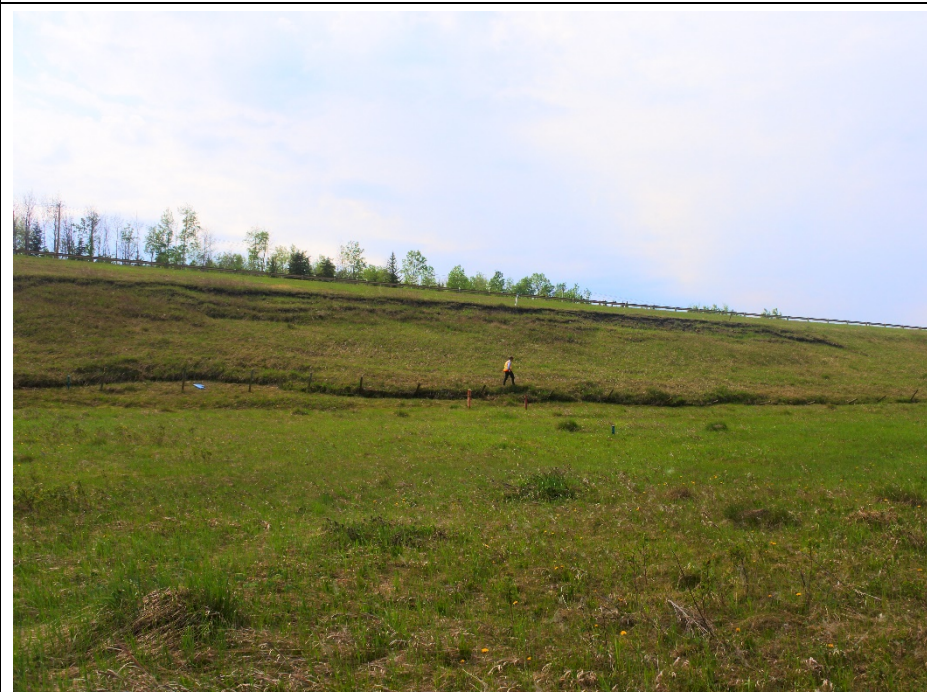
Photo 4. Looking west towards the landslide in the toe berm.
