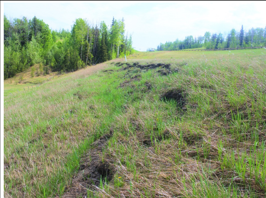
Photo 9. Looking southeast at relatively grownover slumping from head scarp.
