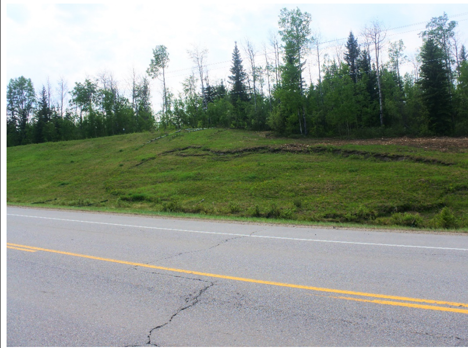
Photo 1. Looking southwest at backslope failure on other side of highway.
