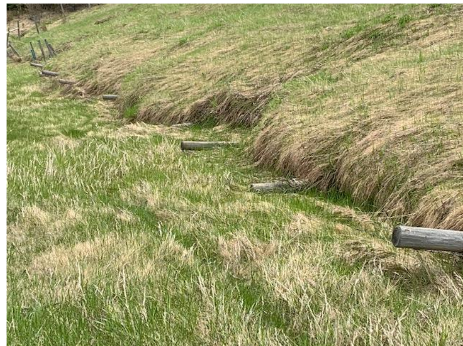
Photo 6. Looking at the toe bulge and bent over posts
