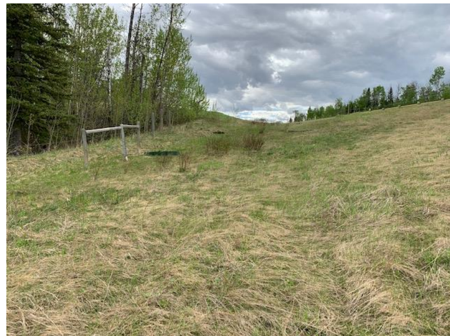
Photo 4. Looking southeast at water dissipation barriers that are tattered and in poor condition.
