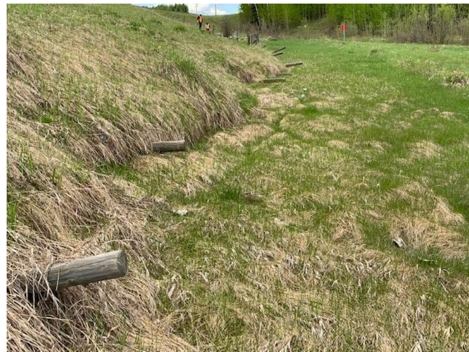
Photo 5. Looking northwest along the toe of the landslide. The fence posts are bent over further from movement of the toe bulge.
