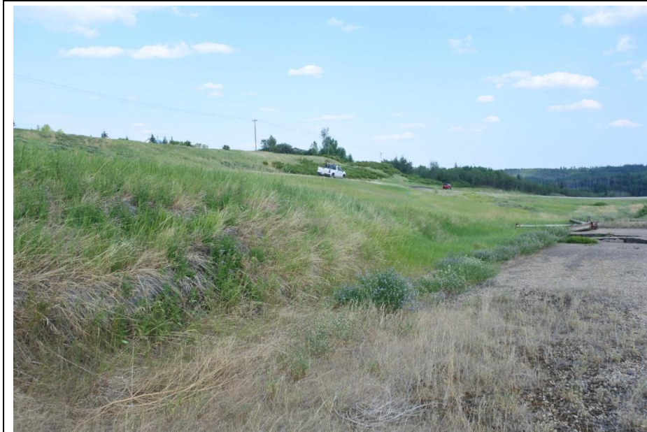
Photo 4. Looking northeast at southern slide scarp which crosses the old highway alignment.
