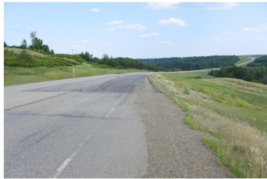
Photo 7. Looking east from the shoulder of the EBL of Hwy 49:06 across the inner crack feature and dip in the 2017 ACP patch.
