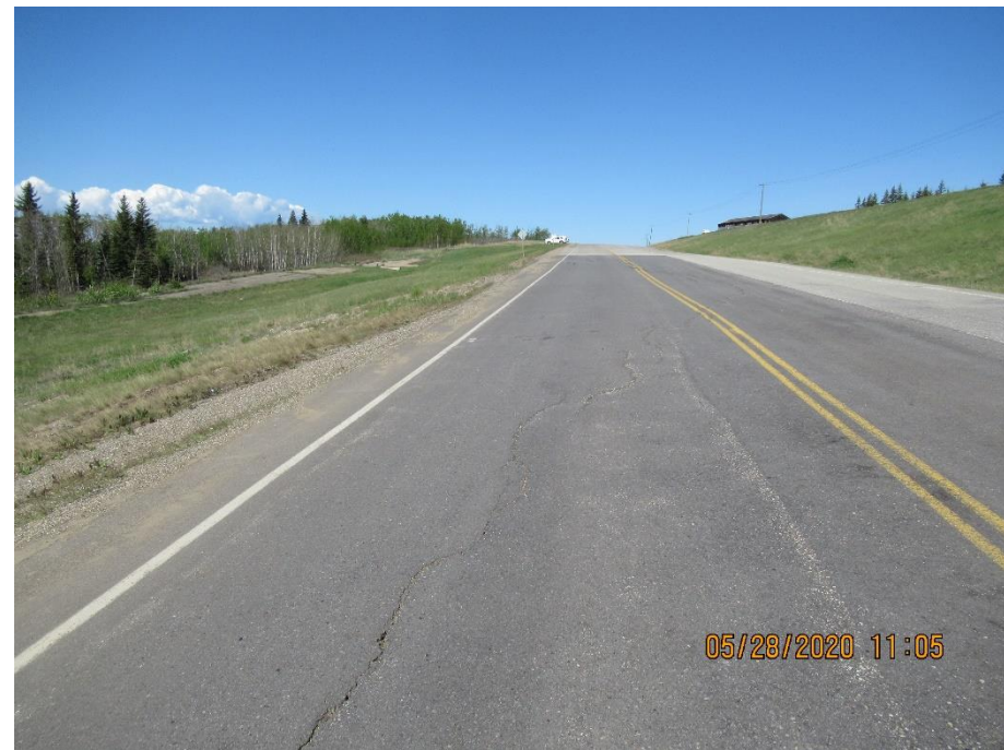
Photo 8. Looking northwest from the middle of Hwy 49:06 from the south end of the 2016 ACP patch.
