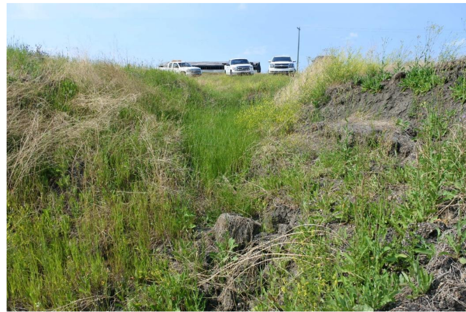
Photo 2. Looking northwest from edge of erosion gully. Note the ditch along east side of highway tails off and has been the contributor to this erosion.
