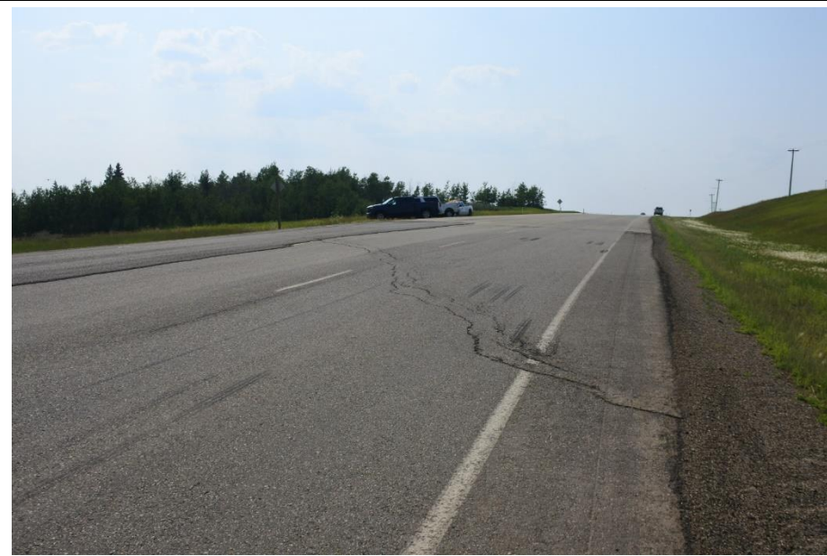
Photo 12. Looking northwest from the EBL shoulder of Hwy 49:06 at scarp crack extending into shoulder at the south end of the site.
