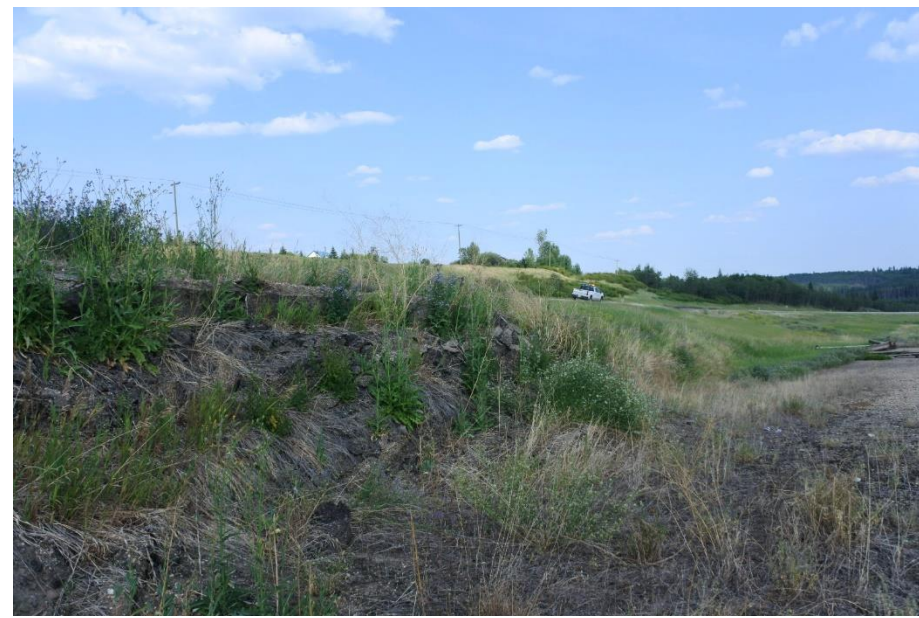
Photo 5. Looking southeast from old highway alignment at south slide scarp.
