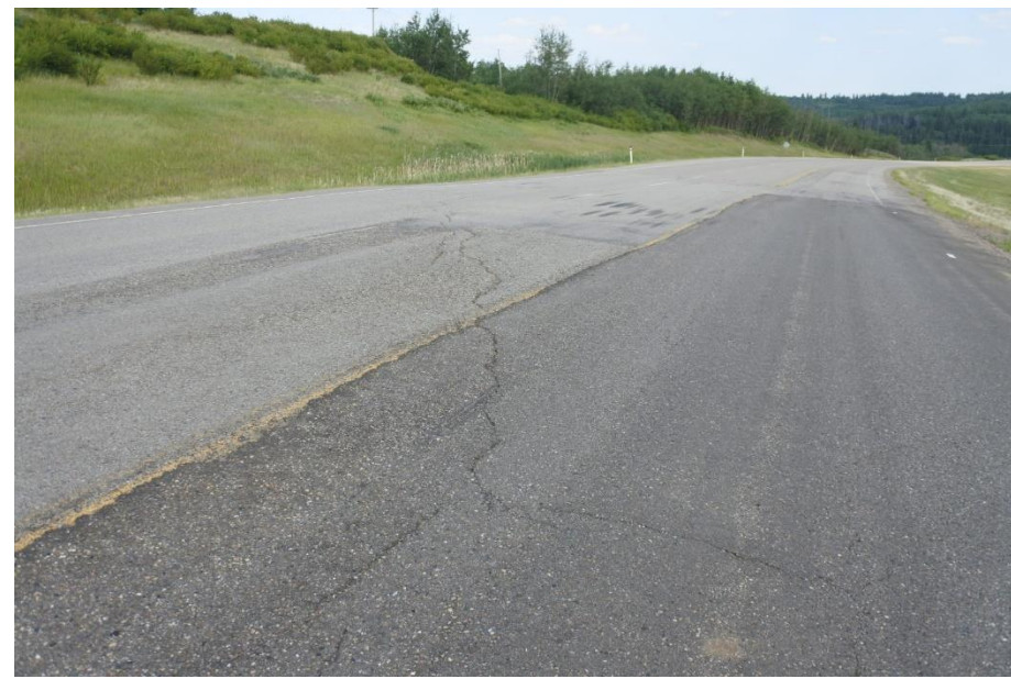
Photo 9. Looking east from near the middle of the 2017 ACP patch where crack continues into WBL.
