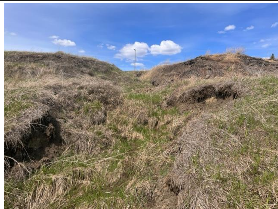
Photo 2. Looking north from edge of erosion gully. Note the ditch along south side of highway tails off and has been the contributor to this erosion.
