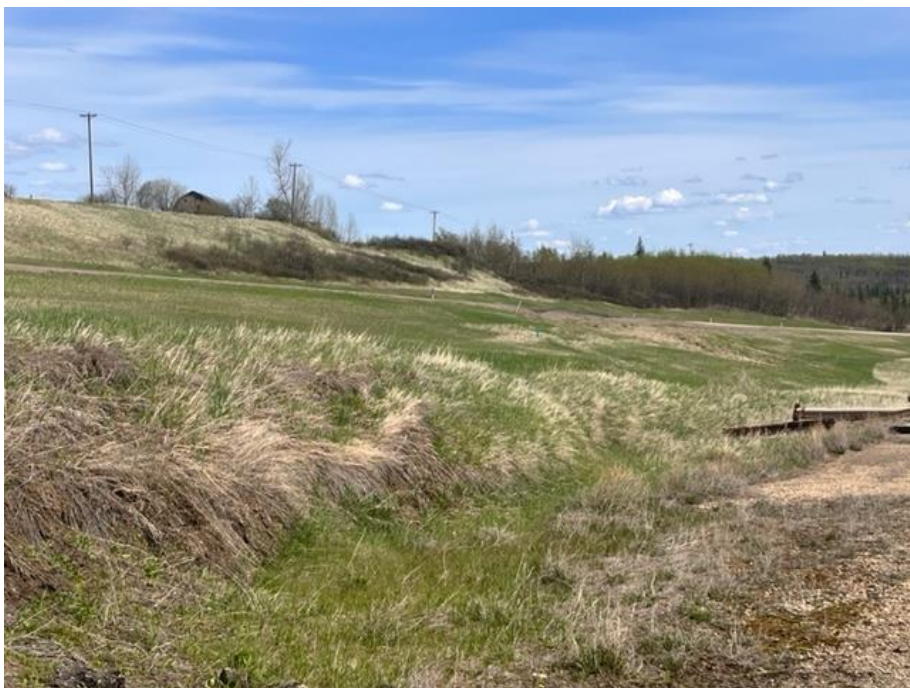
Photo 4. Looking northeast at southern slide scarp which crosses the old highway alignment.
