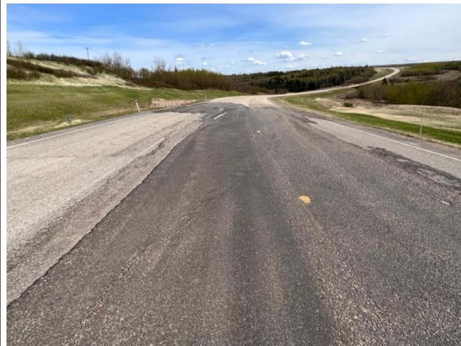
Photo 9. Looking east from near the middle of the 2021 ACP patch where crack continues into WBL.
