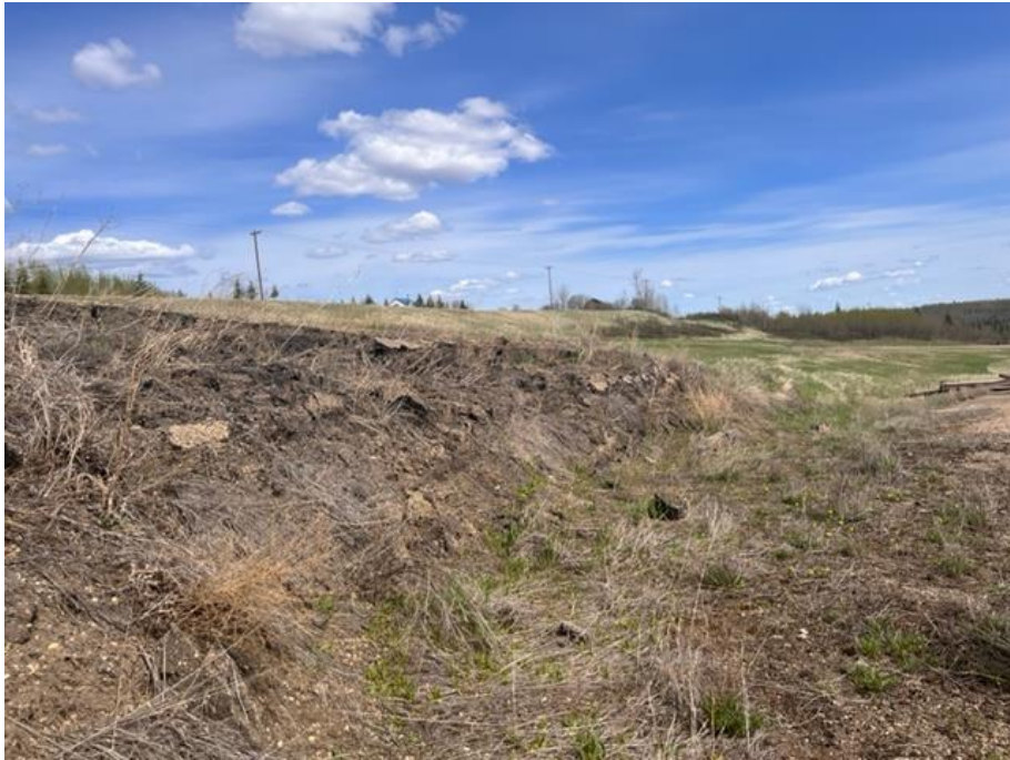
Photo 5. Looking southeast from old highway alignment at south slide scarp.
