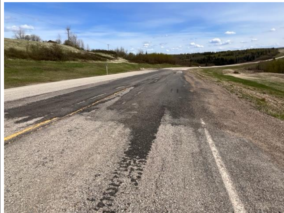
Photo 7. Looking east from the shoulder of the EBL of Hwy 49:06 at the dip in the 2021 ACP patch.
