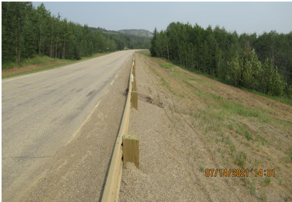
Photo 2 - Looking east at the guardrail at the west highway dip. Note the erosion rill in the embankment slope that formed from channelized runoff flowing along the dip in the highway.
