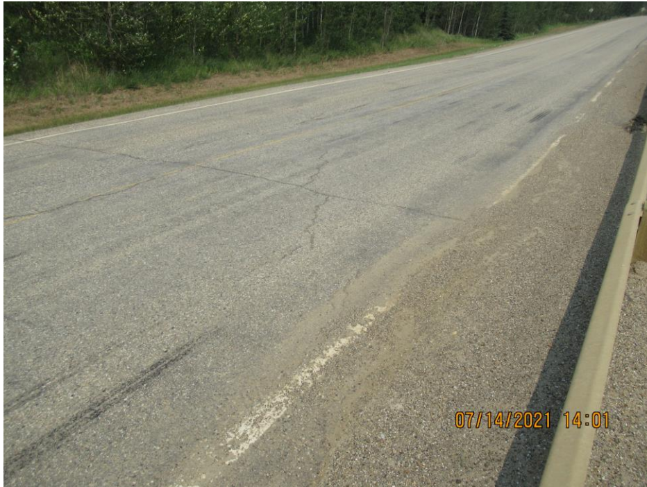
Photo 3 - Looking northeast along the scarp crack at the west end of the site. Note the highway dip to the east of the crack.
