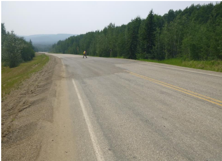
Photo 6 – Looking west at the fresh ACP patch placed over the east end of the site.
