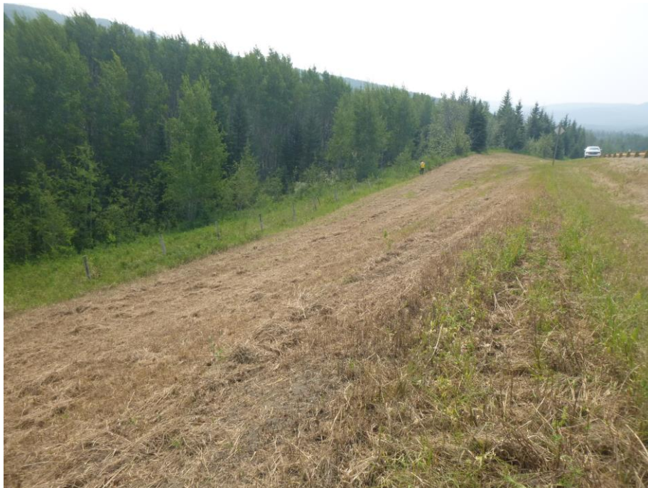
Photo 4 - Looking southwest at the dip/sunken south highway embankment located at the west end of the site below the hwy scarp crack area. There is also a bow in the fence.
