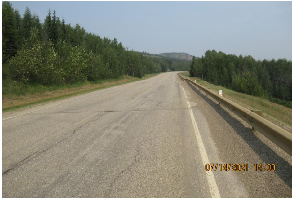
Photo 1 – Looking east along the cracked highway surface from the west end of the site. Note the west dip in the road/guardrail in the background.
