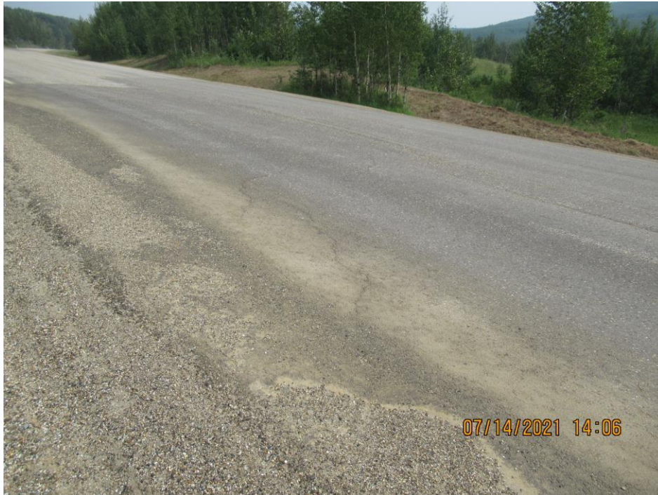
Photo 5 – Looking southeast across the east end of the site at the scarp crack reflecting through the fresh ACP patch.
