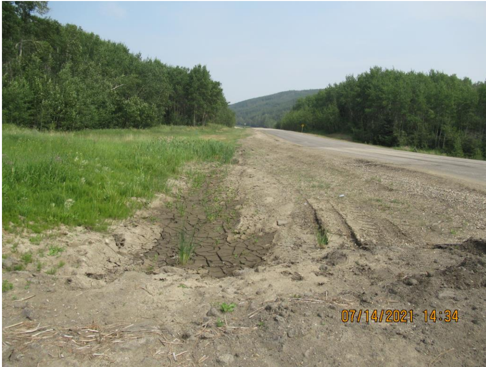
Photo 9 – Looking east along the north highway ditch at the dipped hwy and sagged cattail area (no ponded water this year).
