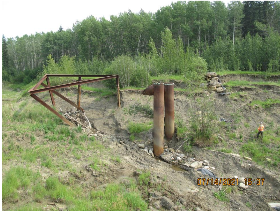
Photo 15 – Looking southeast at the tilted trash rack and twin pipe inlet risers in the eroded (and now partially silted in) channel.
