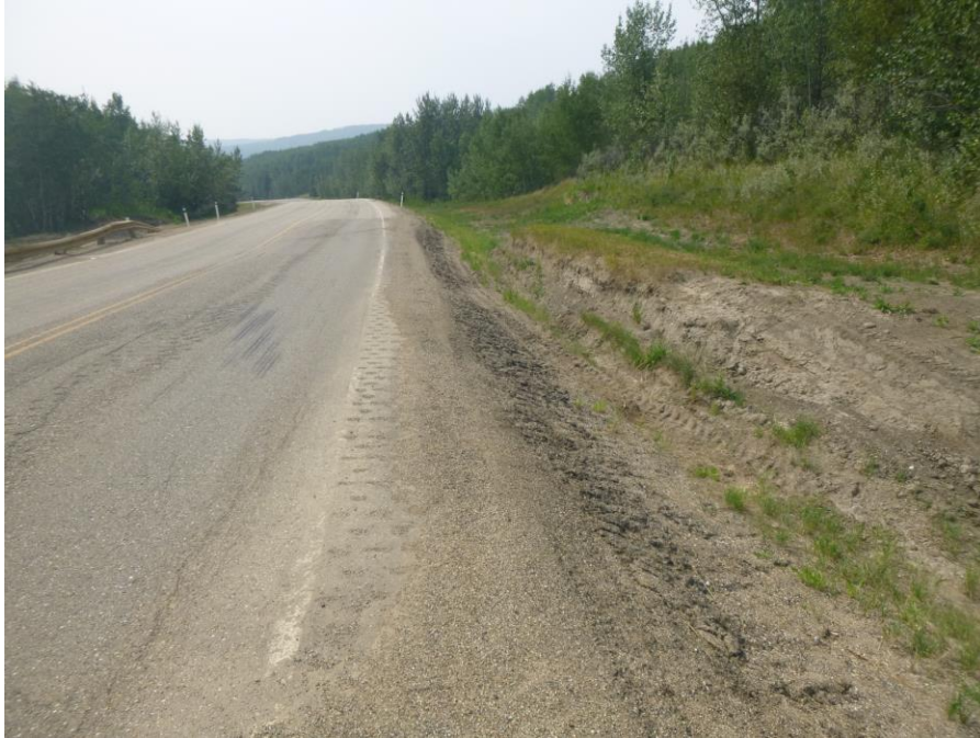
Photo 3 – Looking west from near the west end of the guardrails along the fresh scarp that extends along the north highway ditch.
