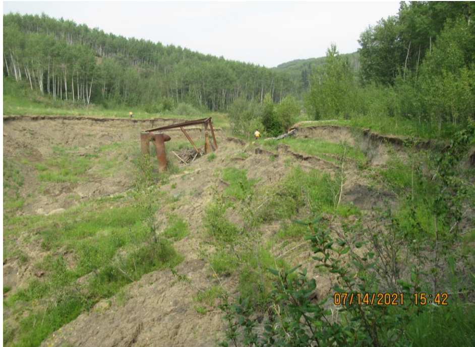
Photo 17 – Looking northeast at the trash rack and pipe inlets in the eroded channel. Note the enlarged south bank perimeter slumping.
