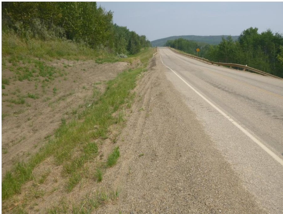
Photo 2 – Looking east along the recent WB lane patch over the highway cracks and large dip that extends across the highway near the west end of the site.
