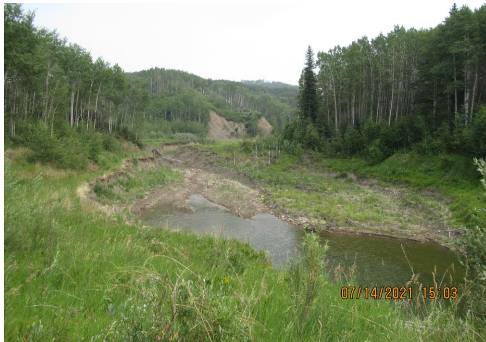
Photo 14 - Looking east at the upstream end of the eroded and silted in channel.
