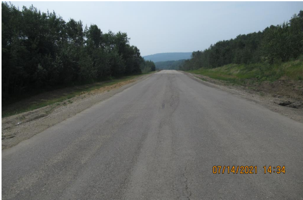
Photo 8 – Looking west at the west milled/patched area over the east slide crack.
