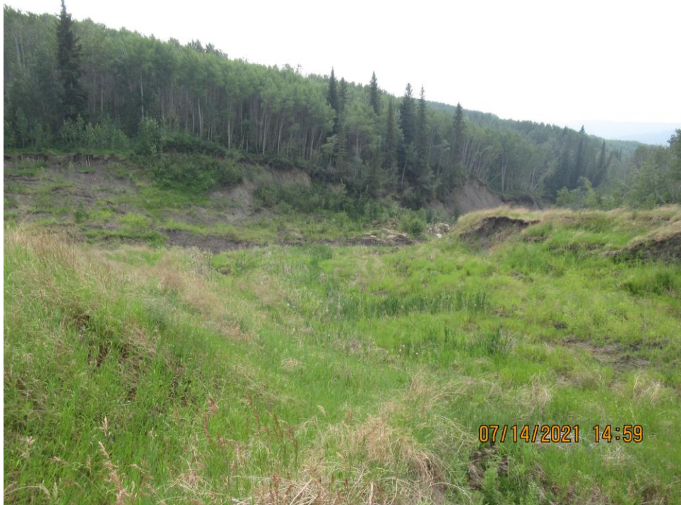
Photo 13 – Looking southwest at the eroded tributary channel from the north side of the eroded piping area. Significant seepage was emanating from the drains in the base.
