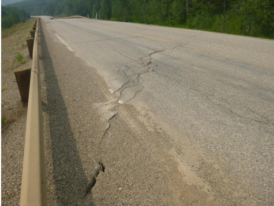
Photo 7 – Looking northwest across the highway at last years unrepaired slide cracks east of the northeast guardrail end.
