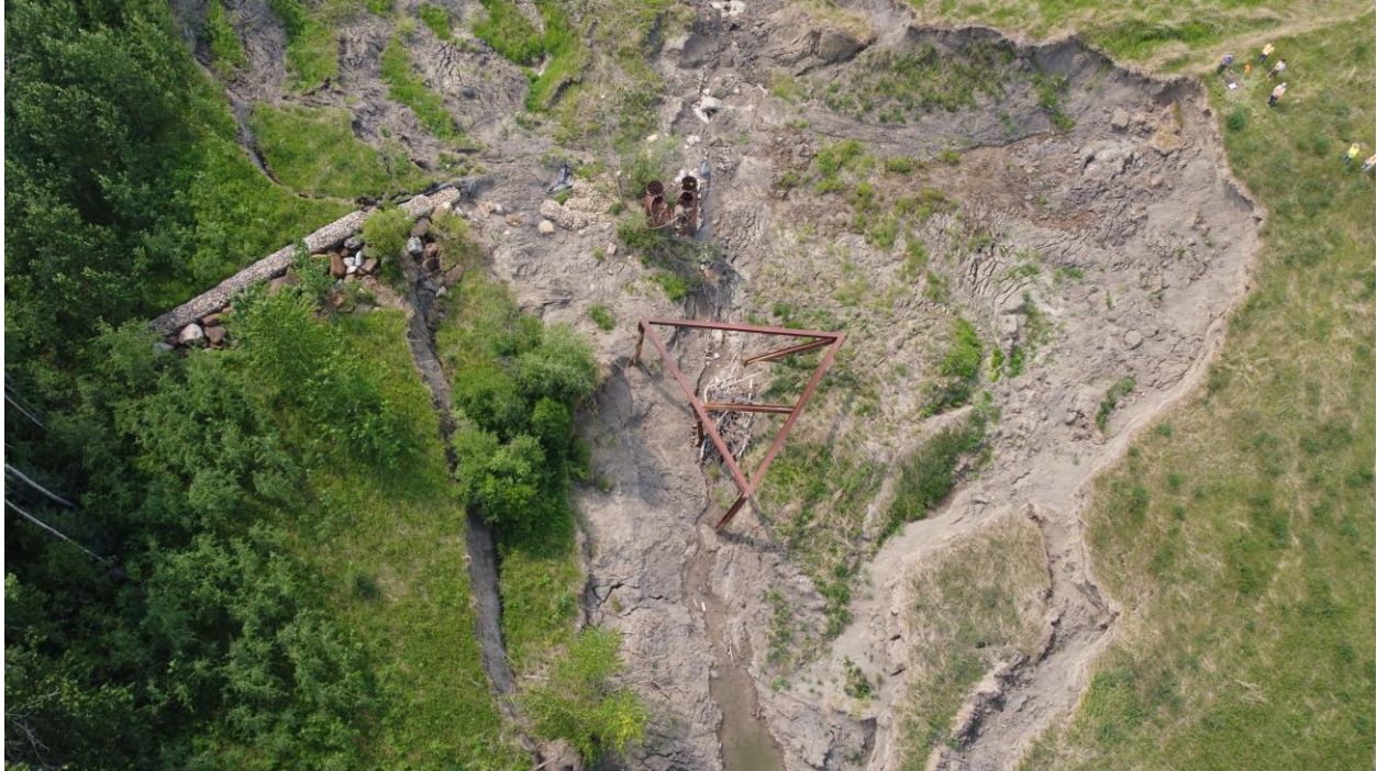
Photo 21 – UAV view looking west overtop the trash rack and twin pipe riser inlets in the eroded channel.
