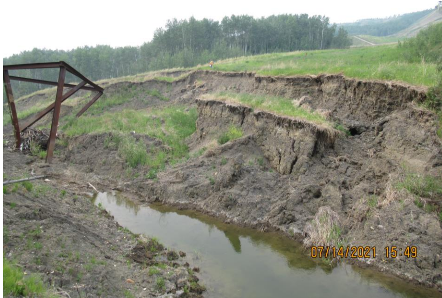
Photo 19 – Looking northwest at the extensive and continued slumping/erosion along the north channel banks adjacent to the trash rack.
