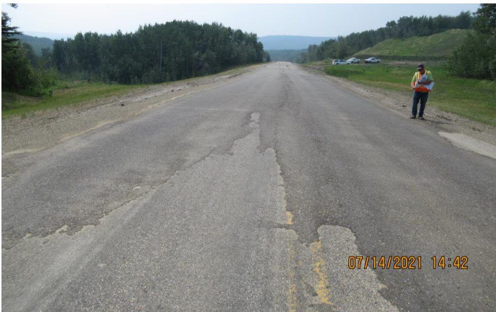
Photo 10 – Looking west along the highway at the east milled/patch over the east scarp cracked area at the east end of the site.
