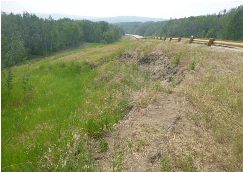
Photo 6 – Looking west at Embankment Slump A on the south side of the hwy.
