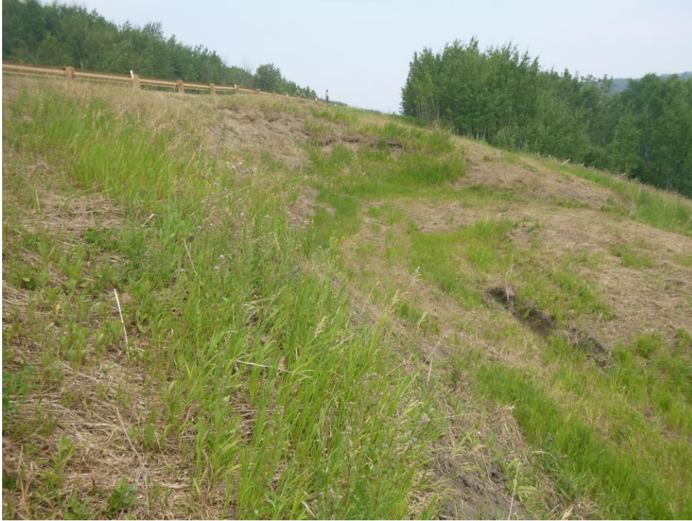
Photo 5 – Looking east along the south highway Embankment Slump B.
