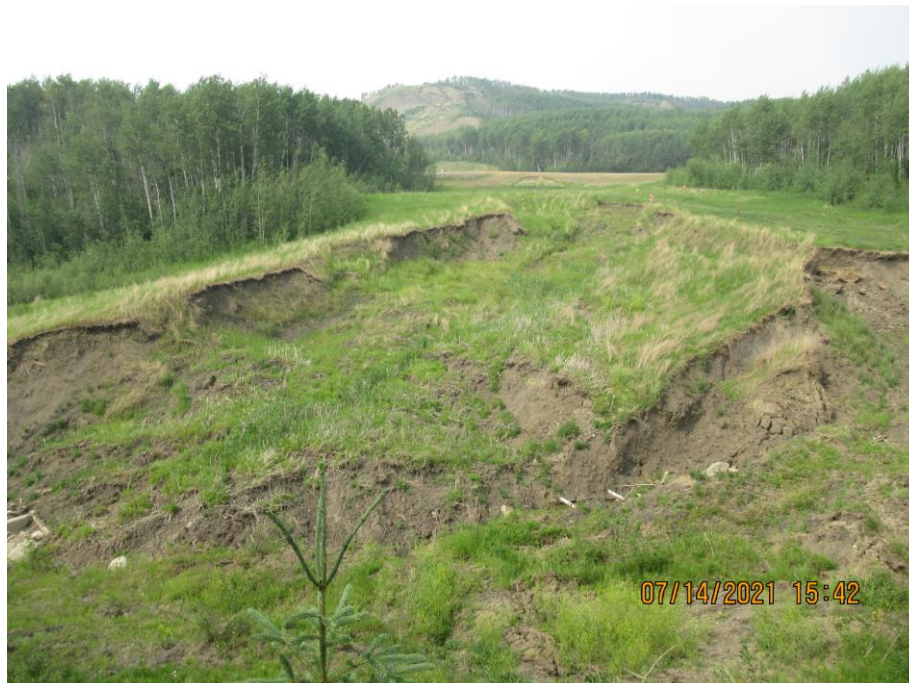
Photo 16 – Looking north at the piping erosion area shown in Photo 13, on the north edge of the channel.
