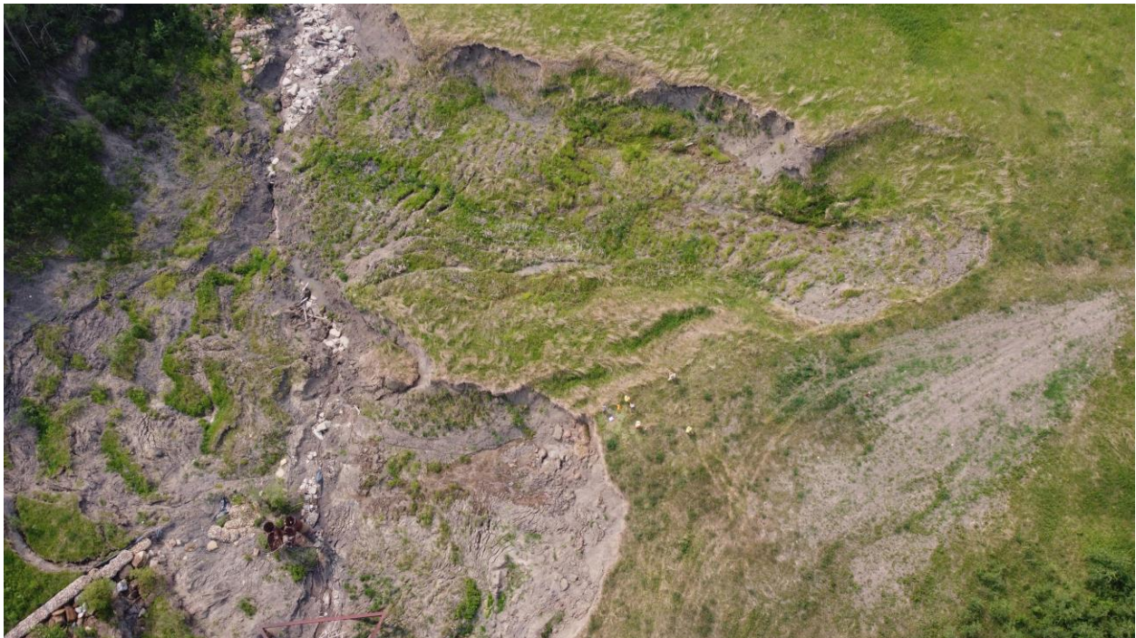
Photo 22 – UAV view looking west at the piping erosion area on the north edge of the eroded channel.
