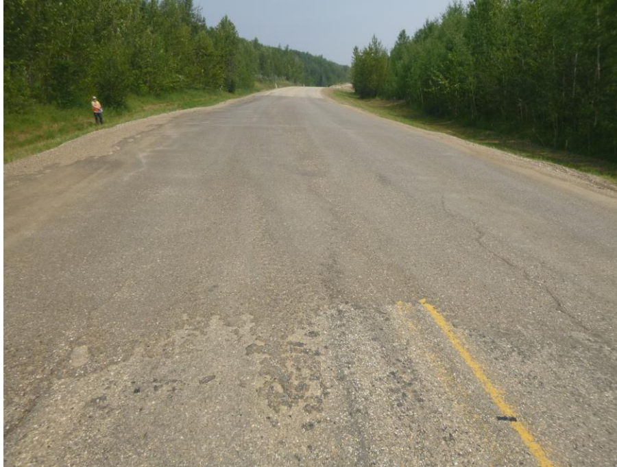
Photo 1 - Looking east along the highway at the milled/patched area over the two cracks first observed in 2013 that mark the west boundary of the slide on the highway.
