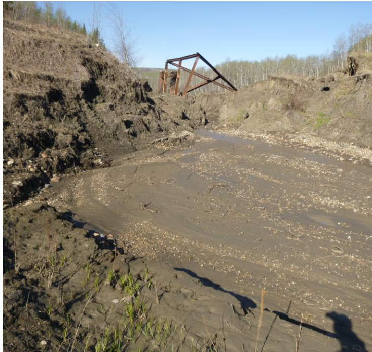
Photo 13 - Looking west at the eroded tributary channel from east of the eroded piping area. Note the fresh silt deposition in the foreground.
