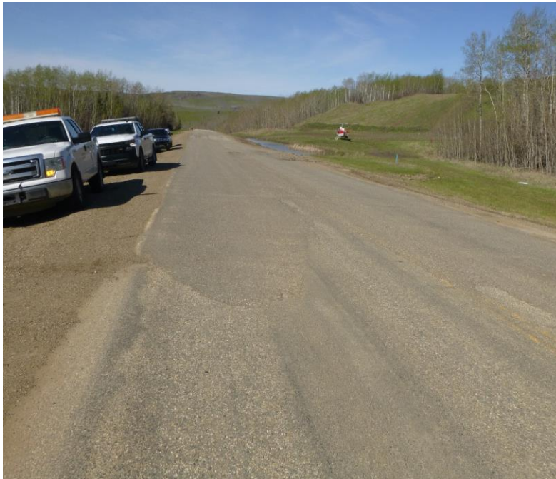
Photo 10 - Looking west along the highway at the east milled/patch over the east scarp cracked area at the east end of the site.
