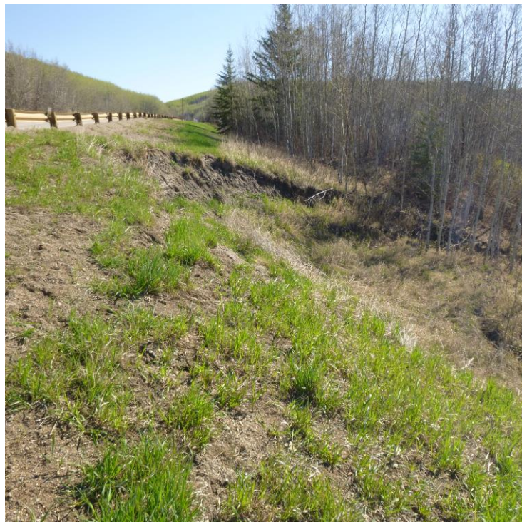
Photo 6 – Looking east at Embankment Slump A on the south side of the hwy.
