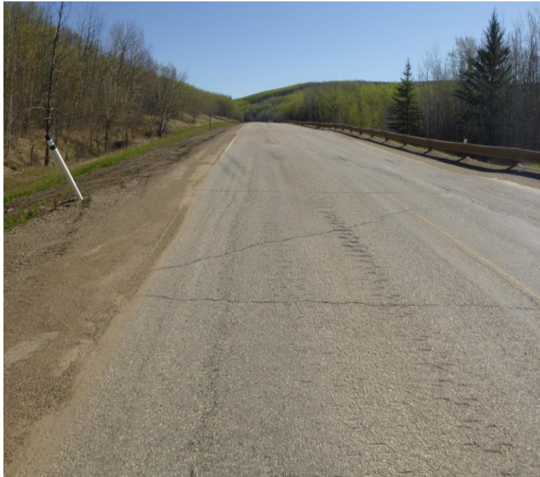
Photo 7 – Looking east along the highway at last years unrepaired slide cracks east of the northeast guardrail end.
