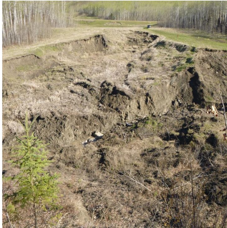
Photo 11 – Looking north towards the highway at the piping erosion area. Note the south hwy embankment slump below the east hwy scarp cracked area.
