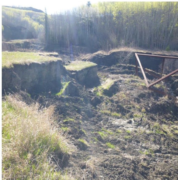
Photo 14 – Looking southeast along the eroded channel where it meets the eroded piping area, with the trash rack on the RHS.
