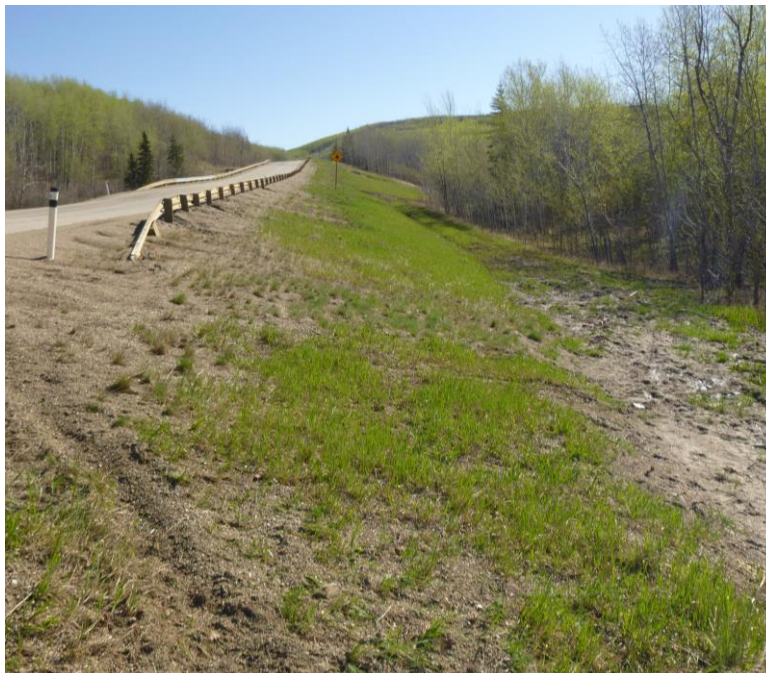
Photo 4 – Looking east along the south side of the highway at an active seepage area below the west end of the south guardrail.
