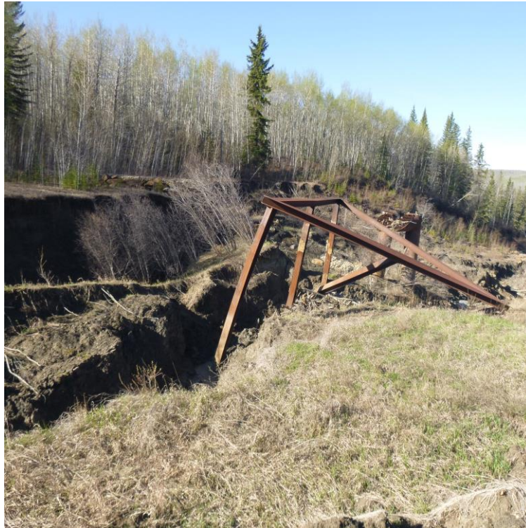
Photo 15 – Looking west at the twin pipe inlet risers, and the eroded trash rack.
