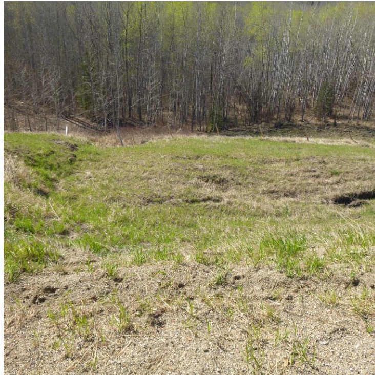
Photo 5 – Looking south along the south highway Embankment Slump B.
