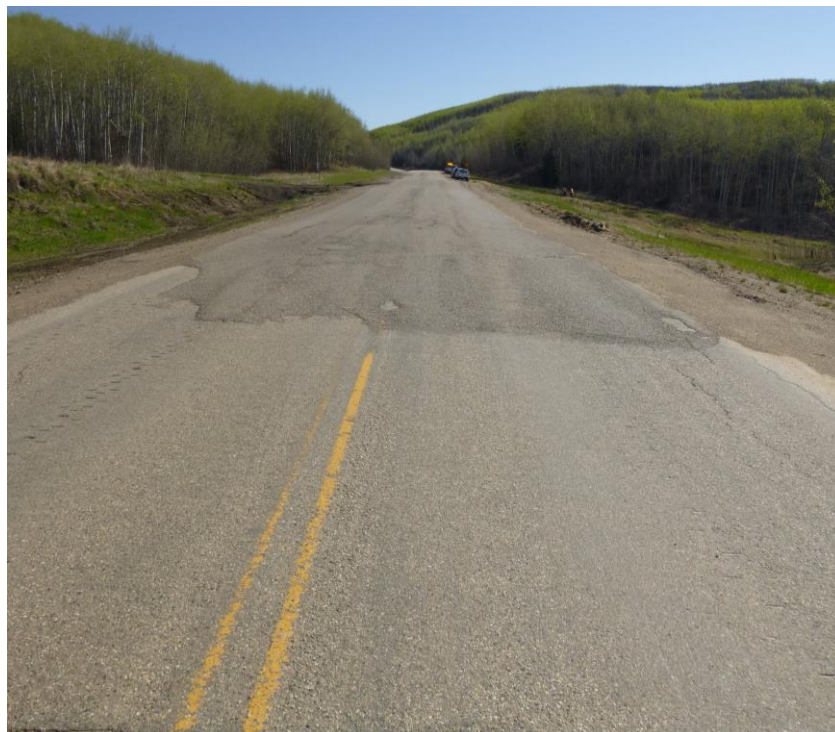
Photo 8 – Looking east at the west milled/patched area over the east slide crack.
