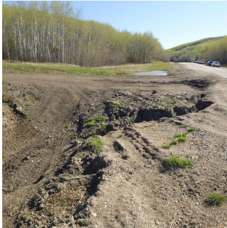
Photo 9 – Looking east along the north highway ditch at the erosion gully across the access, the dipped hwy, and sagged area with ponded water.
