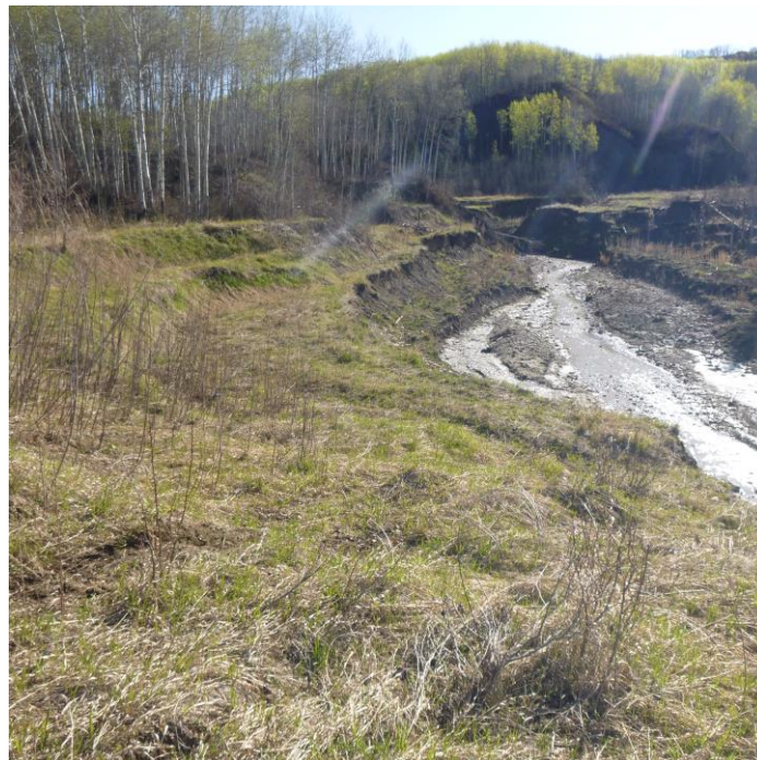
Photo 12 – Looking east at the upstream end of the eroded and silted in channel.
