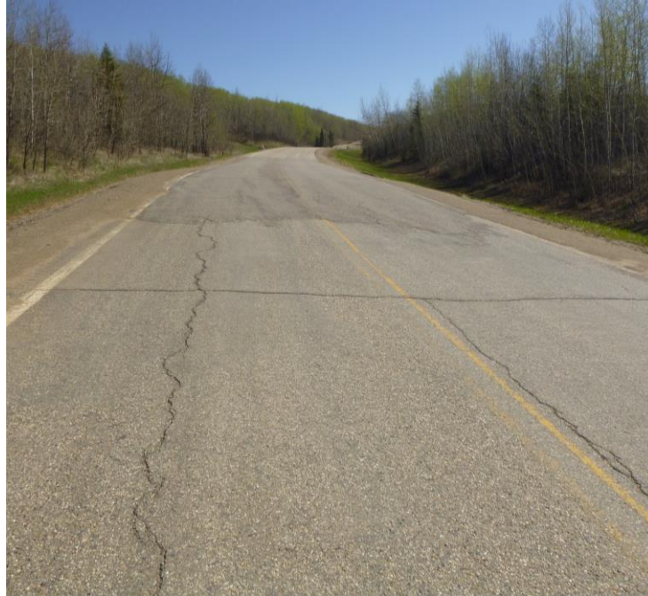
Photo 1 - Looking east along the highway at the milled/patched area over the two cracks first observed in 2013 that mark the west boundary of the slide on the highway.
