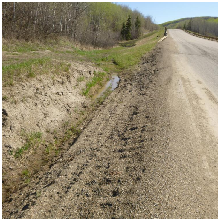
Photo 2 – Looking east along the slide scarp in the south ditch, and large dip that extends across the highway near the west end of the site.
