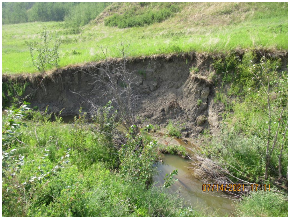
Photo 18 – Looking east (upstream) along the north ditch channel at the ongoing erosion and eroded gabion liner between the 760 SWSP and 810 CSP outlets.
