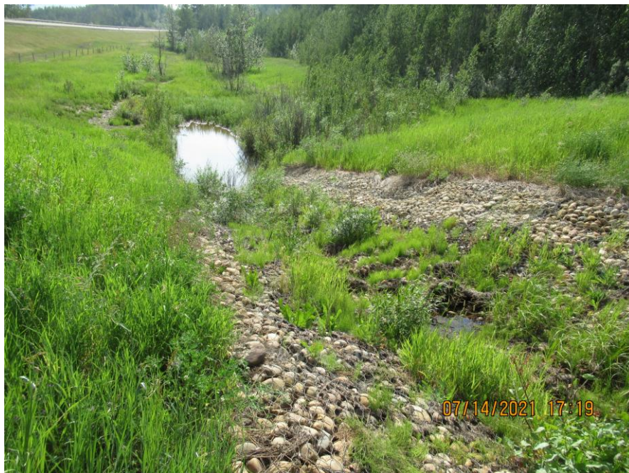
Photo 16 - Looking west (downstream) along the north ditch channel just upstream of the 810 CSP outlet and 1040 SWSP inlet. Note the gabions are still intact here.
