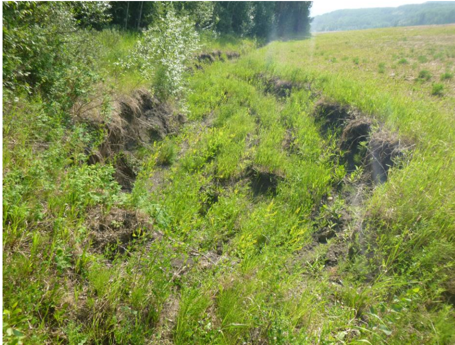
Photo 9 – Looking northwest at the erosion that formed in 2020 along the boundary of the south embankment fill and the bush line.
