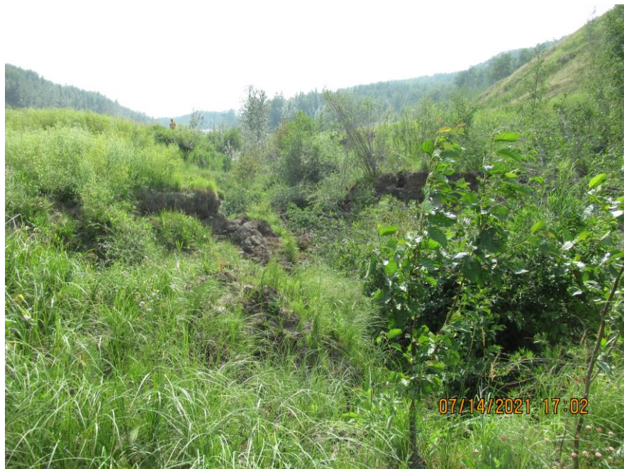
Photo 20 - Looking west at the erosion in the north ditch channel at the completely eroded gabion liner east (upslope) of the 760 SWSP outlet.
