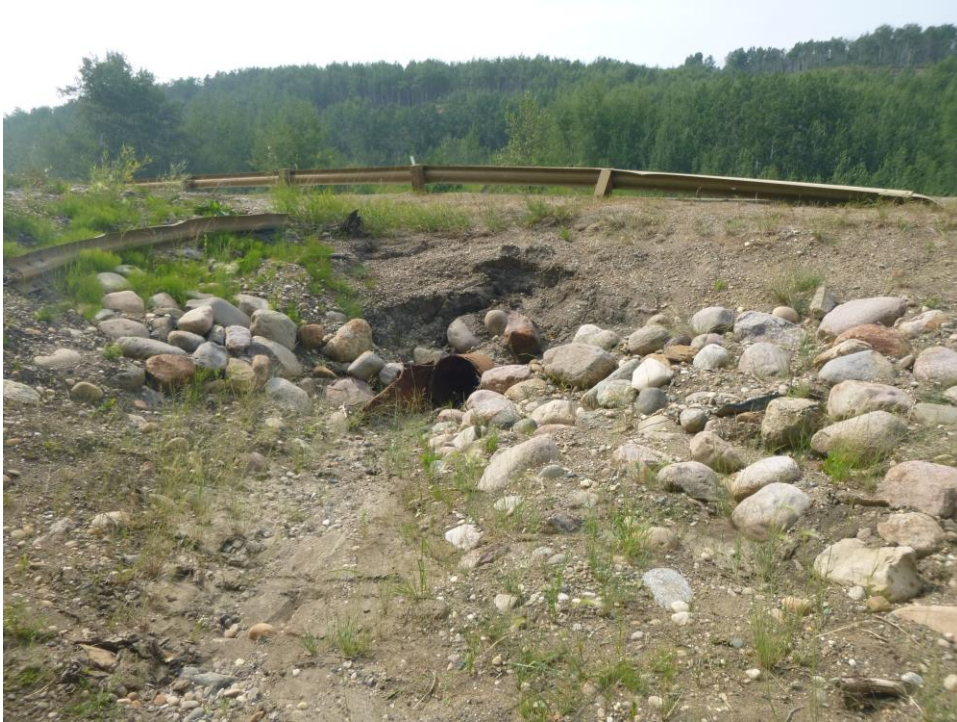
Photo 1 – Looking north at the inlet of the 810 CSP on the south side of the hwy embankment.
