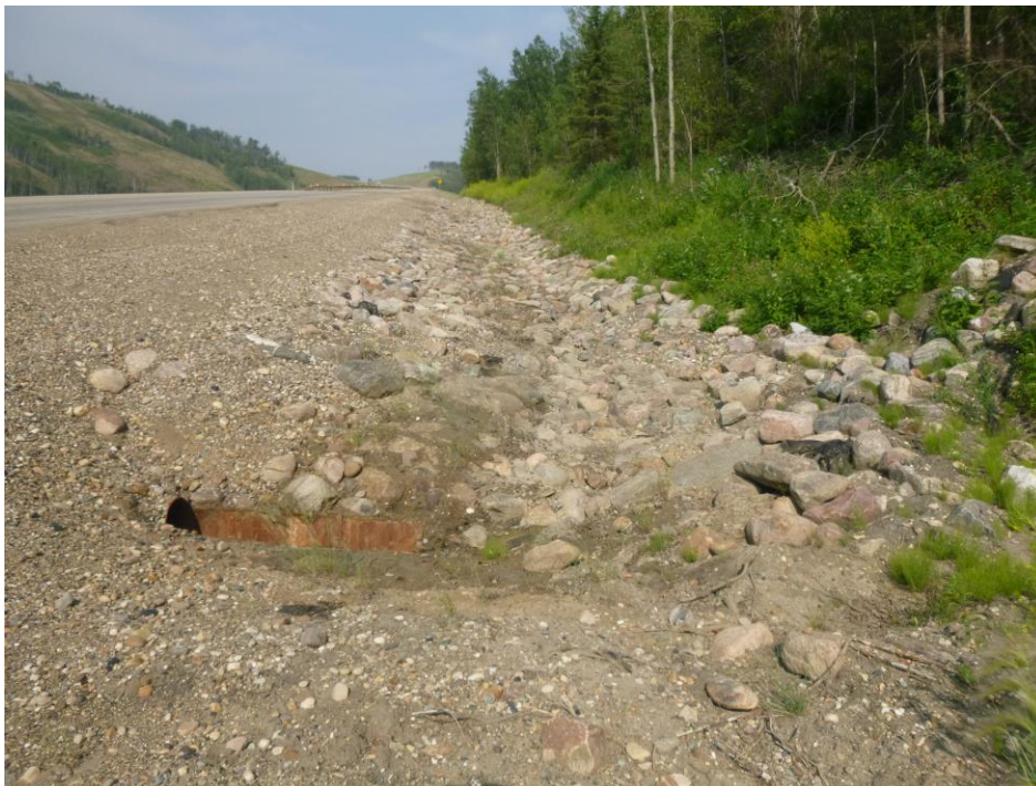
Photo 6 – Looking east from the ditch block along the riprapped south ditch channel from the inlet of the 760 mm dia. SWSP.
