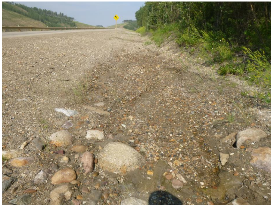
Photo 8 – Looking east along the south ditch channel and hwy embankment that was lined with 6-80 gravel.
