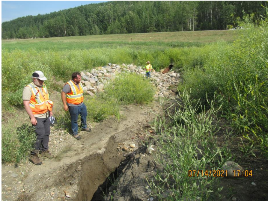
Photo 19 - Looking south at the 760 mm SWSP outlet. Note the erosion gully along the west side of the riprap that was added downslope of the culvert in 2020.
