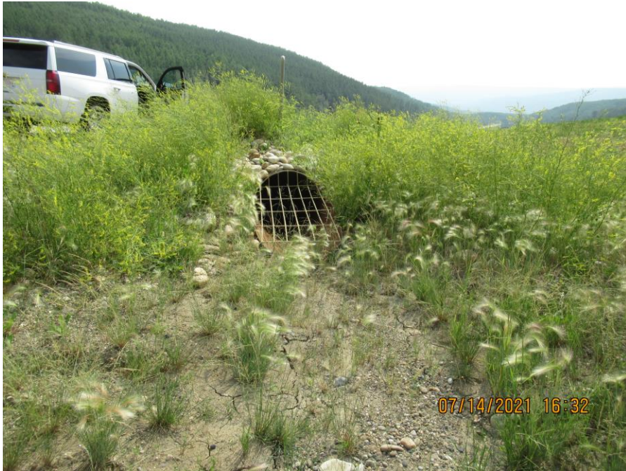
Photo 13 – Looking west at the repaired erosion area around the north 900 mm SWSP entrance.
