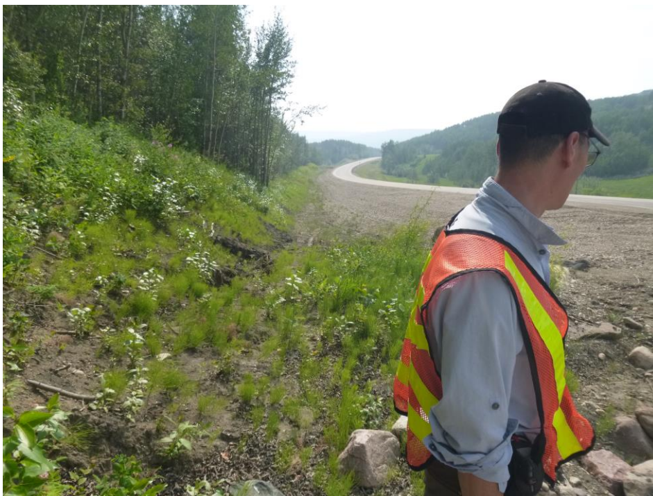
Photo 4 – Looking west along the unlined south highway ditch from the inlet of the 760 mm dia. SWSP.
