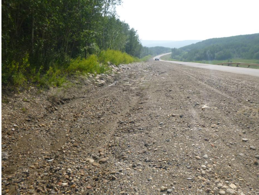
Photo 7 - Looking west along the recently lined south ditch channel and highway embankment, at the point where the riprap (west) and gravel (east) merge.
