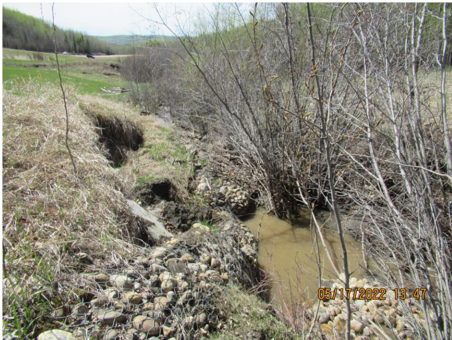
Photo 20 - Looking east at the erosion in the north ditch channel at the completely eroded gabion liner between the 760 SWSP and 1200 CSP outlets.
