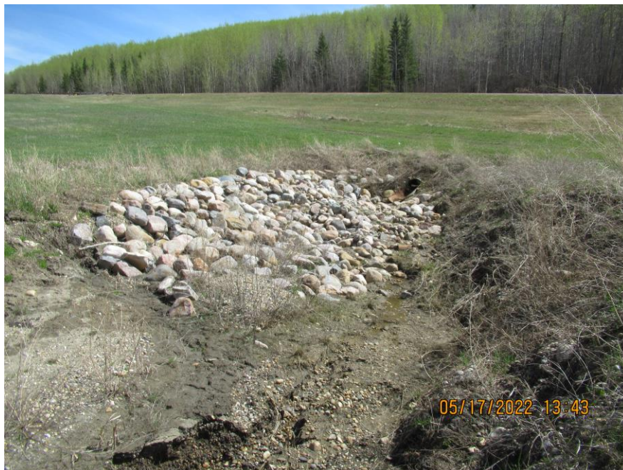
Photo 18 - Looking south at the 760 mm SWSP outlet. Note the erosion gully along the west side of the riprap that was added downslope of the culvert in 2020.
