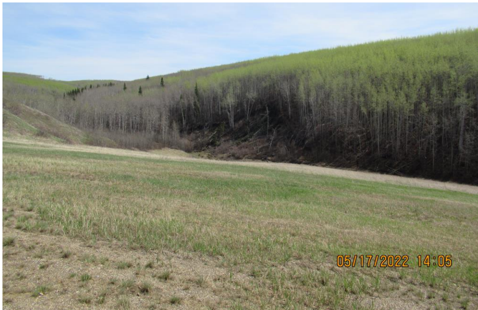
Photo 12 – Looking south at the valley slope slumping above the 1200 culvert inlet and gabion outlet area, caused by rapid drawdown of built-up floodwater.
