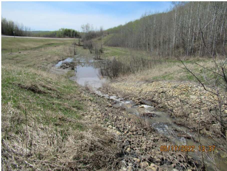
Photo 16 - Looking west (downstream) along the north ditch channel upstream of the 810 CSP outlet. Note the gabions are still intact here.
