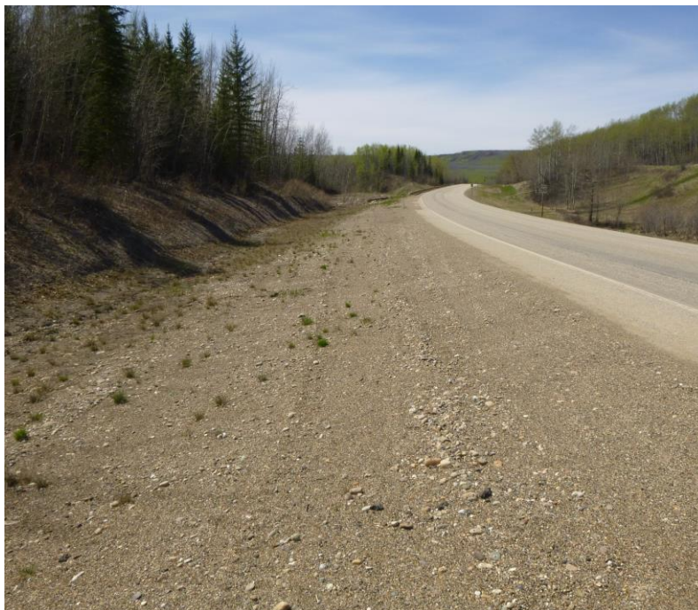
Photo 4 – Looking west along the unlined south ditch from near the west end, at the 2020 grading that took place along the south highway embankment and ditch.
