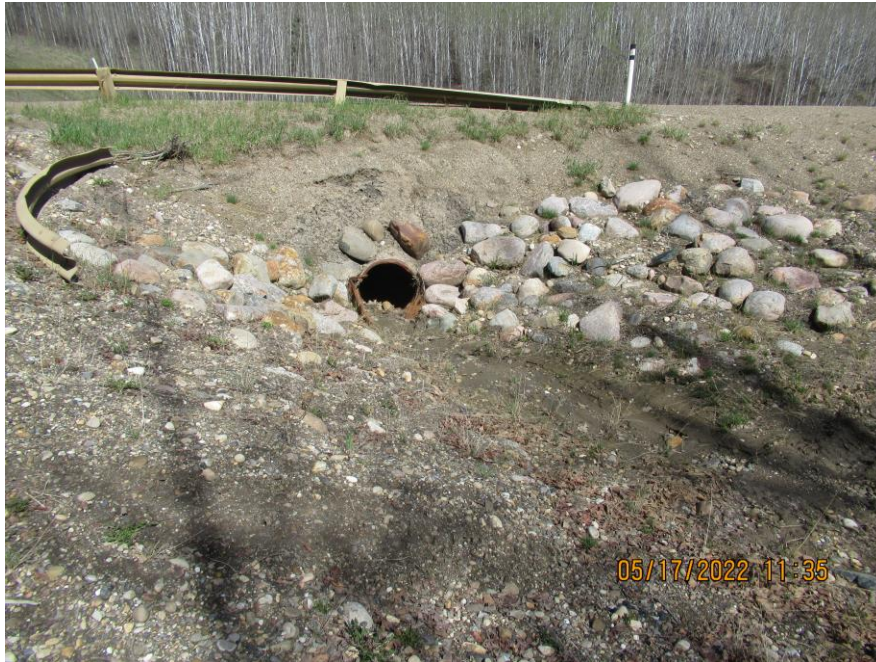
Photo 3 – Looking north at the inlet of the 810 CSP on the south side of the hwy embankment.
