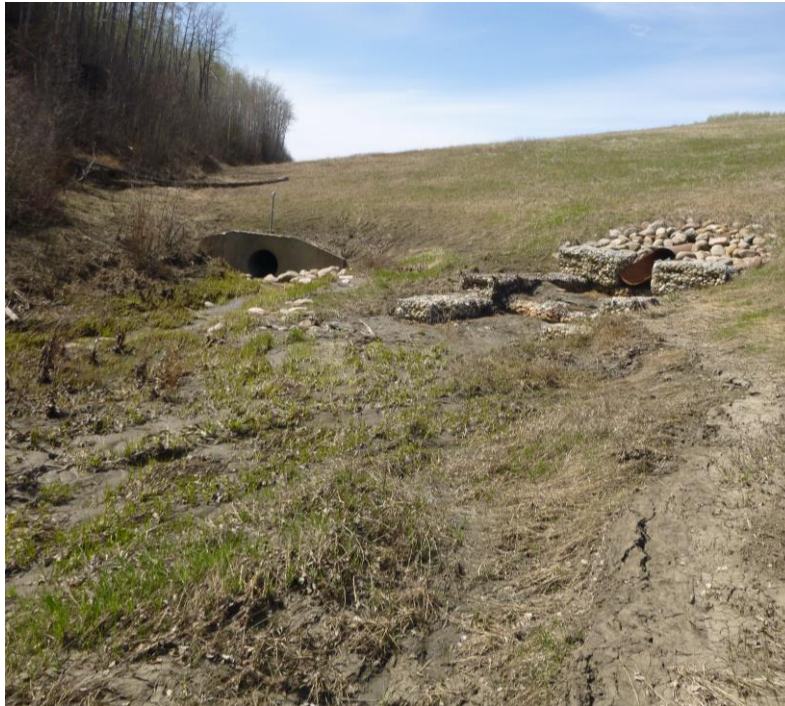
Photo 11 - Looking northwest at the 1200 CSP inlet headwall (left), and the 900 SWSP outlet and gabion outlet structure (right).
