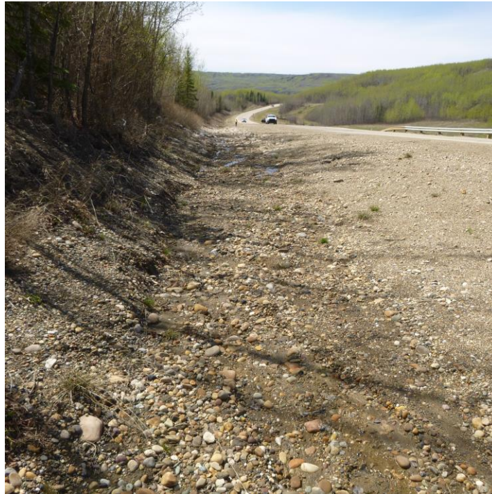
Photo 9 – Looking west along the south ditch channel and hwy embankment that was lined with 6-80 gravel.
