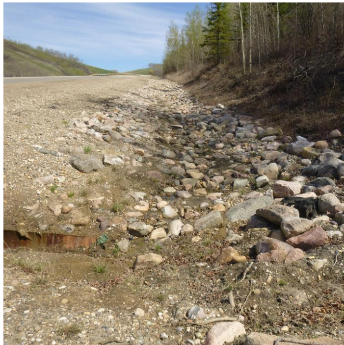
Photo 8 – Looking east from the ditch block along the riprapped south ditch channel from the inlet of the 760 mm dia. SWSP.
