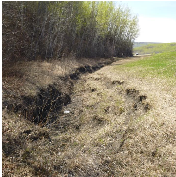
Photo 10 – Looking west at the erosion that formed in 2020 along the boundary of the south embankment fill and the bush line.
