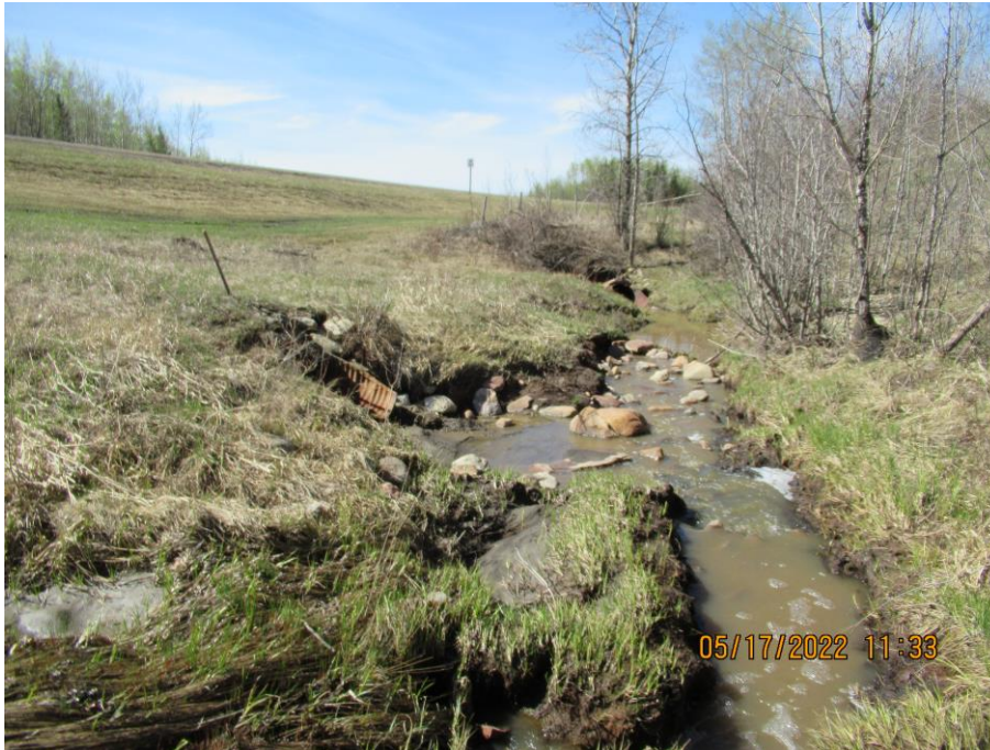
Photo 15 - Looking southwest at the 810 CSP outlet (left), and the 1040 SWSP inlet (right), at the west end of the north ditch channel.
