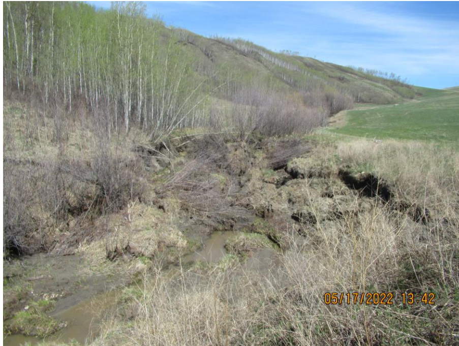
Photo 17 – Looking east (upstream) along the north ditch channel at the ongoing erosion and eroded gabion liner just downstream of the 760 SWSP outlet.
