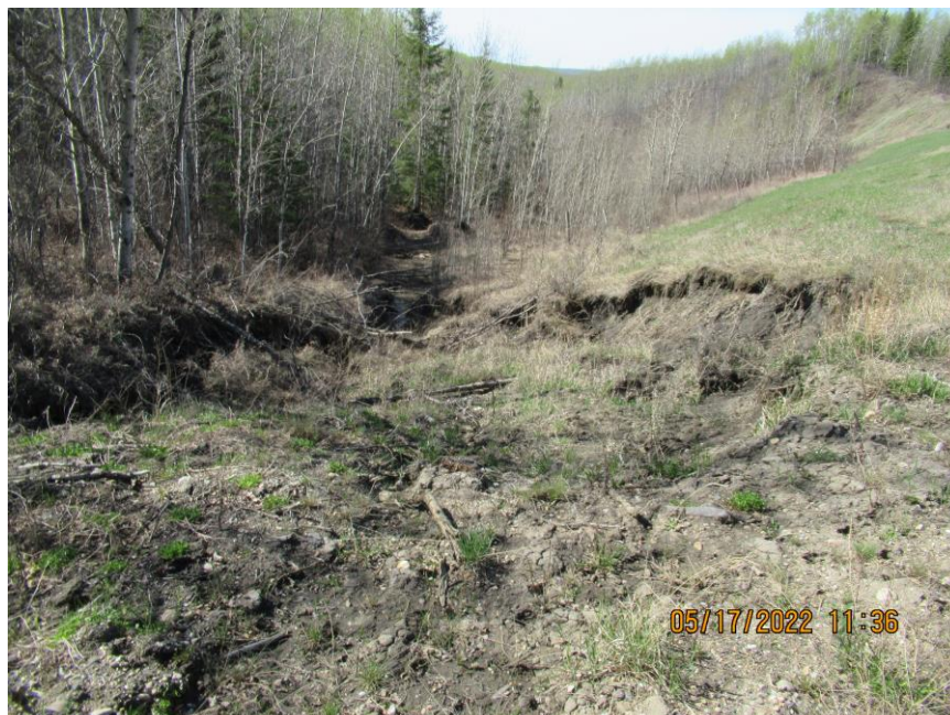
Photo 2 – Looking south along the eroded bush channel at the west end of the site.
