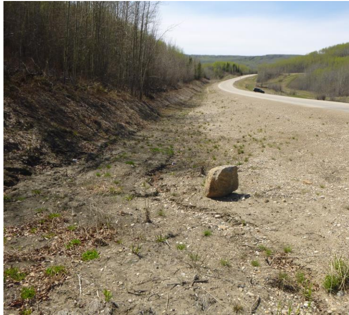
Photo 7 - Looking west along the unlined south highway ditch from the inlet of the 760 mm dia. SWSP.
