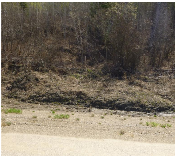
Photo 6 – Looking at a 12m wide x 3m high toe slump into the south edge of the south ditch.
