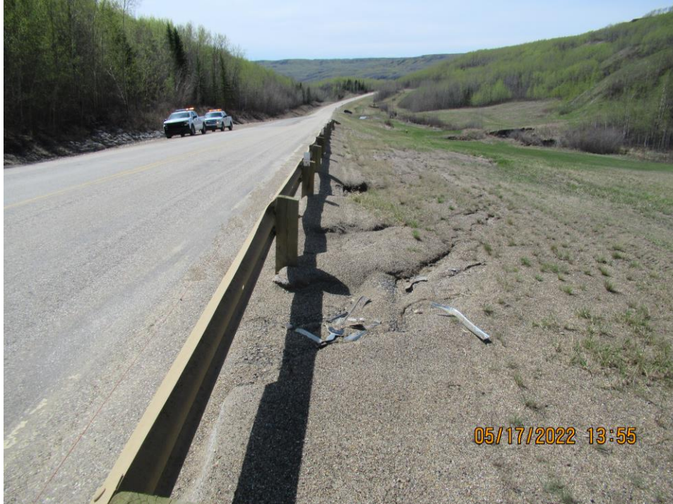
Photo 14 – Looking west at the rilling adjacent to the north guardrail (just west of the repaired rilling on the north embankment).
