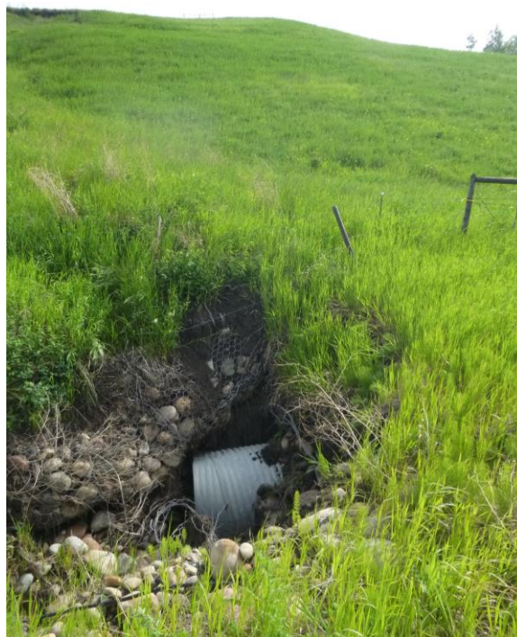
Photo 12 – Looking north at the damaged gabions squeezing in around the culvert inlet caused by slide movement from above (~STA 2+740).
