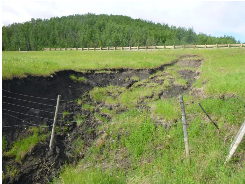
Photo 16 – Looking south along the erosion gully formed downstream of the cross-culvert outlet. The headscarp of this erosion has encroached to 6.2m from the white line.
