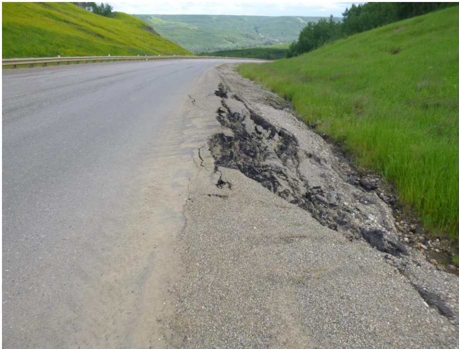
Photo 8 – Looking east along the highway from ~STA 2+900 at the area of the 20 m long slump in the edge of the eastbound driving lane pavement and a crack along the center of the EB driving lane pavement spanning beyond this slump.
