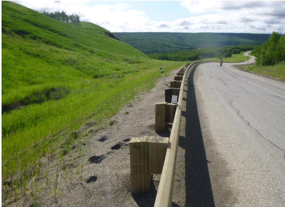
Photo 11 – Looking east along the cracked pavement and soft north shoulder and embankment (~STA 2+880). Note the slide debris that has pushed into the north ditch.
