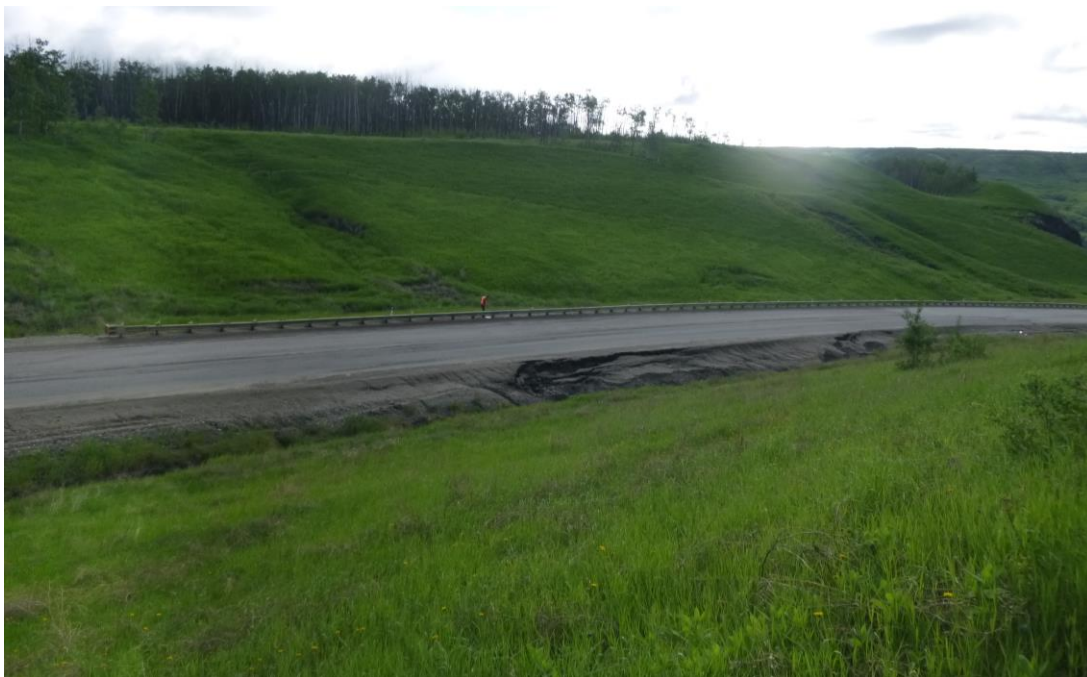
Photo 2 – Looking northeast at the east end of the north backslope erosion and slumps. Also note the south highway embankment slumping and ditch erosion formed from concentrated surface runoff.
