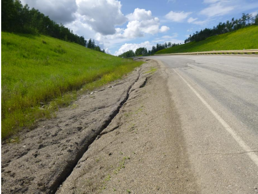
Photo 9 - Looking west along the soft south highway embankment and ditch at ~STA 2+790, showing the patched EB lane and the south embankment slumps in the background.
