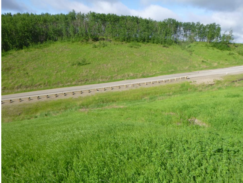
Photo 3 – Looking south at the slumping in the west end of the south highway cut backslope. Note the north guardrail, shoulder pitrun, and ditch grading that took place in 2017.
