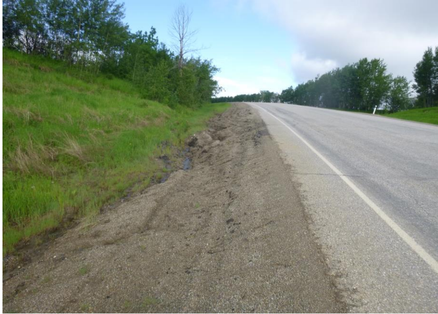
Photo 5 – Looking west along the south ditch from ~STA 3+020. Note the wet, soft, rilled shoulder and slumping highway embankment adjacent to the ditch which was graded in 2017. The tall dead tree beside the south ditch marks the start of the proposed repair (~STA 3+060).
