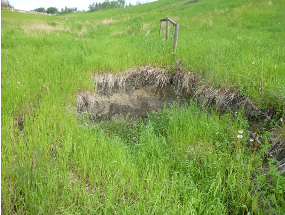
Photo 13 – Looking west along the north ditch at the 3m x 5m x 2.8m deep sinkhole overtop the culvert a short distance east of the inlet (~STA 2+730).
