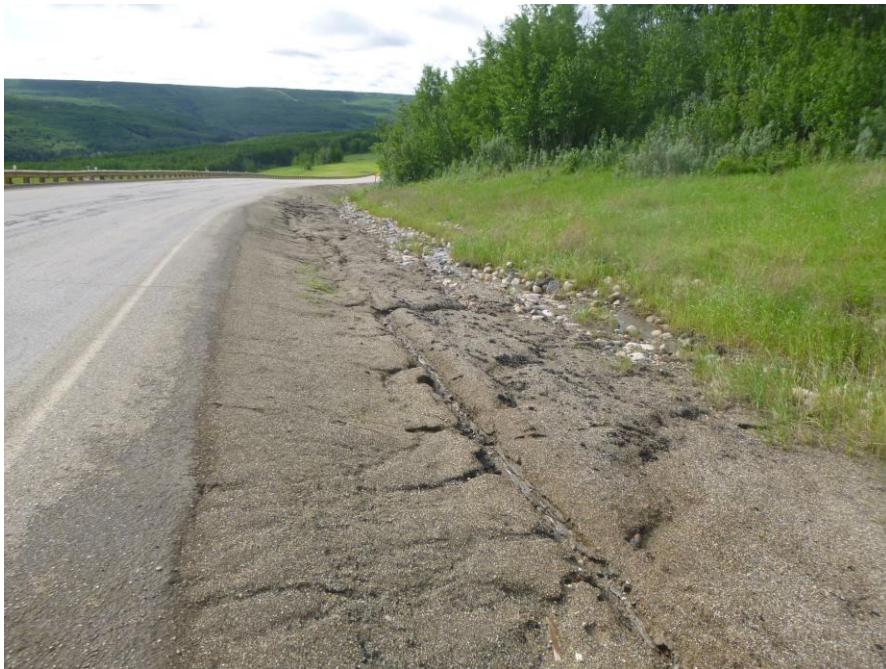
Photo 10 – Looking east at the riprap lined portion of south ditch, and the soft, distorted shoulder/highway embankment above it (~STA 2+790).
