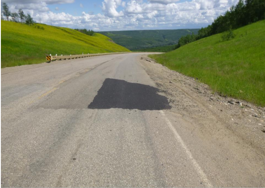
Photo 7 – Looking east along the south edge of the highway at the west end of the patched, cracked and slumping south highway surface and embankment (~STA 2+930).
