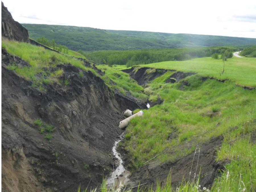
Photo 14 - Looking east along the large erosion ravine and fence line from the north ditch culvert outlet. Note the slide blocks that have slid down and broken off pieces of culvert.
