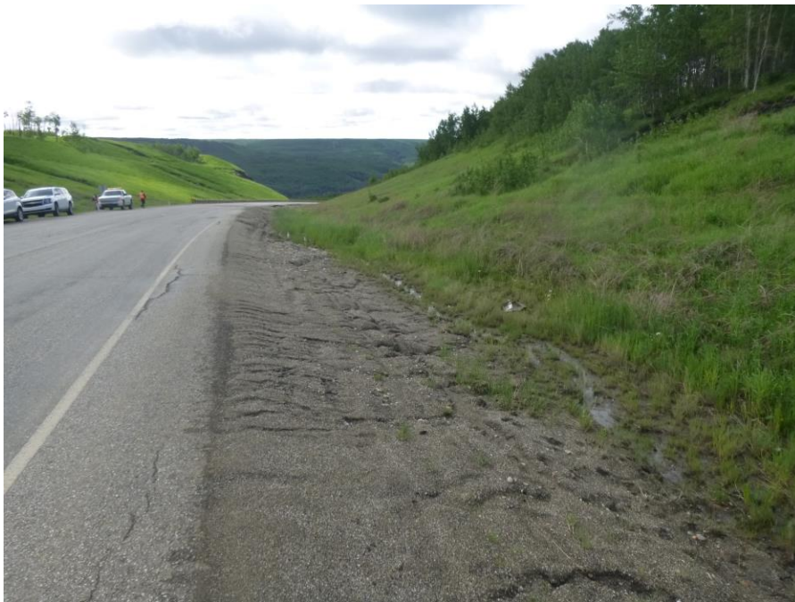
Photo 6 – Looking east along the south soft embankment and ditch from ~STA 2+980. The georidge ditch barriers installed as part of 2008 repairs are now gone.
