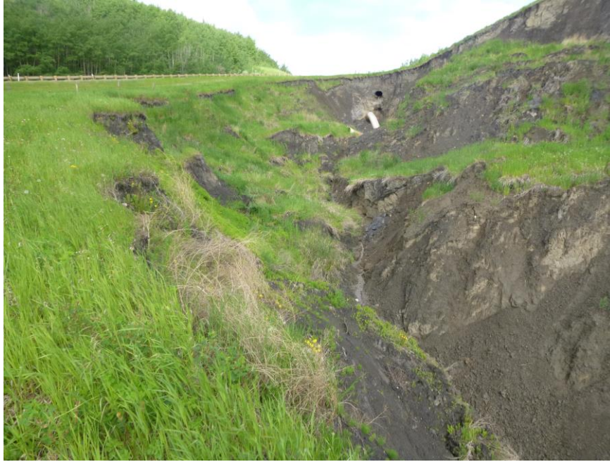
Photo 15 - Looking west parallel to the highway at the 7 m deep erosion ravine headscarp caused by runoff from the north ditch culvert outlet. The erosion/slumping has again encroached closer to the pavement white line.
