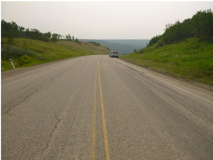
Photo 2 – Looking east along the center of the hwy from ~STA 3+060. The north half of the hwy (WB lane) was deemed to not require repairs at this location. Note the rutted outside wheel path in the EB lane.
