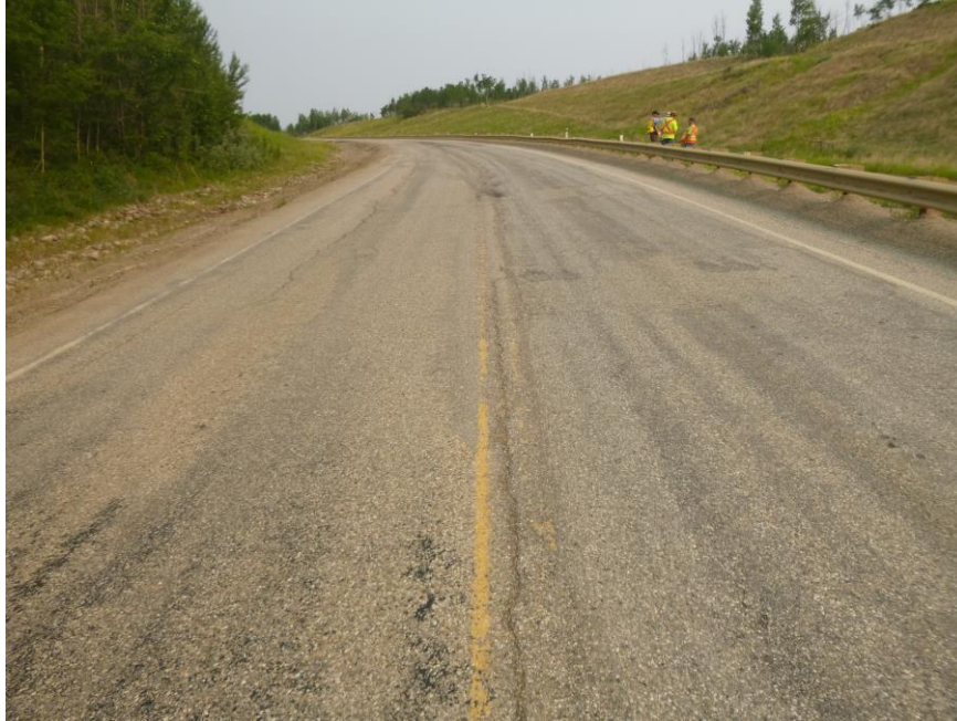
Photo 7 – Looking west along the cracked and deformed pavement from the east end of the proposed repair area (~STA 2+670, ~ 20 m west of the yellow curve sign). Note this area was also previously patched.
