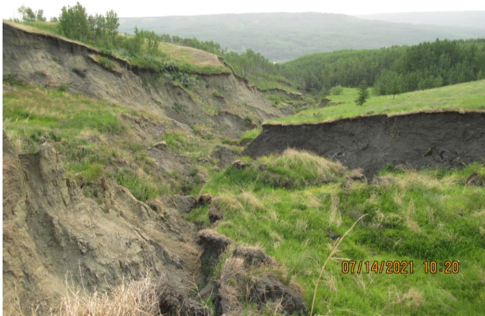
Photo 10 – Looking northeast along the large erosion ravine where the cross-culvert outlet erosion merges into it.
