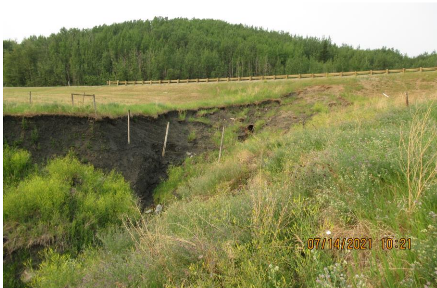
Photo 12 – Looking southeast at the erosion gully formed downstream of the cross-culvert outlet. The headscarp of this erosion has encroached to 5.3 m from the white line (from 6.2 m last year).
