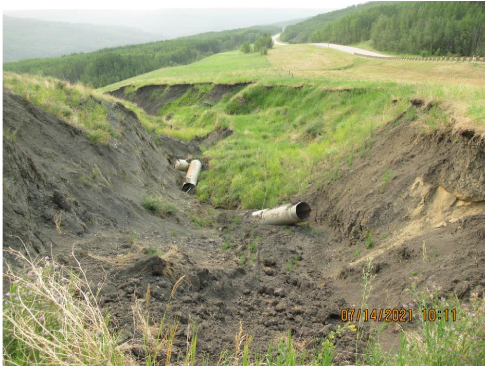
Photo 9 - Looking east along the large erosion ravine and fence line from the north ditch culvert outlet. Note the slide blocks that have slid down and broken off pieces of culvert.
