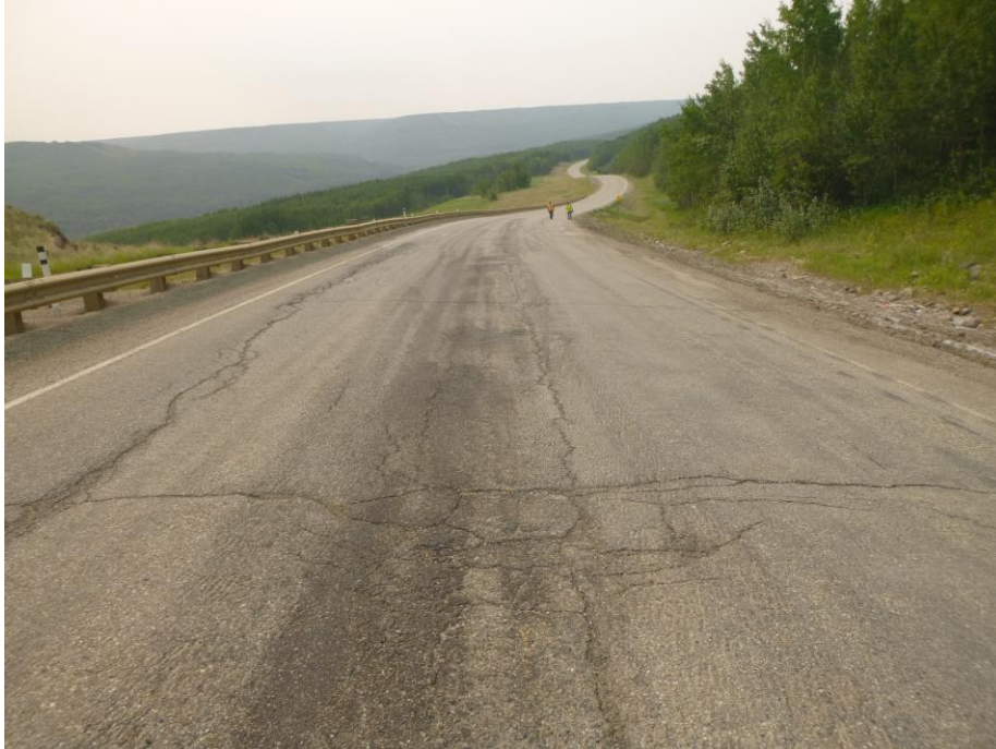
Photo 5 - Looking east along the center of the highway at ~STA 2+760, showing the cracking and rutting occurring in this previously patched area.
