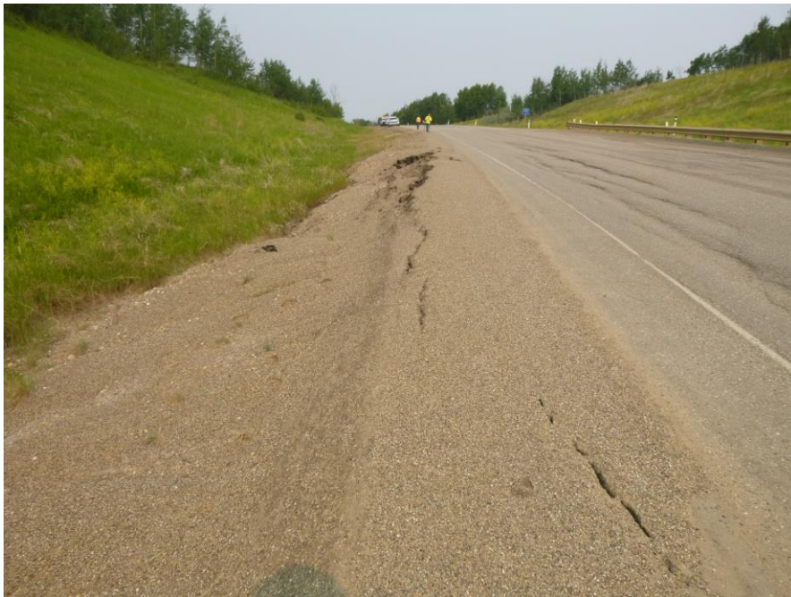
Photo 4 – Looking west along the south edge of the highway from ~STA 2+860 at the area of the 20 m long slump in the edge of the eastbound driving lane pavement and a crack along the center of the EB driving lane pavement spanning beyond this slump.
