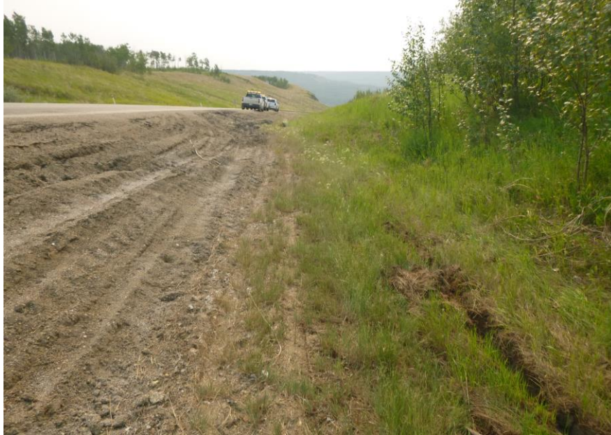
Photo 1 – Looking east along the south ditch from the tall dead tree landmark (~STA 3+060). Note the wet, soft, rilled shoulder and slumping highway embankment adjacent to the ditch which was graded in 2017. Also note the toe of a backslope slump encroaching into the ditch on this side of the vehicles.
