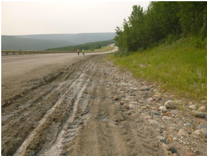
Photo 6 – Looking east along the riprap lined portion of south ditch, and the soft, distorted shoulder/highway embankment above it (~STA 2+760).
