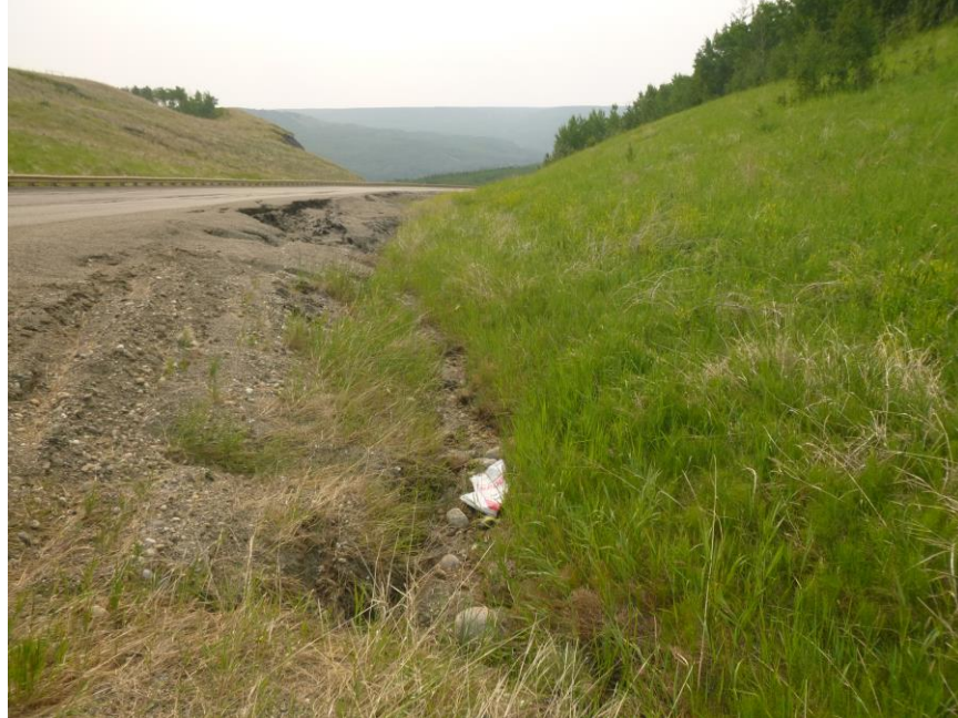
Photo 3 – Looking east along the south highway ditch from the west end of the guardrail (~STA 2+910). Note the patched, cracked and slumping south highway shoulder and embankment.
