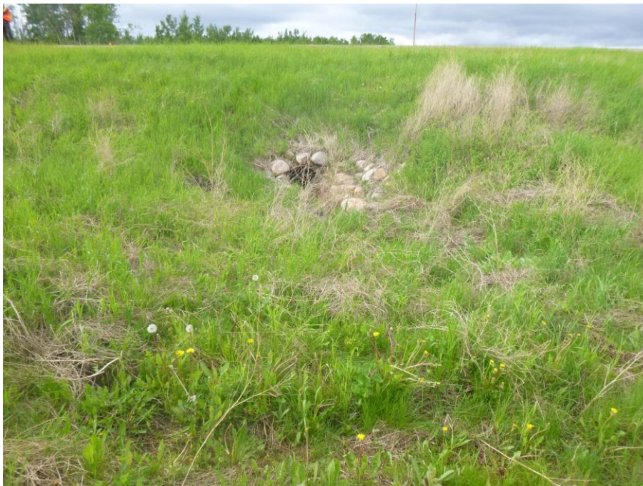
Photo 8 – Looking north at the inlet of the 900 mm dia. SWSP of Slide 1. A few cracks formed around the steeply sloping embankment surface around the inlet.
