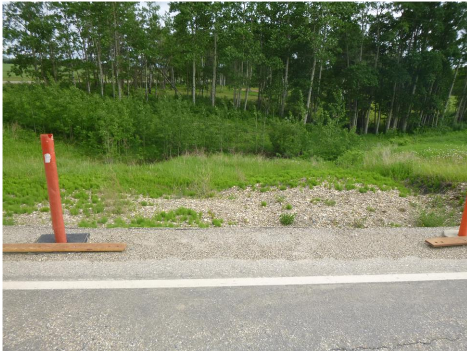
Photo 6 – Looking south from the highway over Slide 2.
