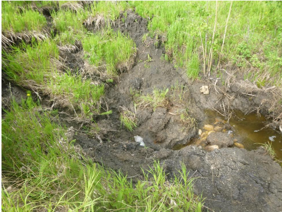
Photo 5 – Close-up view of the culvert inlet, where Slide 2 debris squeezed around and covered it.
