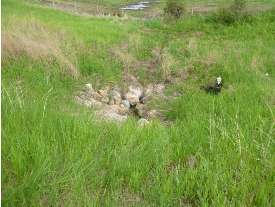
Photo 7 – Looking southeast at the drainage gully leading into the culvert inlet area on the opposite (south) side of the highway from Slide 1.
