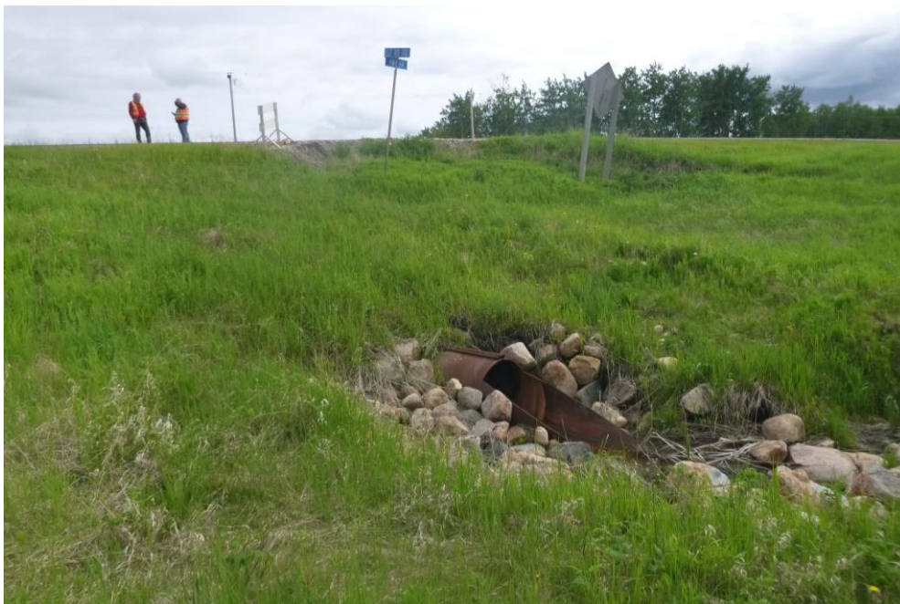
Photo 10 – Looking south across Slide 1 at the north highway embankment and the 900 mm dia. SWSP outlet.
