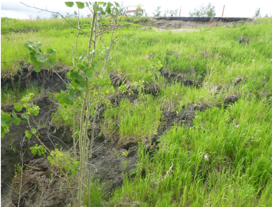
Photo 2 – Looking north (upslope) at Slide 2.
