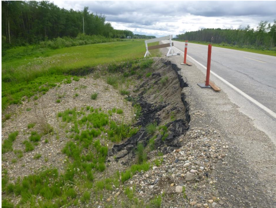
Photo 3 – Looking west along the highway embankment and scarp of Slide 2. Note the pitrun gravel that was placed overtop of the slide scarp adjacent to the highway continues to settle and move downslope.
