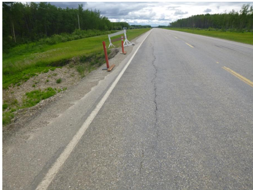
Photo 4 – Looking west at the crack in the highway EB lane OWP adjacent to the Slide 2 scarp.
