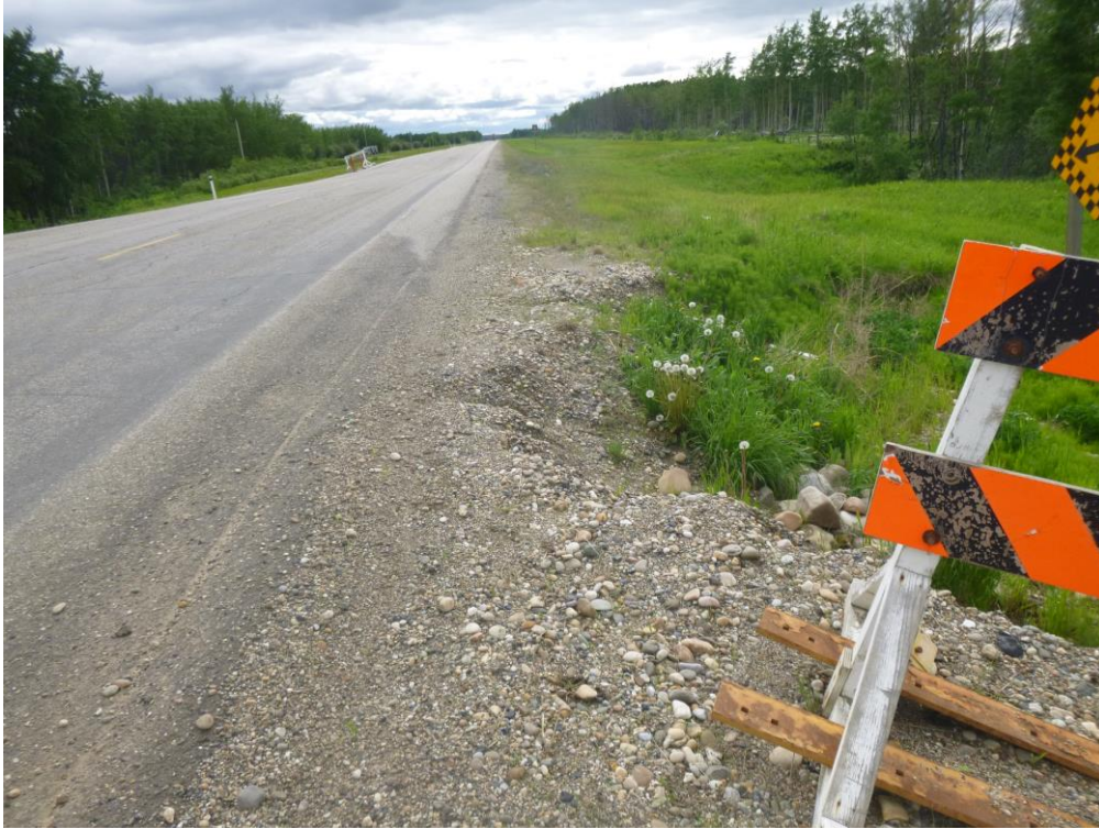
Photo 9 – Looking west adjacent to the hwy at the Slide 1 slide scarp. Note the dip in the hwy ovetop the culvert crossing at Slide 2 (in the background).
