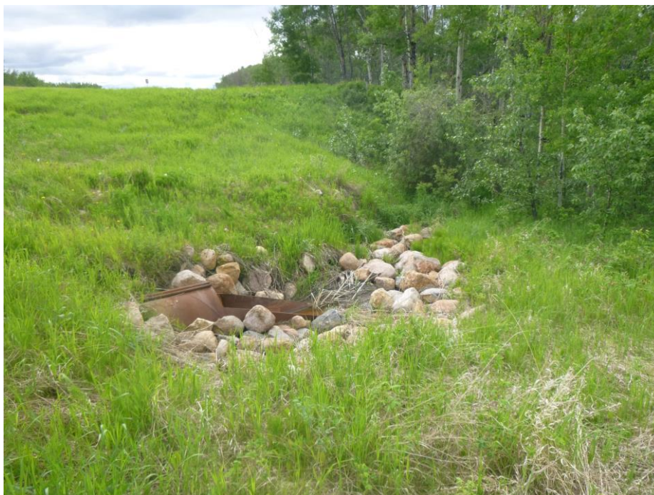
Photo 12 – Looking northwest at the outlet and downstream erosion gully of Slide 1.
