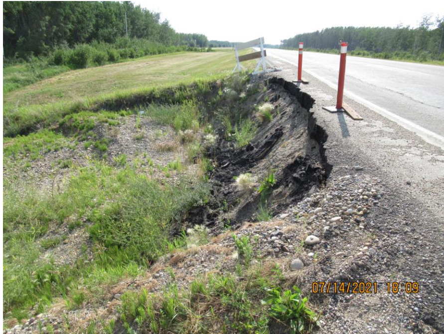
Photo 3 – Looking west along the highway embankment and scarp of Slide 2. Note the pitrun gravel that was placed overtop of the slide scarp adjacent to the highway continues to settle and move downslope.
