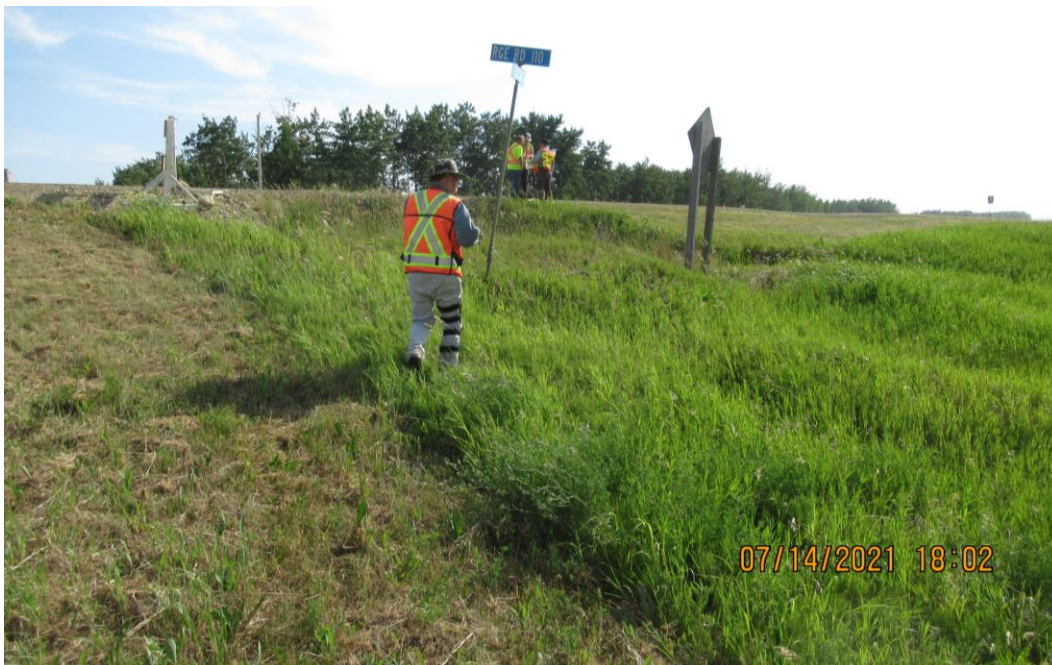
Photo 8 – Looking southwest towards the highway across Slide 1.
