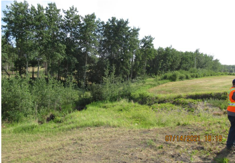
Photo 5 – Looking west across the culvert inlet area, where Slide 2 debris squeezed around and covered it, before it was excavated and partially opened.
