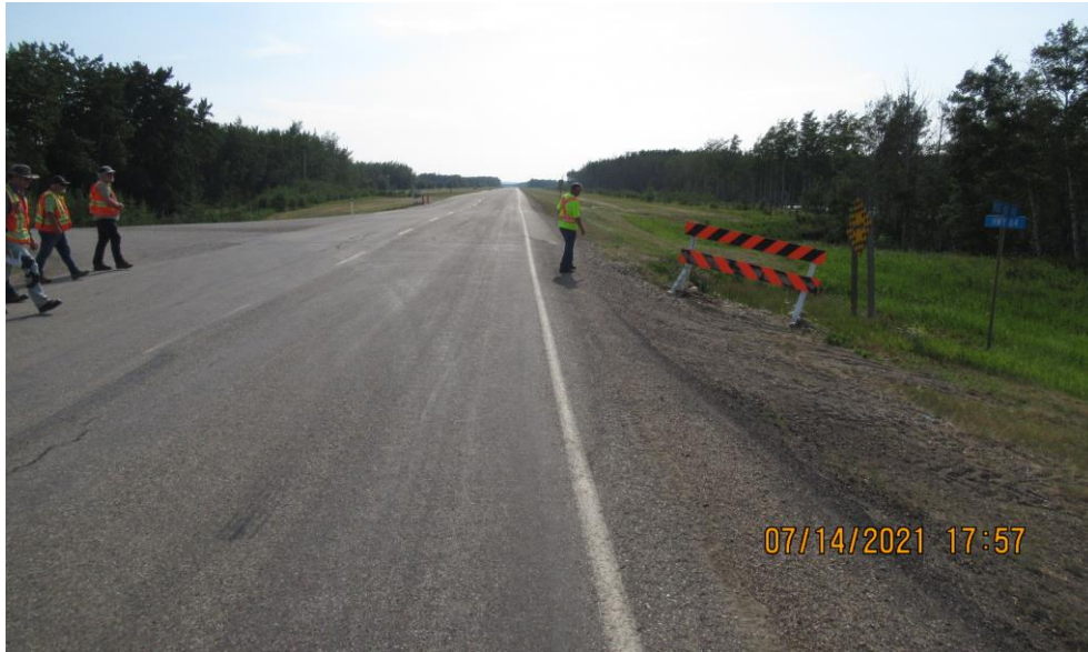
Photo 9 – Looking west adjacent to the hwy at the Slide 1 slide scarp. Note the dip in the hwy overtop the culvert crossing at Slide 2 (in the background).
