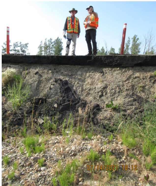
Photo 6 – Looking north at the slide scarp that has bit into the highway shoulder over Slide 2.
