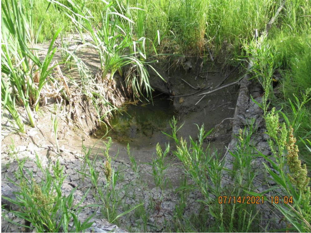
Photo 1 – Looking south at the outlet of the 900 mm diameter SWSP culvert of Slide 2 north of the hwy. The outlet is below ground, and somebody had dug around it to open it up.
