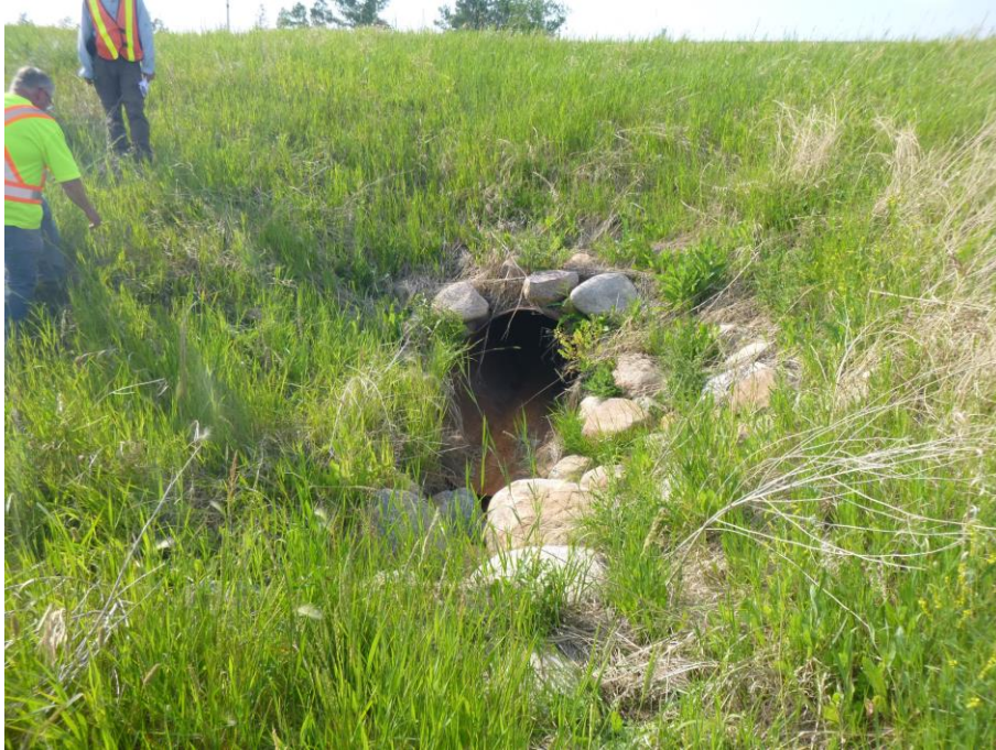
Photo 7 – Looking north at the 900 mm culvert inlet area on the opposite (south) side of the highway from Slide 1. A few cracks formed around the steeply sloping embankment surface around the inlet.
