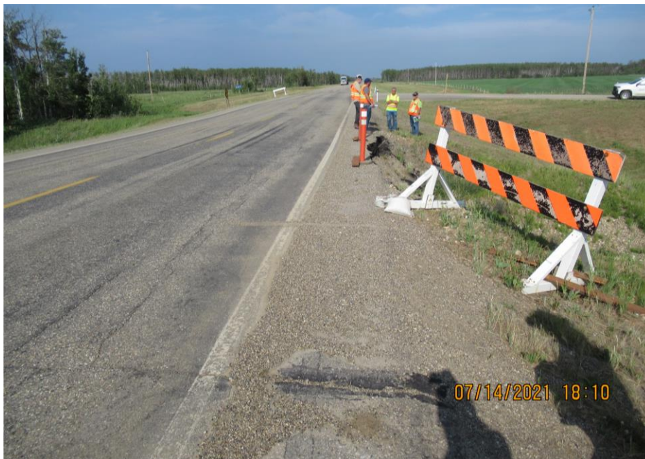
Photo 4 – Looking east along the crack in the highway EB lane OWP adjacent to the Slide 2 scarp.
