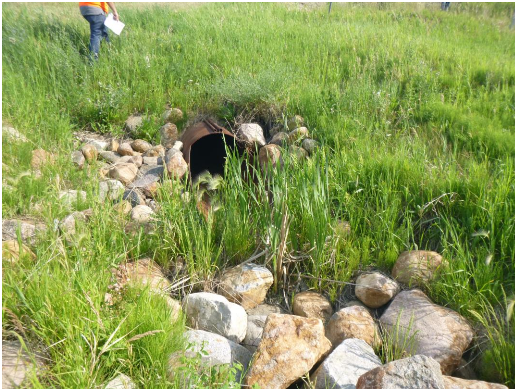
Photo 10 – Looking south at the 900 mm dia. SWSP outlet of Slide 1. Note the edge of the slide has moved right up to the edge of the culvert.
