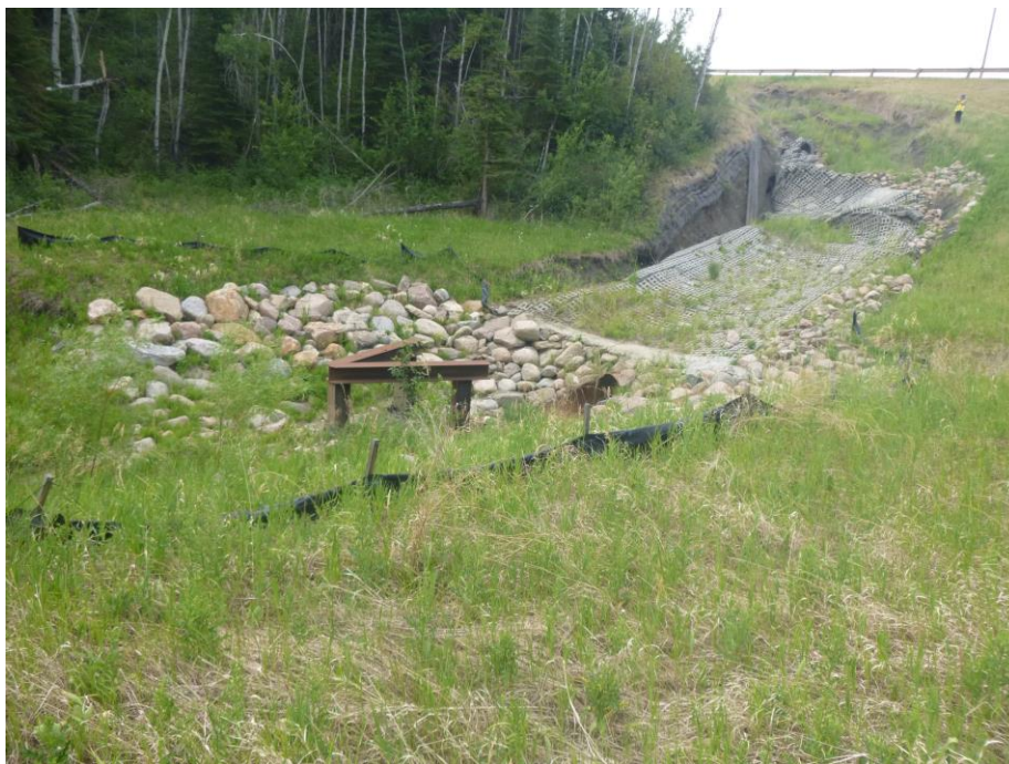
Photo 8 – Looking southeast at the culvert inlet and eroded ACB mat area leading to it.
