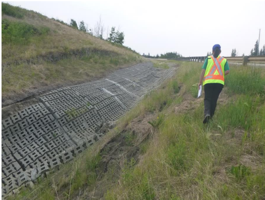
Photo 2 – Looking southeast along the edge of the eroded ACB mat area. Note the recent scarp extension along the south edge of the mats.
