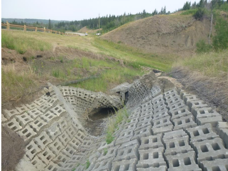
Photo 3 – Looking northwest along the severely damaged ACB mat area and enlarged slide scarp area.
