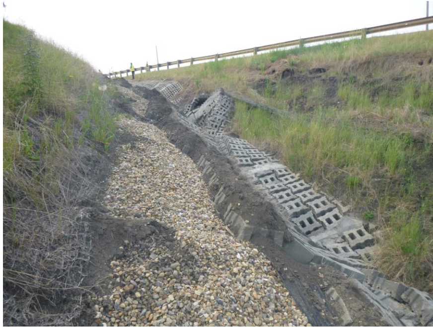
Photo 5 – Looking southeast along the north edge of the eroded ACB mats. Here the mats have slid down into the deeply eroded channel, exposing the underlying gravel.
