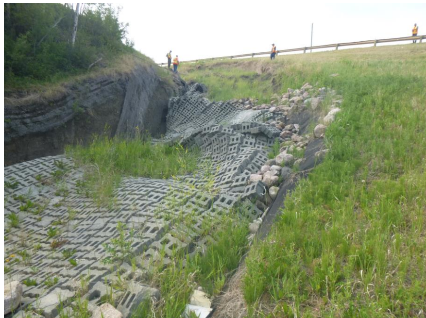
Photo 4 – Looking southeast at the severe erosion through the ACB mat and peripheral riprap areas. Note the enlarged erosion and slide developing south of the mats.
