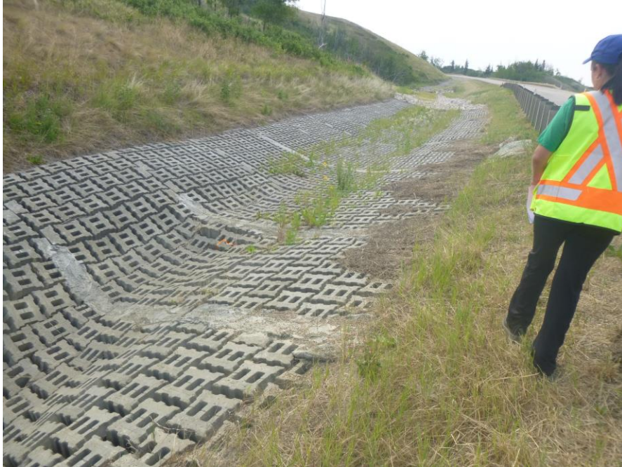
Photo 1 – Looking east along the beginning of the eroded ACB mat area north of the highway. The first 11 mats are still intact (1 east of the ribbon).
