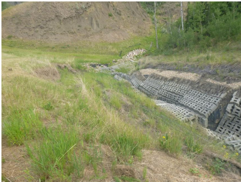
Photo 6 – Looking north along the southwest side of the damaged and eroded ACB mats.
