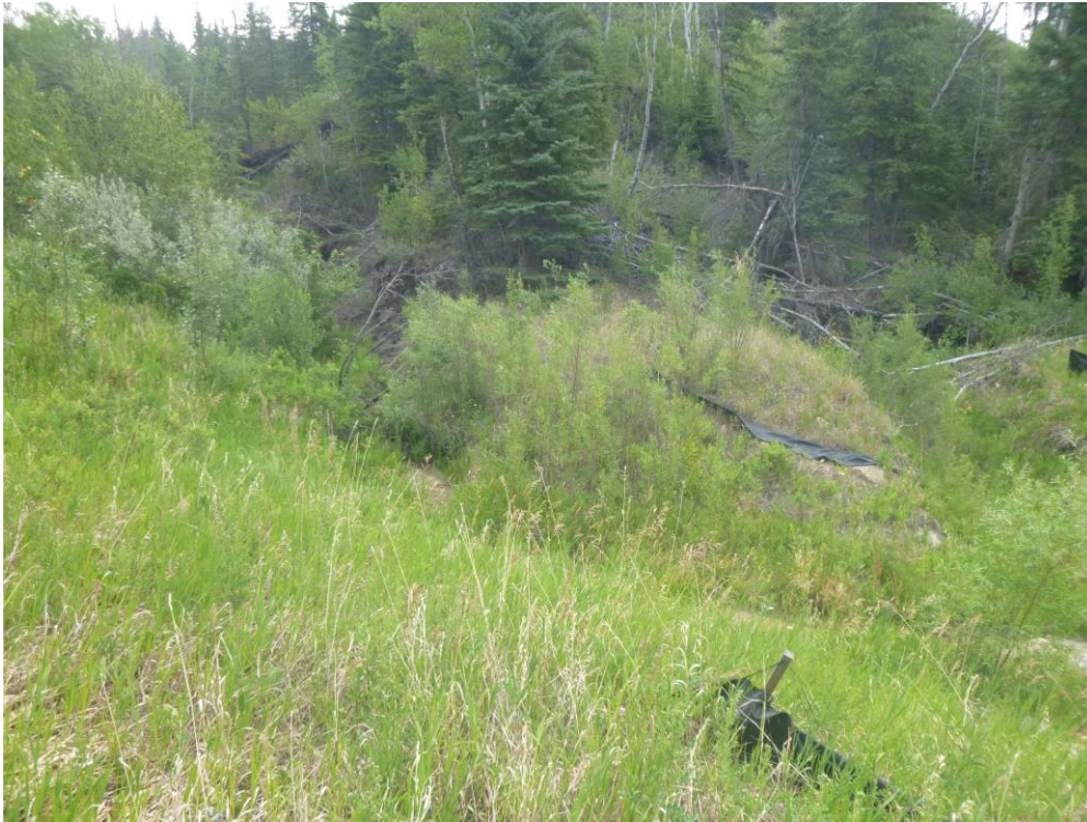
Photo 9 – Looking north at the slumping and infill occurring into the channel upstream of the 1524 SWSP culvert entrance.
