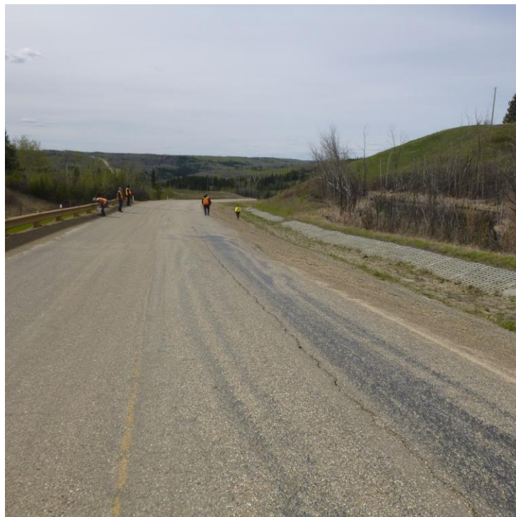
Photo 14 – Looking northwest at cracks in asphalt and dip in highway.
