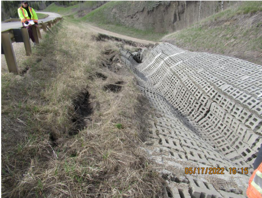
Photo 3 – Looking northwest along the severely damaged ACB mat area and enlarged slide scarp area.
