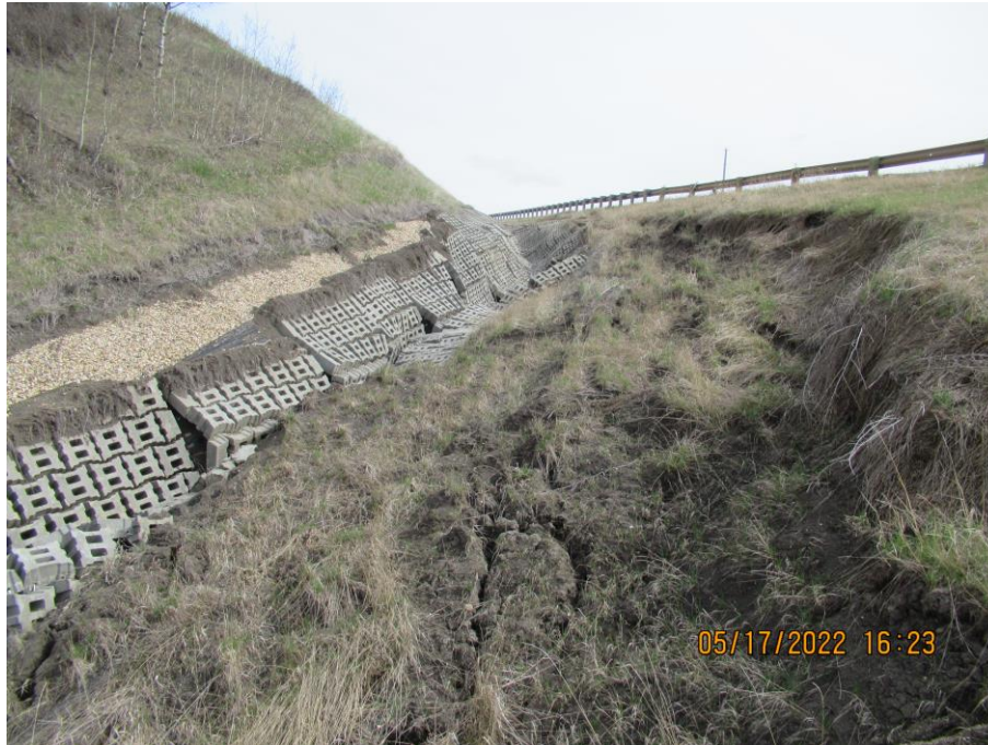
Photo 5 – Looking southeast along the north edge of the eroded ACB mats. Here the mats have slid down into the deeply eroded channel, exposing the underlying gravel.
