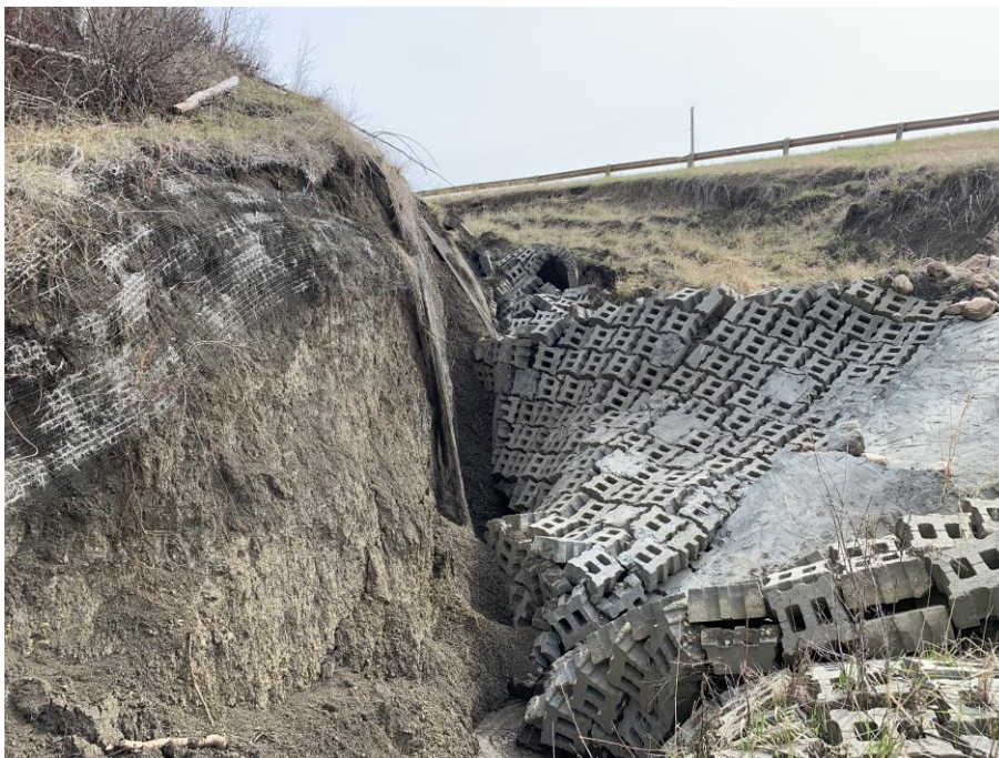
Photo 4 – Looking southeast at the severe erosion through the ACB mats. Note the enlarged erosion and slide developing south of the mats.
