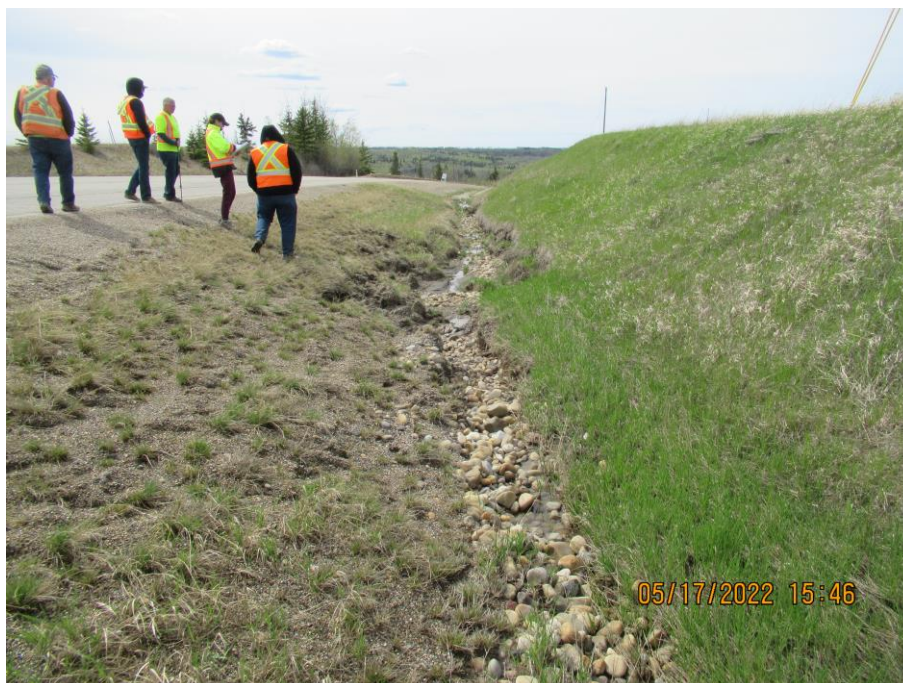
Photo 10 – Looking west at erosion that has formed uphill from the ACB matting.
