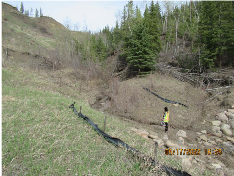
Photo 9 – Looking north at the slumping and infill occurring into the channel upstream of the 1524 SWSP culvert entrance.
