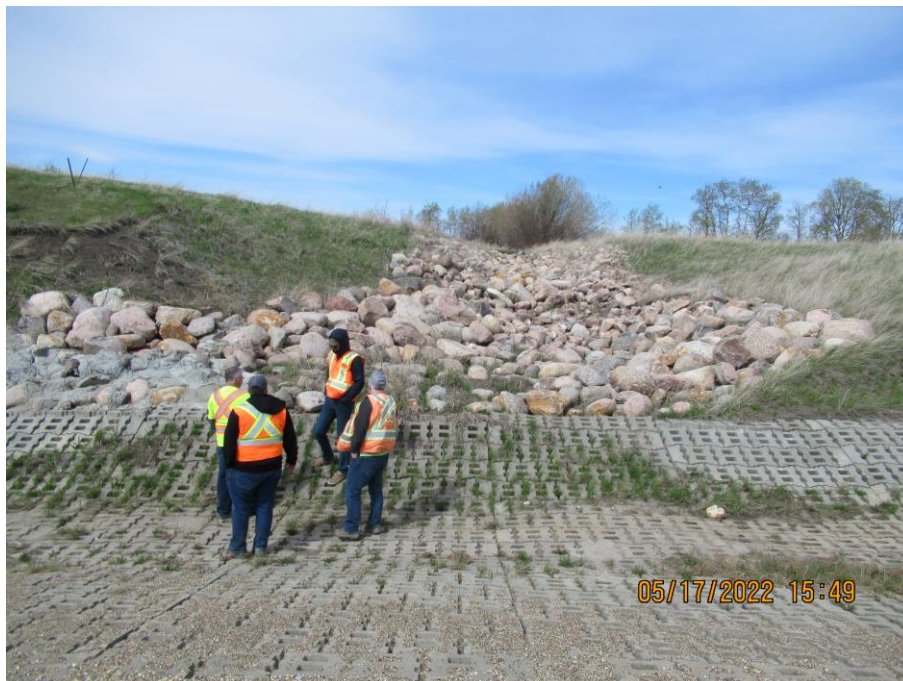
Photo 12 – Looking north at where riprap was previously placed, appears to be in good condition.
