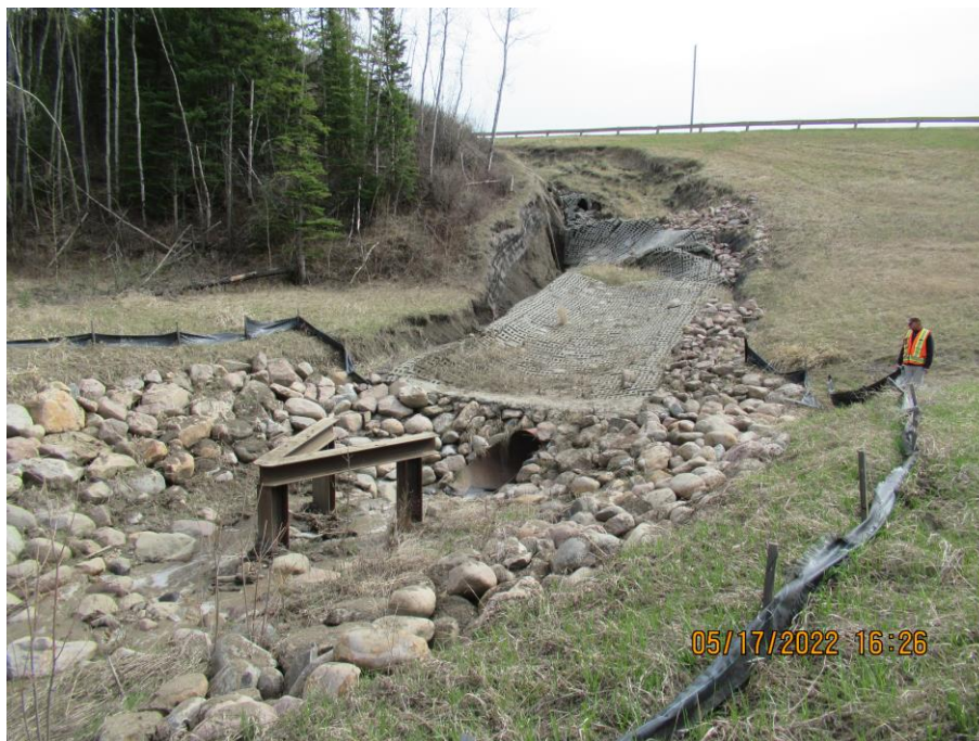
Photo 8 – Looking southeast at the culvert inlet and eroded ACB mat area leading to it.
