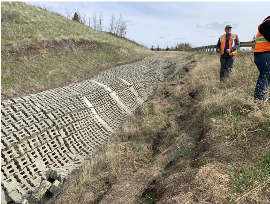
Photo 2 – Looking southeast along the edge of the eroded ACB mat area. Note the recent scarp extension along the south edge of the mats.
