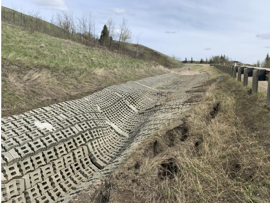
Photo 1 – Looking east along the beginning of the eroded ACB mat area north of the highway.
