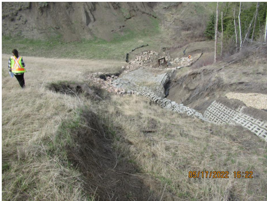
Photo 6 – Looking north along the southwest side of the damaged and eroded ACB mats.
