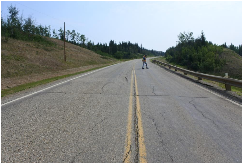
Photo 4 - Looking east along the highway at the crack/dip in the highway above the Slide at PH077-1.
