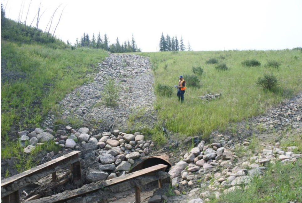
Photo 11 – Looking south at the culvert inlet area of the north embankment of PH077-2. The trash rack and culvert inlet were cleaned of debris since the 2020 inspection.
