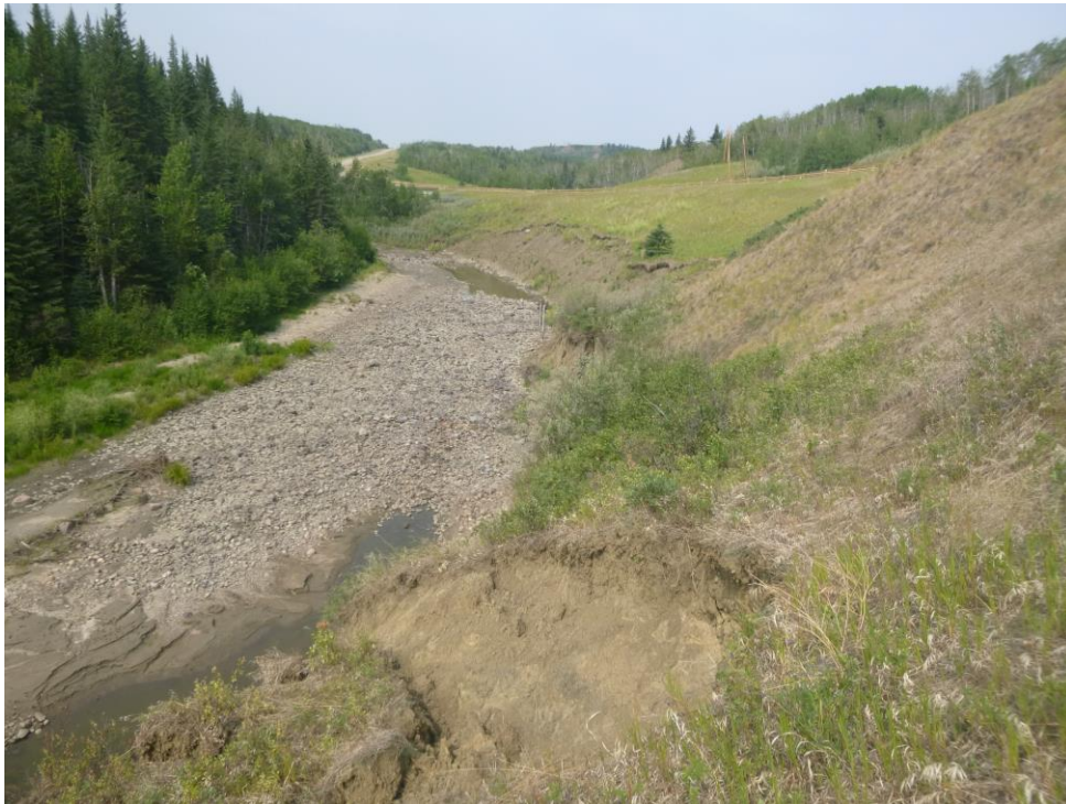
Photo 2 – Looking west at the fresh toe slumping above the creek at PH077-1 in the south highway embankment.
