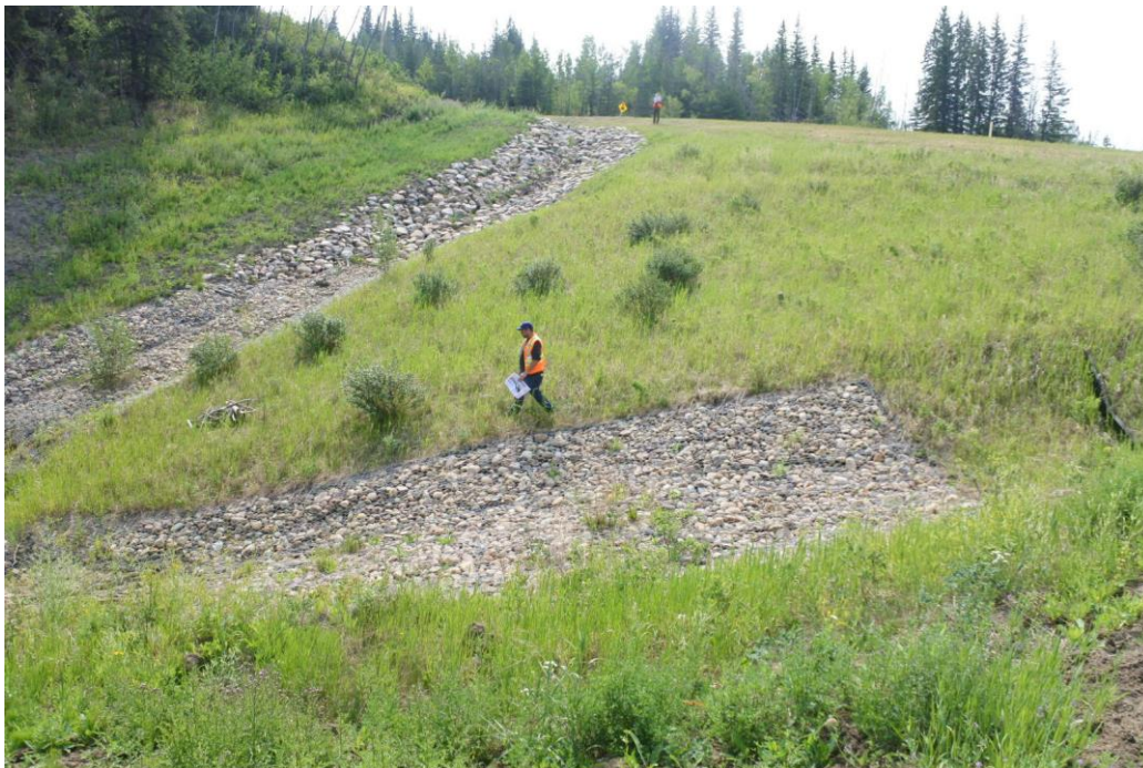
Photo 10 – Looking south at the erosion along the northeast ditch crotch leading to the culvert inlet area of the north embankment of PH077-2. The riprap protection has been extended further upslope on the east side since the 2020 inspection
