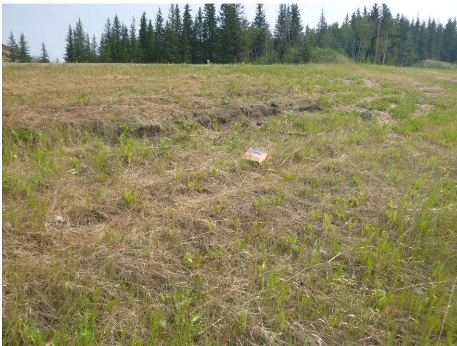
Photo 8 – Looking north towards the hwy from the south embankment of PH077-2, at the slide scarp in proximity to the highway.
