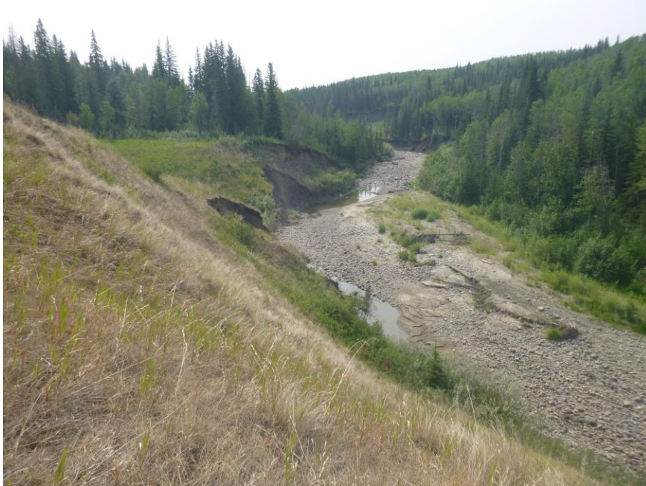
Photo 9 - Looking southeast at the culvert outlet area of PH077-2. Note the riverbank slumping east of the culvert outlet.
