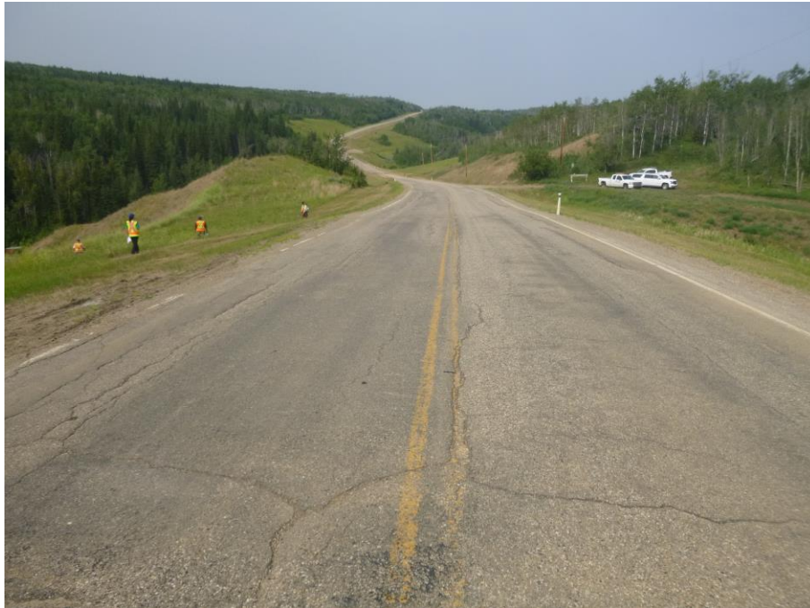
Photo 5 - Looking east along the highway across PH077-2. Note the settlement and cracking in the highway.
