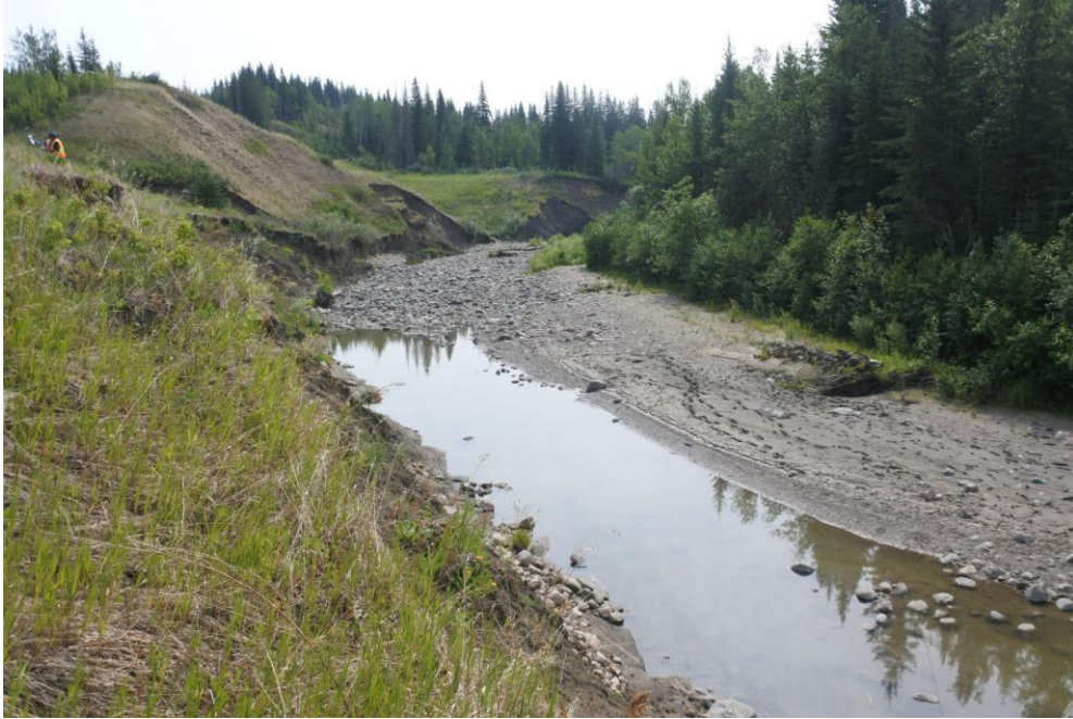
Photo 1 – Looking east at Slide PH077-1 at the erosion along the north side of the Creek.
