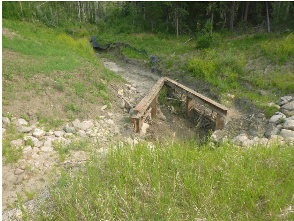
Photo 12 - Looking north along the infilled channel leading into the culvert inlet north of the highway at PH077-2.
