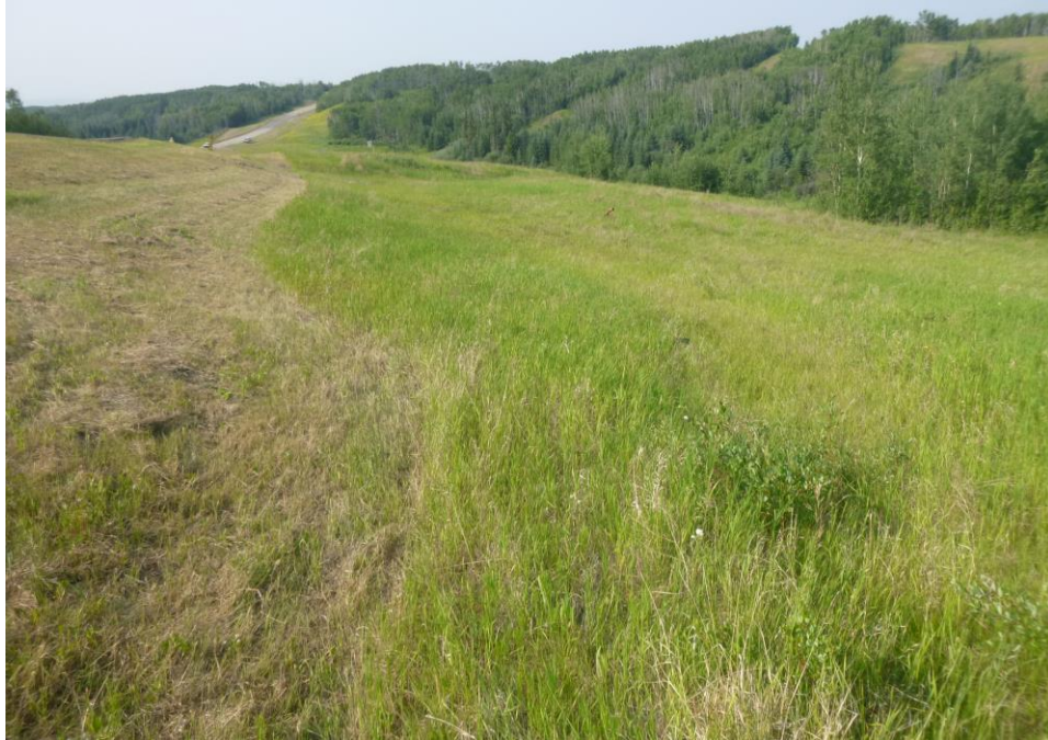
Photo 5 – Looking north along the east highway embankment from the south end of Slide Site 2.
