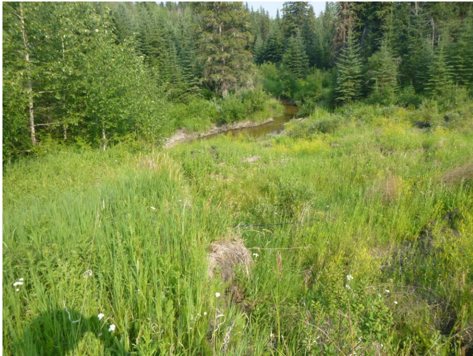
Photo 6 – Looking southeast at the outside bend of the river, which is causing the most active slumping area at Site 2.
