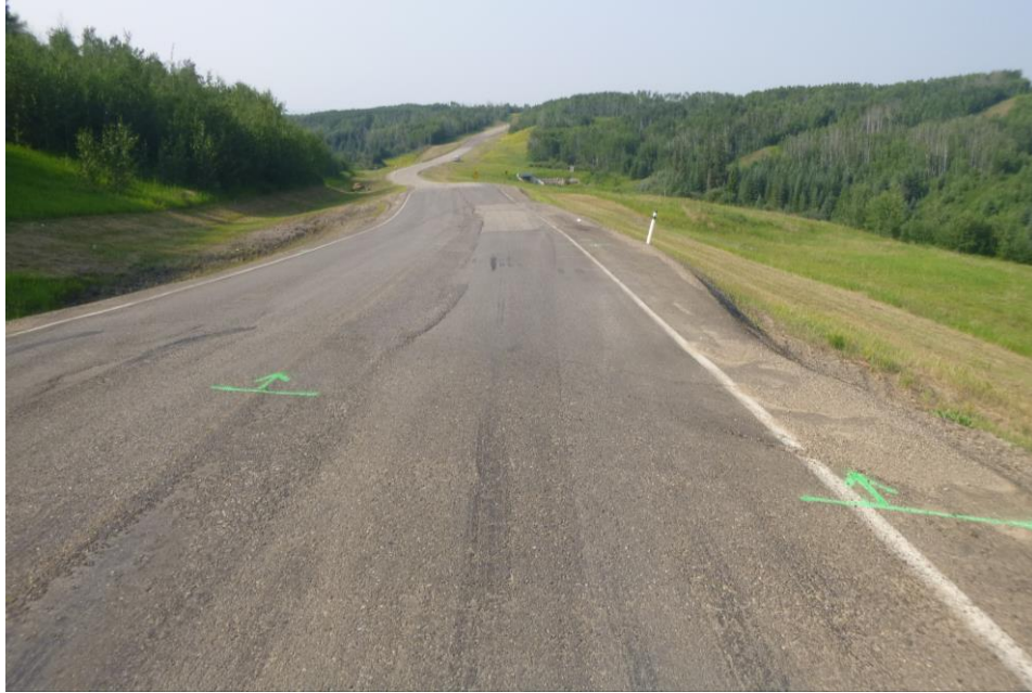
Photo 1 – Looking north from the south end of Slide Site 2 at the fresh milled/patched pavement. Note the more well-defined reflective south scarp crack extending into the east highway embankment.
