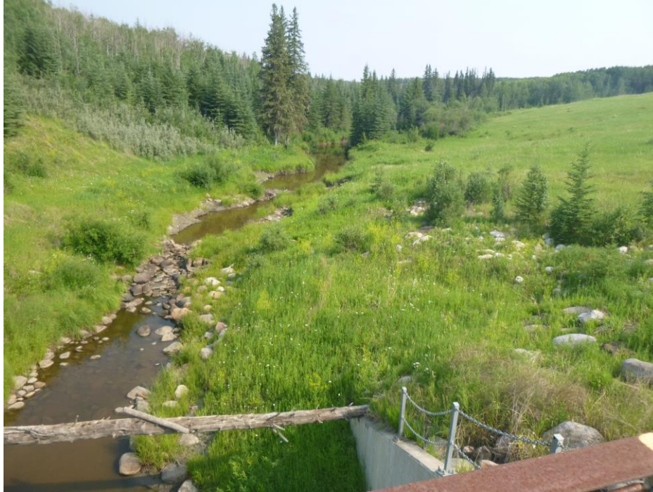
Photo 9 - Looking south along the River at the toe of Slide Site 1. Note in the background the piping erosion from the eroded gravel drain that has developed into a slump at the river toe.
