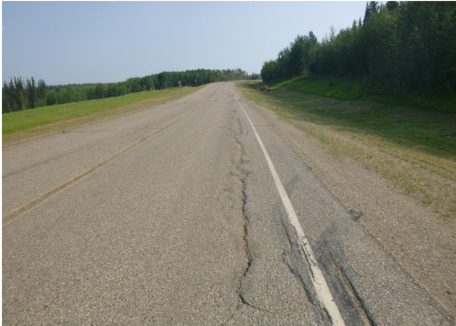
Photo 13 – Looking south towards Site 4 at the cracking/distortion along the highway directly above the Site 1 slide.
