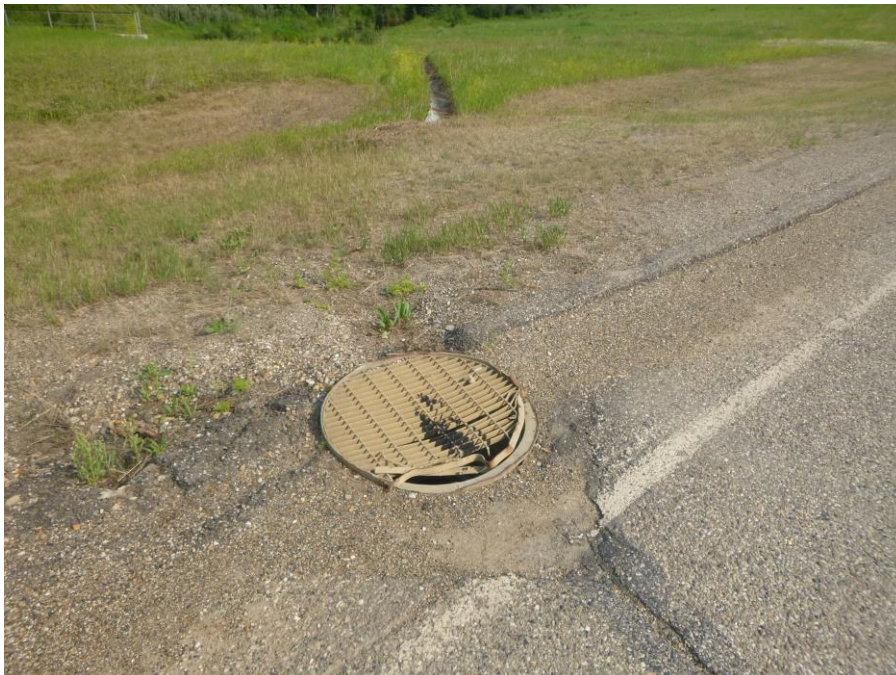
Photo 12 – Looking southeast at the damaged lid of the 800 mm diameter down drain along the east edge of the hwy that leads to the half culvert at Site 1.
