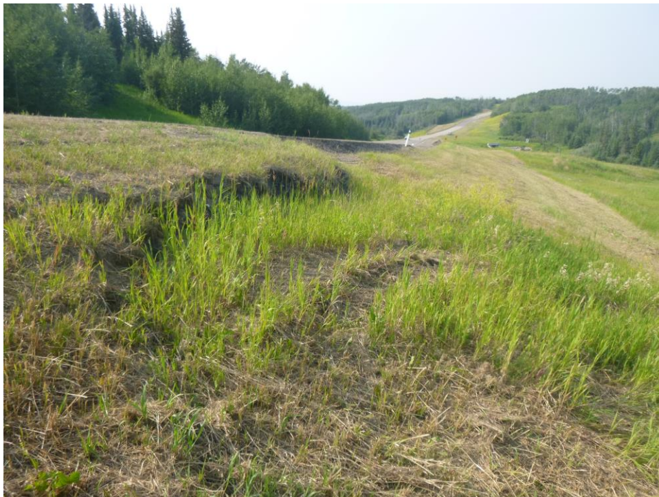
Photo 2 – Looking north across the south end of slide Site 2 and slide scarp extension along the east highway embankment.
