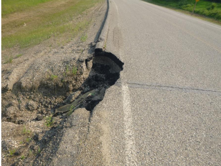
Photo 11 – Looking south along the east edge of the highway near the north end of Slide Site 1 where the AC curb has been breached, and runoff is causing erosion on the highway embankment and the edge of the pavement (it has extended to the white line this year).
