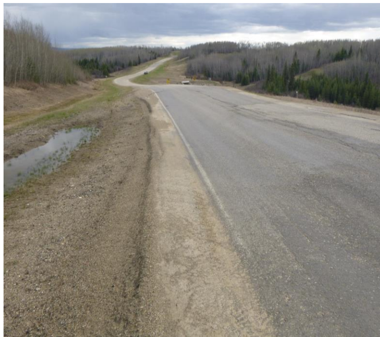
Photo 2 – Looking north from the Slide Site 2 at the fresh milled/patched pavement. Note the fresh, well-defined reflective north end scarp crack extending across the SB driving lane/shoulder.
