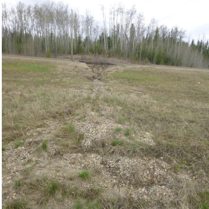
Photo 11 – Looking west towards the highway near the north end of Slide Site 1 where the AC curb has been breached, and runoff is causing erosion on the highway embankment and the edge of the pavement.
