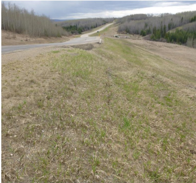
Photo 3 – Looking north across the south end of slide Site 2 and the slide scarp extension along the east highway embankment.
