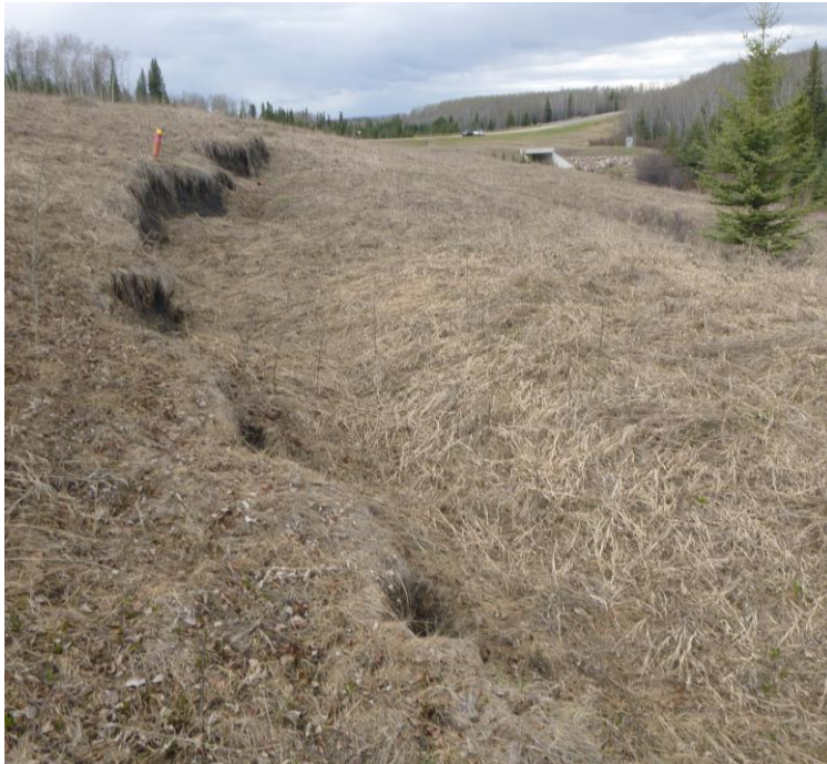
Photo 7 – Looking northwest along the fresh extended slide scarp/crack of Site 2, from just north of the most active portion of the slide.
