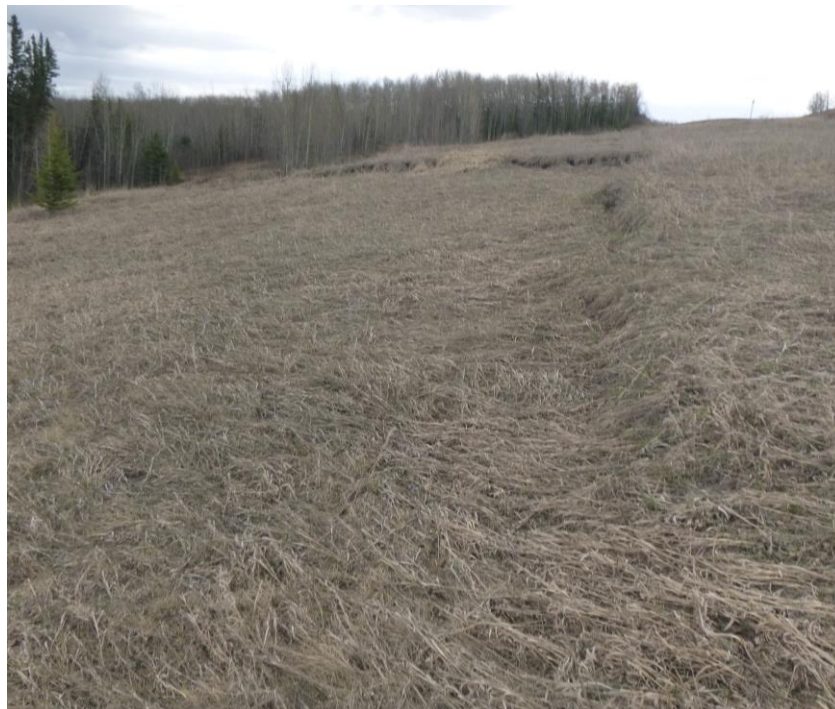
Photo 8 – Looking south along the north end of the slide scarp between Sites 2 and 4.
