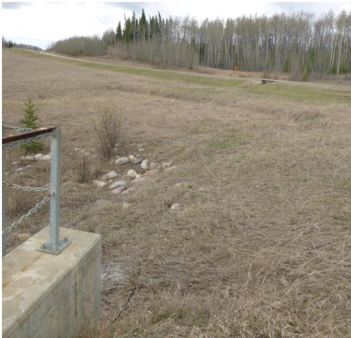
Photo 10 - Looking southwest across the Site 1 Slide from northeast of the river (Site 4 is on the left-hand side). Note the grassed over slide scarp parallel to the highway.
