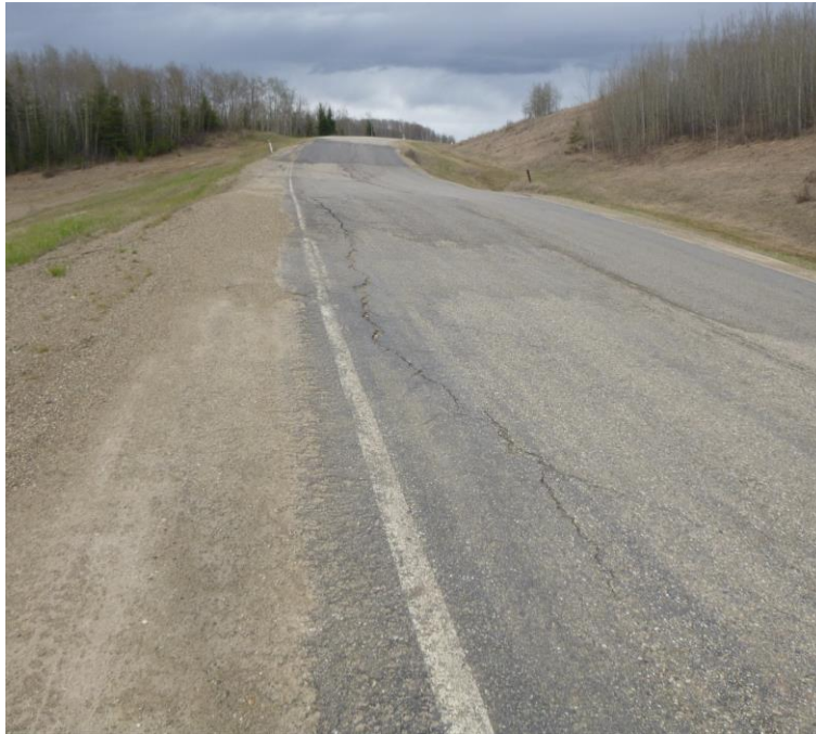
Photo 1 – Looking south at the slide scarp crossing the highway at Site 2. Note the dip in the highway, and the extended slide crack reflecting through the patch along edge of the NB driving lane.
