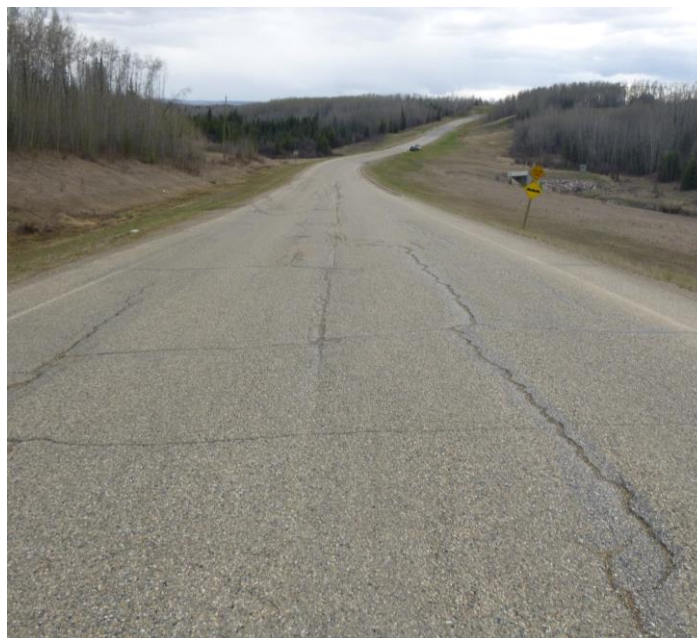
Photo 12 – Looking north from Site 4 at the cracking/distortion along the highway towards the Site 1 slide.
