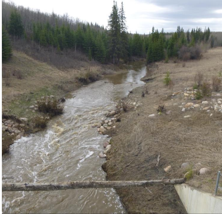
Photo 9 - Looking south along the River at the toe of Slide Site 1. Note in the background the piping erosion from the eroded gravel drain that has developed into a slump at the river toe.
