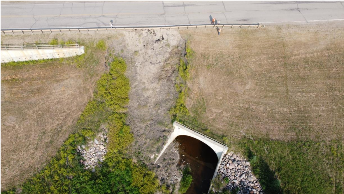
Photo 5 – Drone photo of the slide south of the pile wall at Site #3.
