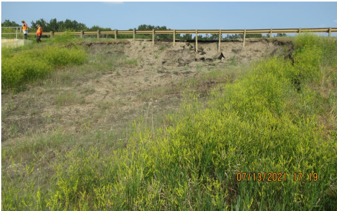
Photo 2 – Looking east at the body and scarp face of the slide at the south end of the pile wall at Site 3.
