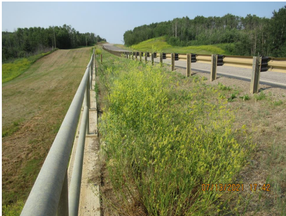
Photo 8 – Looking north along the top of the pile wall from near the south end. Note the gutter is filled with sand/debris, and the separated handrail.
