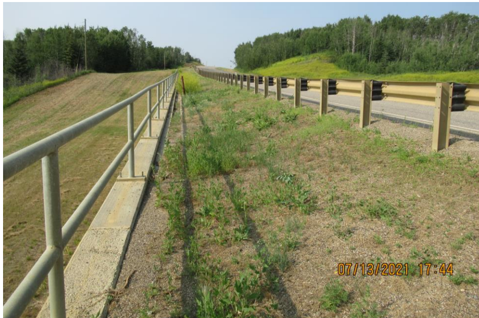
Photo 10 – Looking north along the area between the top of the pile wall and the guardrail. Note the infilled gutter.
