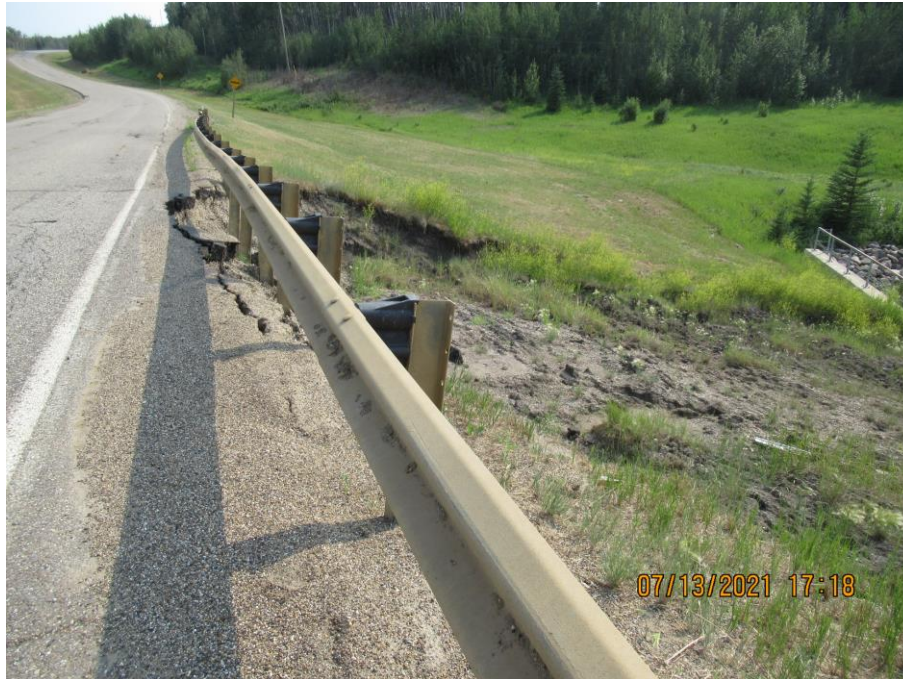
Photo 3 – Looking S. along the hwy at the slide scarp that has extended into the SB shoulder to within 0.3 m of the white line beyond the south end of the upper pile wall at Site #3.
