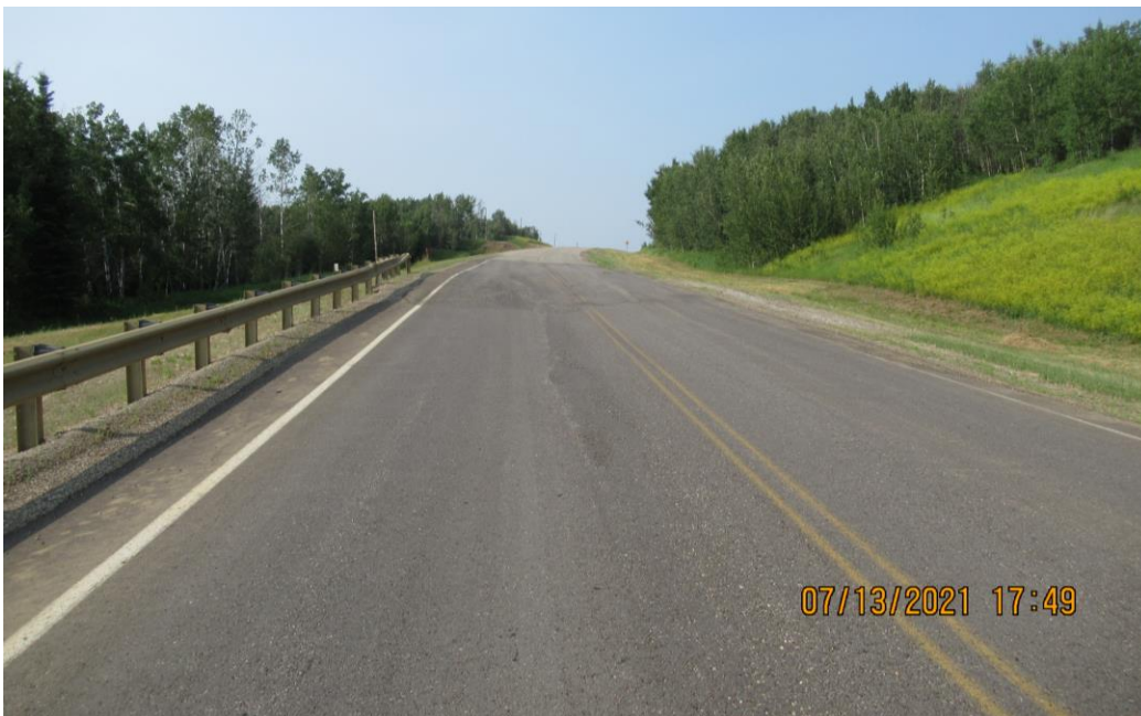
Photo 14 – Looking north along the highway at a fresh patch adjacent to the north end of the pile wall at Site 3. Note the hump near the north end of the Lightweight Fill.
