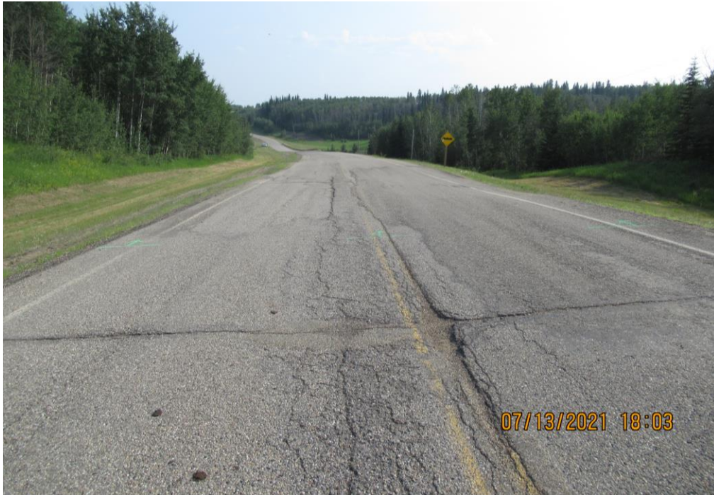
Photo 19 - Looking south along the highway at the fatigued pavement along the north end of Site 5. Note the settled east ditch and scarp that crosses the highway.
