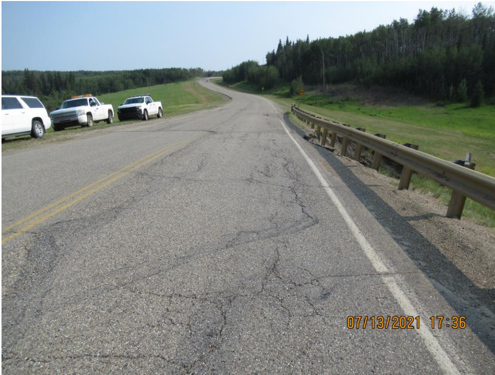
Photo 13 – Looking south along the highway at the map cracking adjacent to the south end of the pile wall and the slide further south.
