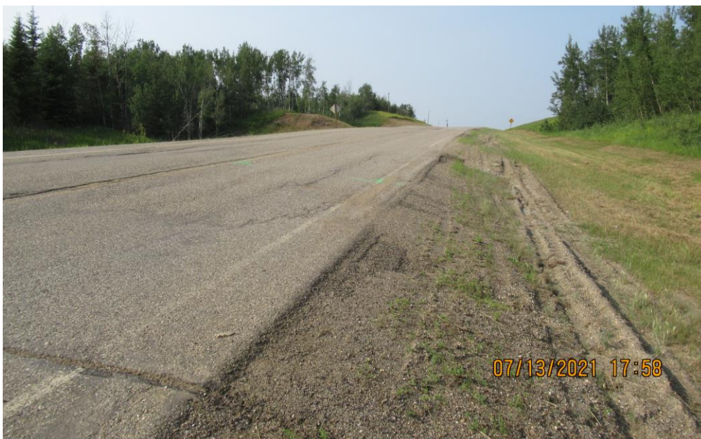
Photo 18 - Looking north along the east highway ditch and backslope slump at Site 5.
