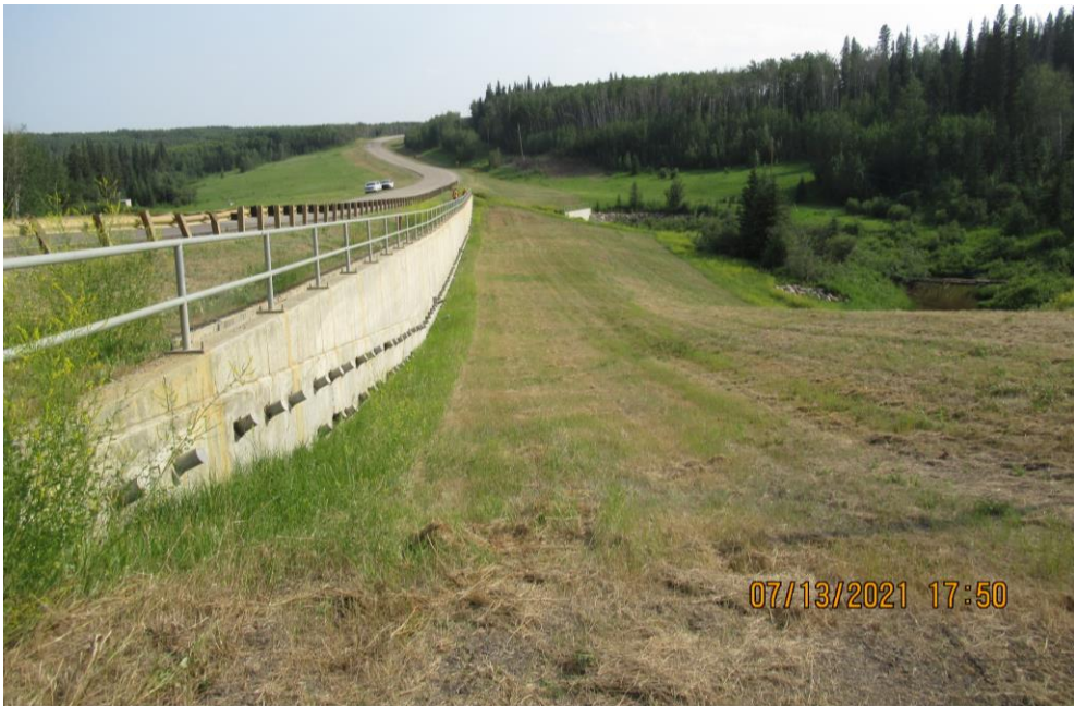
Photo 12 - Looking south along the upper pile wall and downslope embankment at Site 3.
