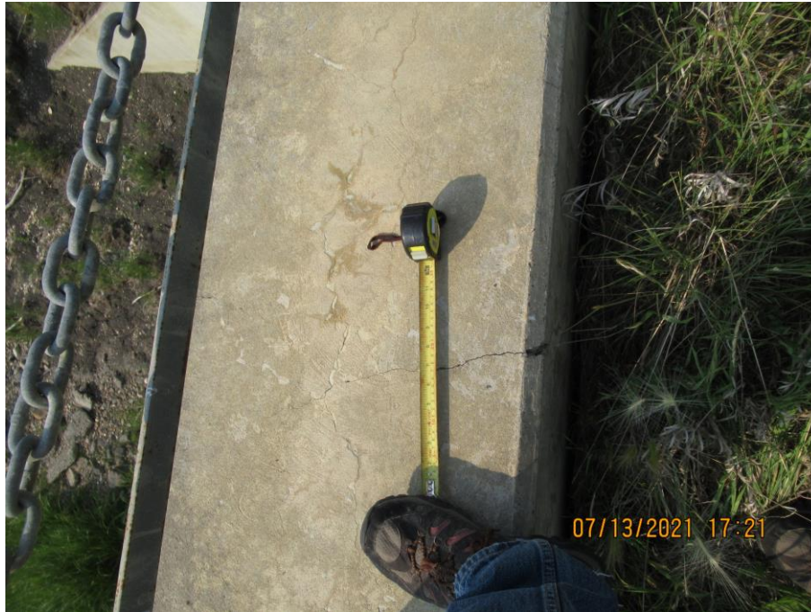
Photo 7 – Close up of a hairline crack in the arch culvert outlet headwall (4 m south of the north end).
