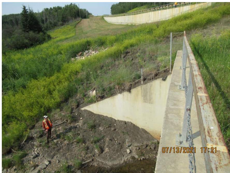
Photo 4 – Looking north at the toe of the slide that pushed debris against and around the arch culvert outlet headwall.
