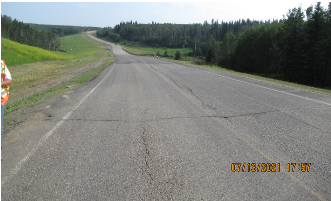
Photo 16 - Looking south along the highway at the distorted pavement and fresh patch further south, near the north end of Site 3/south end of Site 5. Note the broken Impact Attenuator on the north end of the guardrail.
