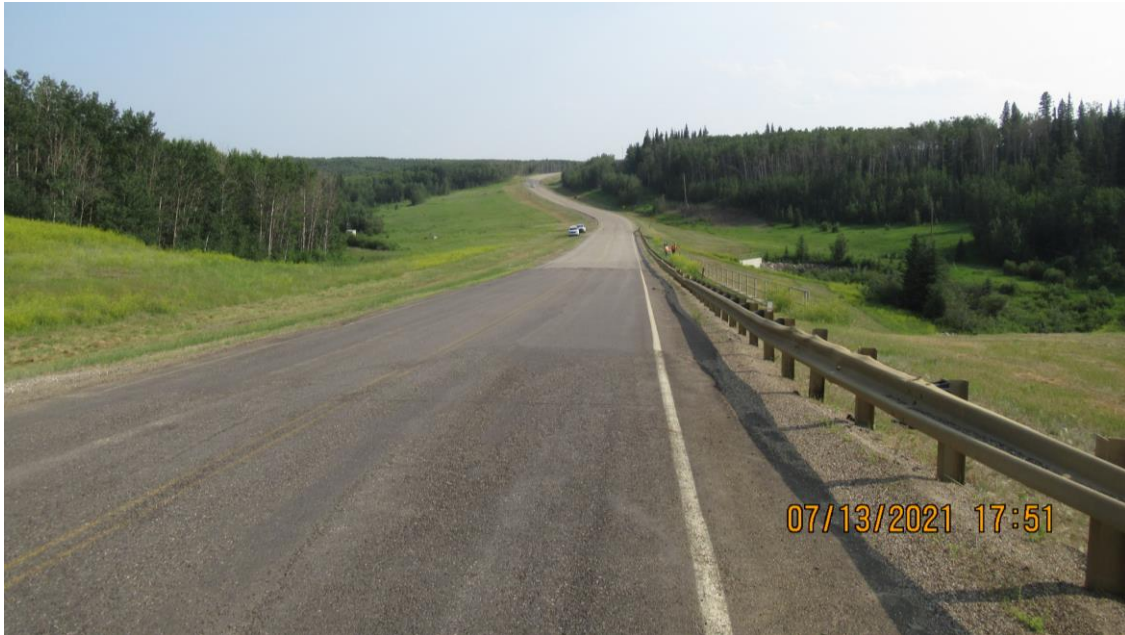
Photo 15 - Looking south along the highway from the hump in the fresh patch near the north end of the pile wall at Site 3.
