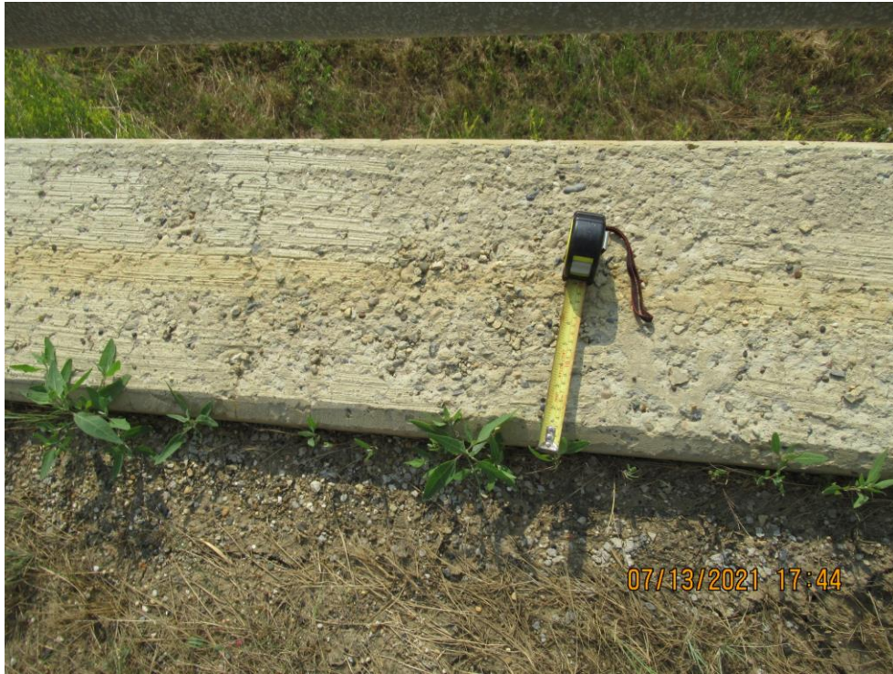
Photo 9 – Looking at the spalling concrete on the top of the upper pile wall of Site 3.
