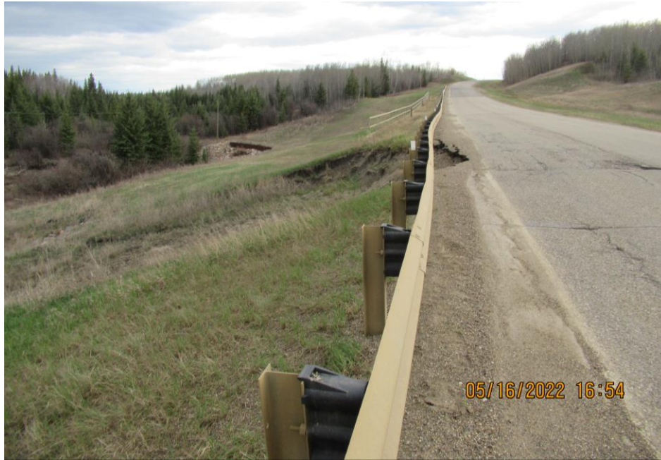
Photo 1 – Looking north along the highway south of the upper pile wall at the landslide that developed at Site 3.
