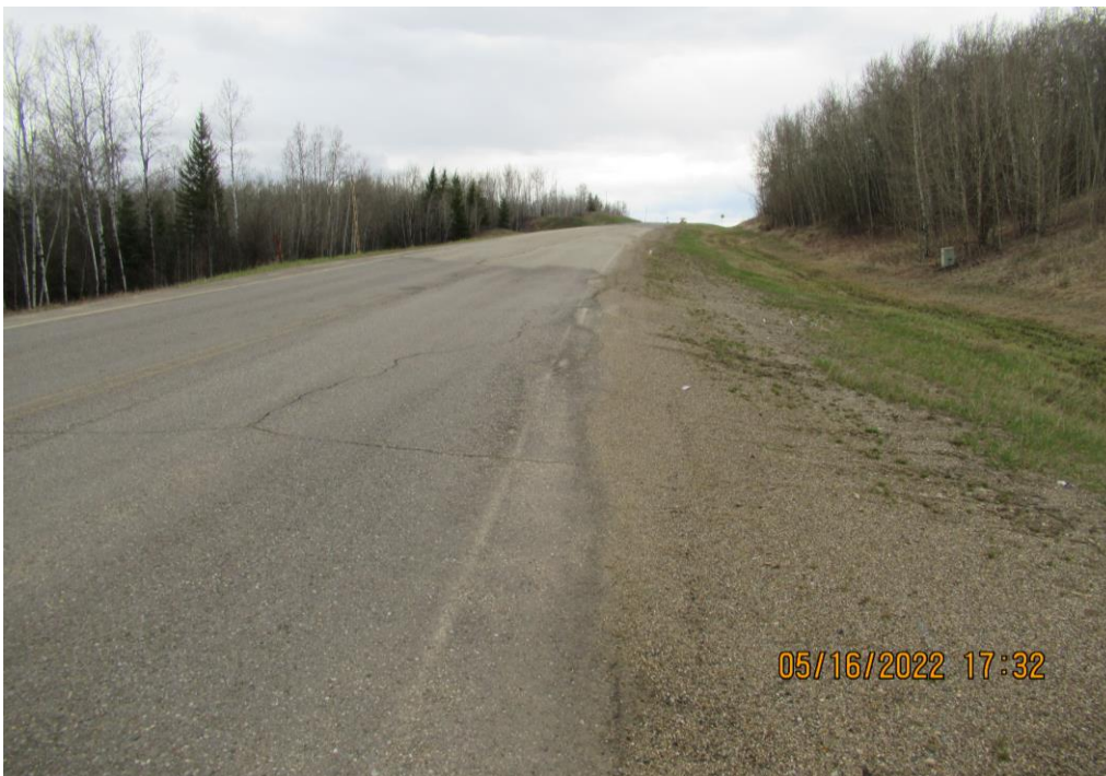
Photo 12 - Looking north along the highway at the distorted pavement and fresh patch, near the south end of Site 5.
