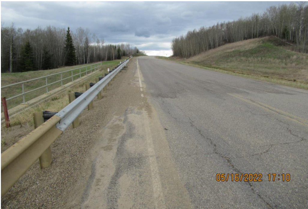
Photo 10 – Looking north along the highway at last year's patch adjacent to the north end of the pile wall at Site 3. Note the freshly placed guardrail, and the hump near the north end of the Lightweight Fill and guardrail.
