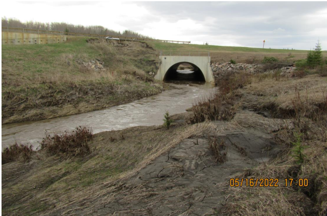
Photo 4 – Looking east at the body and scarp face of the slide between the south end of the pile wall and the arch culvert at Site 3.
