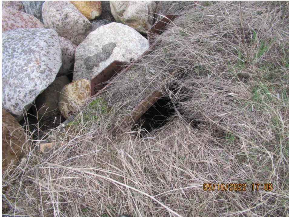
Photo 7 – Looking at the small void on the upslope side of the lower pile wall at Site 3.
