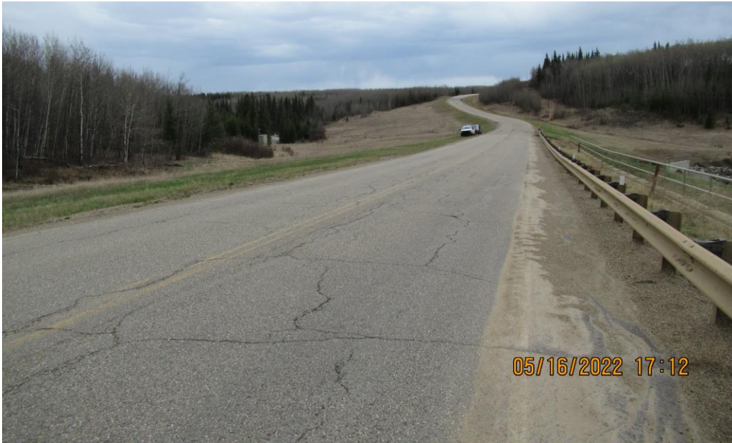
Photo 9 – Looking south along the highway at the highway map cracking adjacent to the south half of the pile wall at Site 3.
