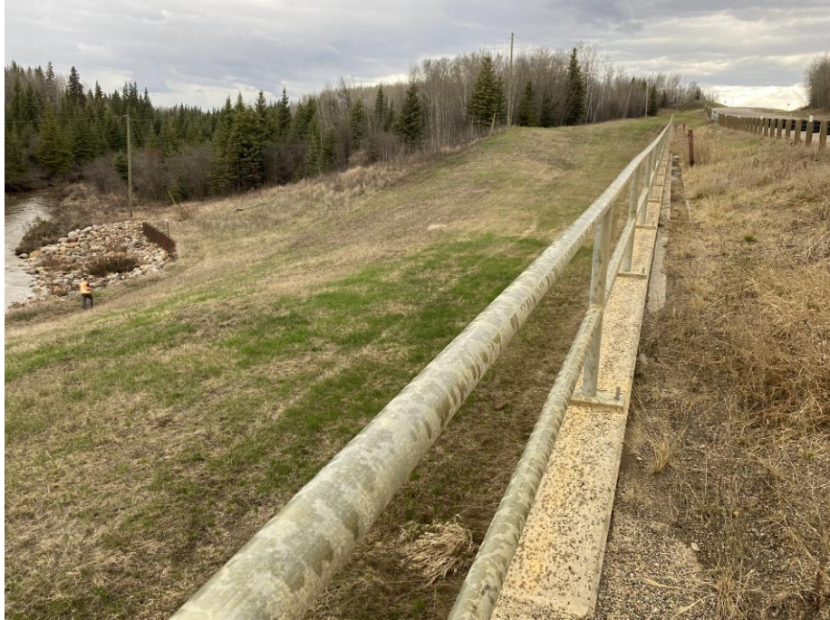
Photo 5 – Looking north along the top of the pile wall from near the south end at Site 3. Note the gutter is filled with sand/debris.
