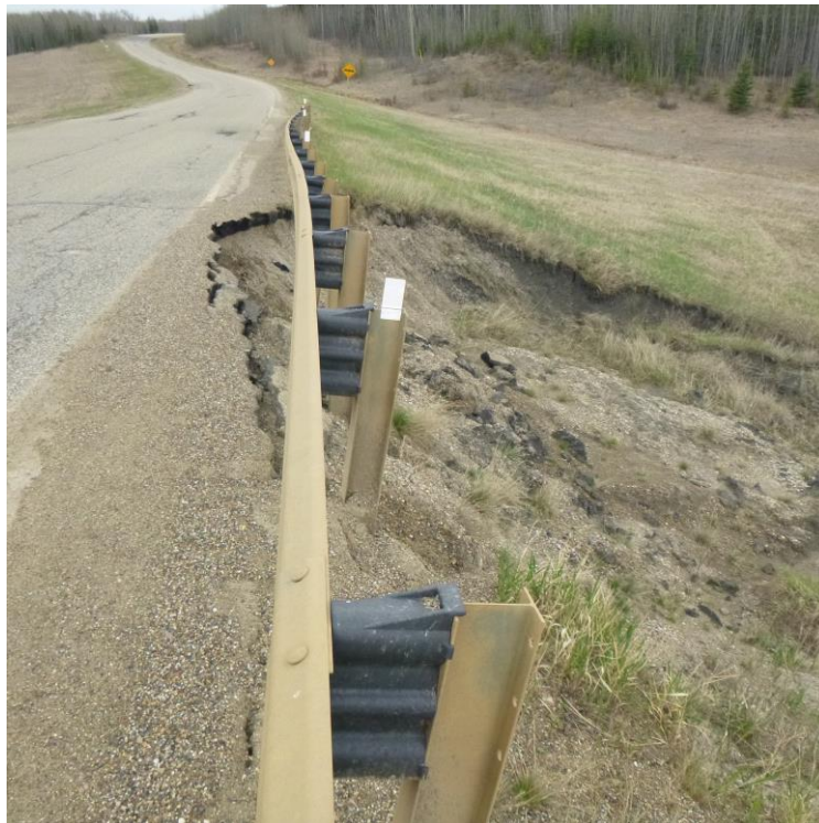
Photo 2 – Looking south at the slide scarp that has extended into the SB shoulder to within 0.3 m of the white line beyond the south end of the upper pile wall at Site 3.
