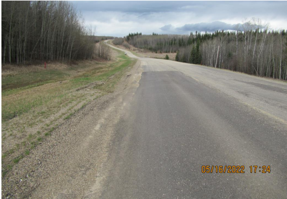
Photo 13 - Looking south along the highway at the subsidence in the NB driving lane and shoulder at Site 5.
