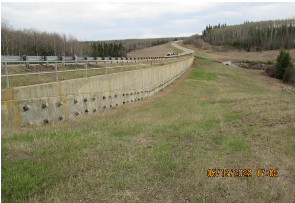
Photo 8 - Looking south along the upper pile wall and downslope embankment at Site 3.
