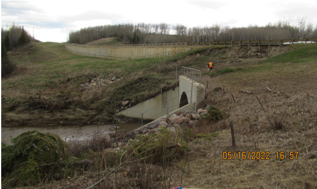
Photo 3 – Looking north at the toe of the slide that pushed debris against and around the arch culvert outlet headwall at Site 3. Note the cut trees on the south side of the arch culvert.
