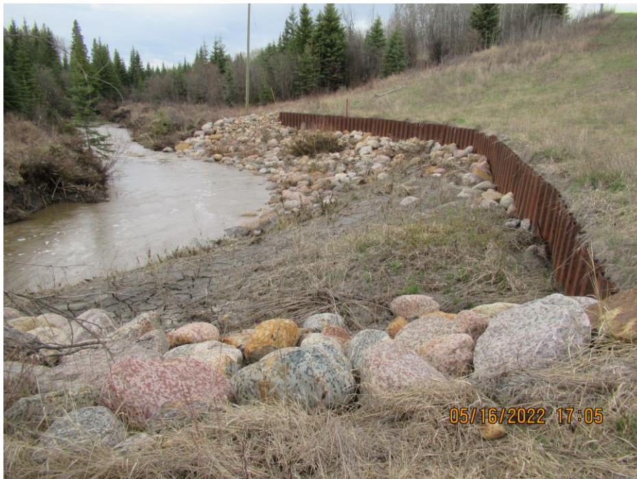
Photo 6 – Looking northwest at the lower pile wall area and riprap behind it at Site 3.
