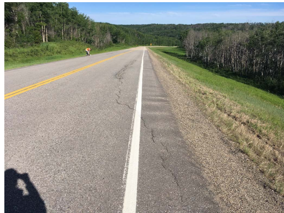
Photo 5. Crack near middle of southmost patch which may be a scarp crack from arch shape.
