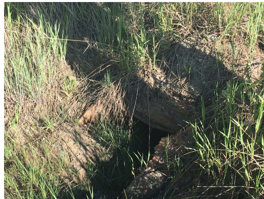
Photo 8. Culvert inlet patially damaged and blocked.
