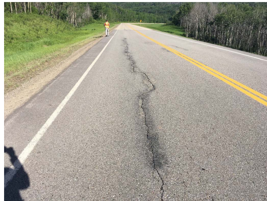
Photo 6. Cracks on southern asphalt patch in northbound lane.
