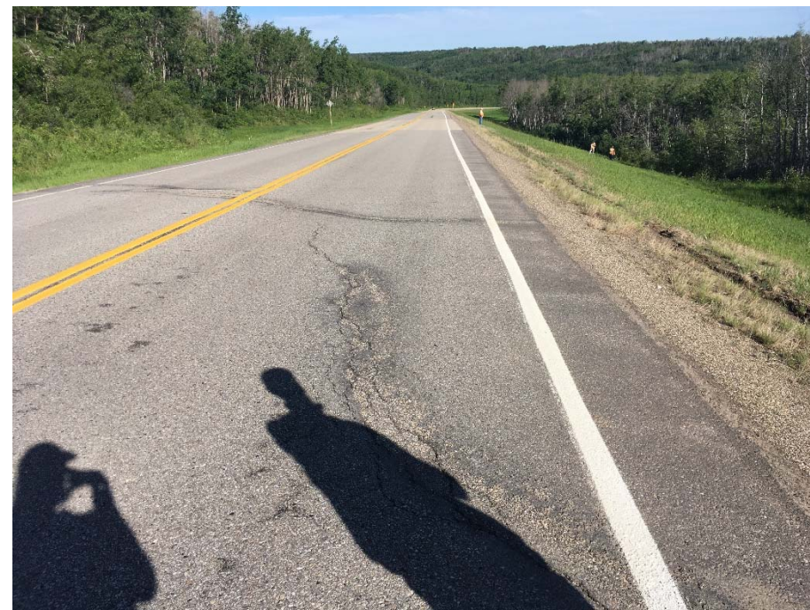
Photo 3. Crack near middle of northmost asphalt patch.
