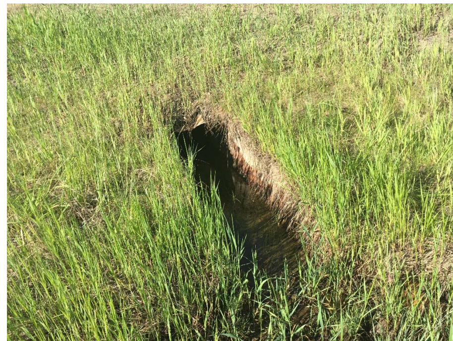
Photo 7. 600 mm CSP culvert outlet with water ponding around outlet.
