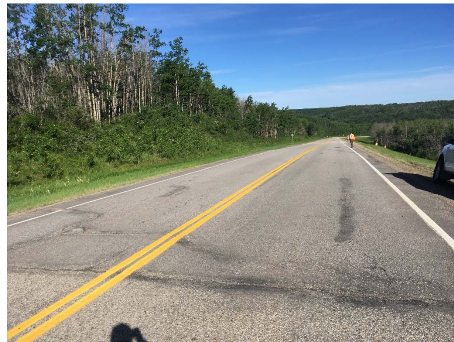
Photo 2. Cracks reflecting through patch in pavement.
