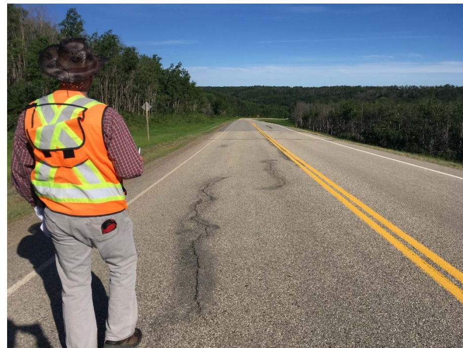
Photo 4. Cracks on asphalt in between the two patches.
