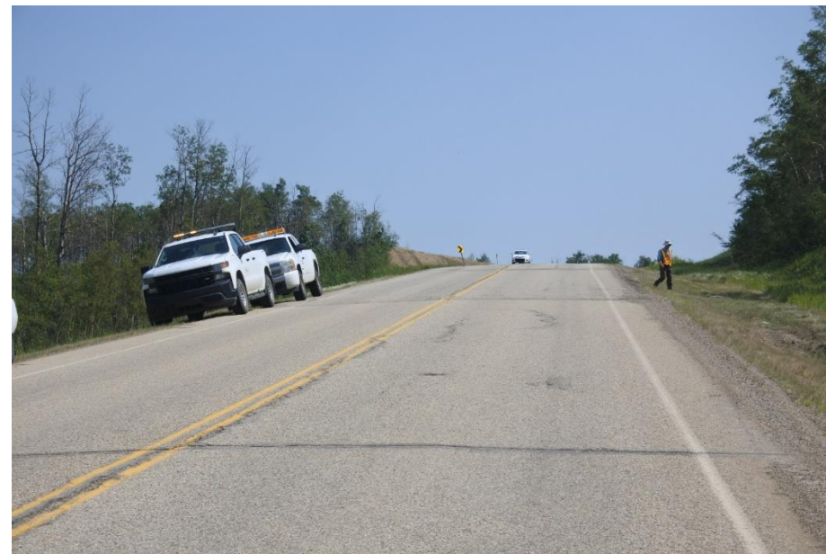
Photo 2. Cracks reflecting through patch in pavement.
