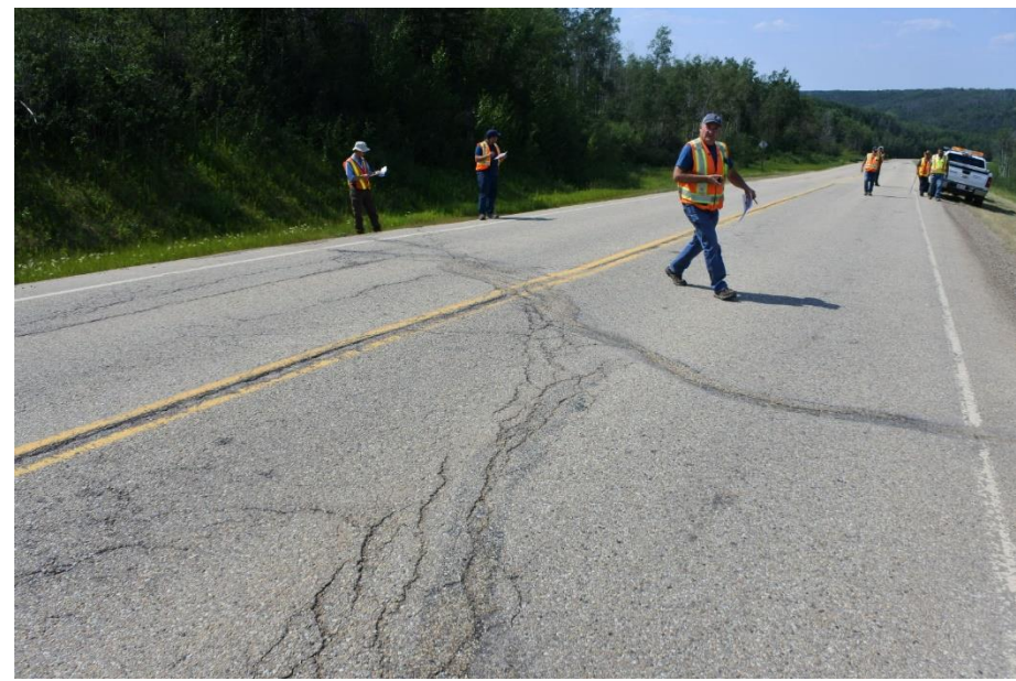
Photo 3. Crack near middle of northmost asphalt patch.
