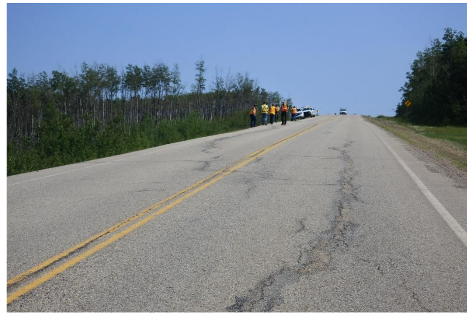
Photo 8. Looking northwest at cracks in pavement on south portion of the site.
