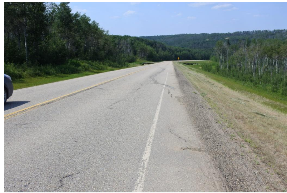
Photo 5. Crack near middle which may be a scarp crack from arch shape.
