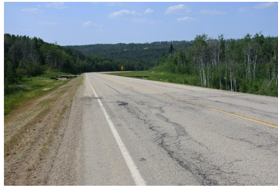
Photo 6. Cracks on southern asphalt patch in northbound lane.
