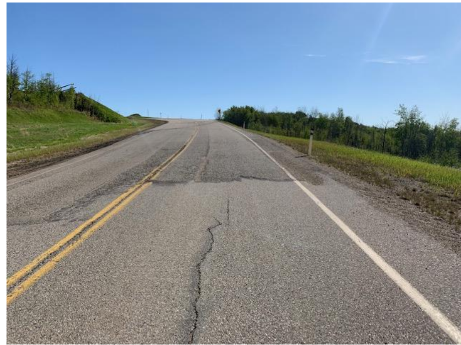
Photo 4. Looking northeast along Hwy 733 (former north slide) Possible tension crack.
