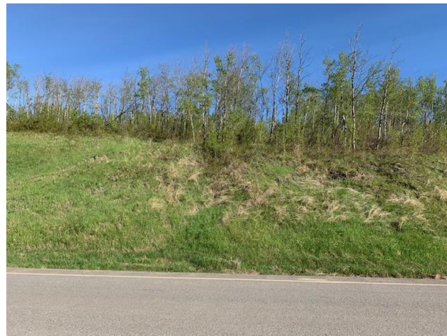
Photo 5. Looking northwest at backslope slump
