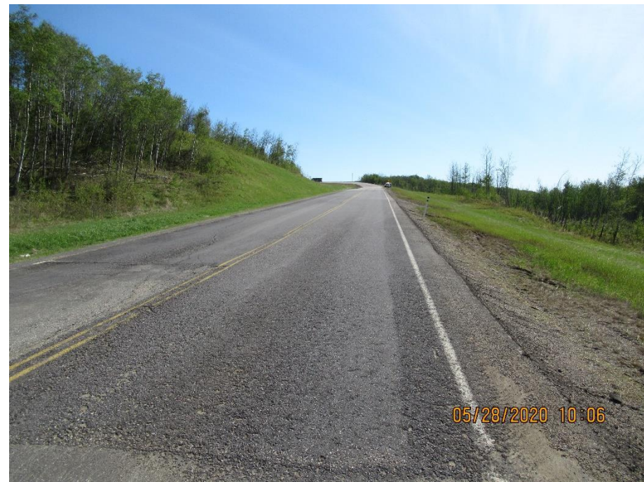
Photo 10. Looking northeast near the middle of the former south slide.
