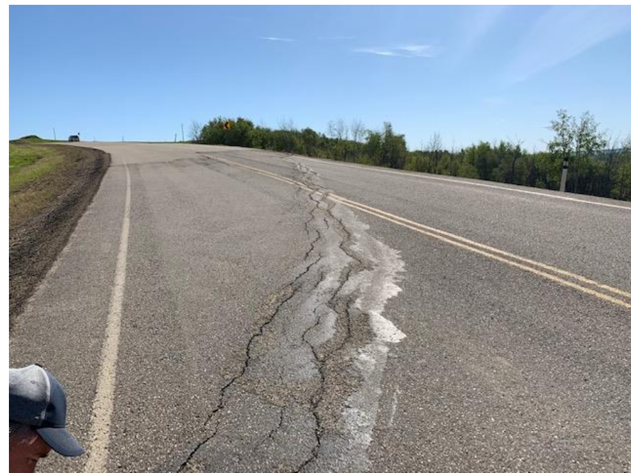
Photo 3. Looking northeast along Hwy 733 at scarp crack which extends into should and embankment (former north slide)
