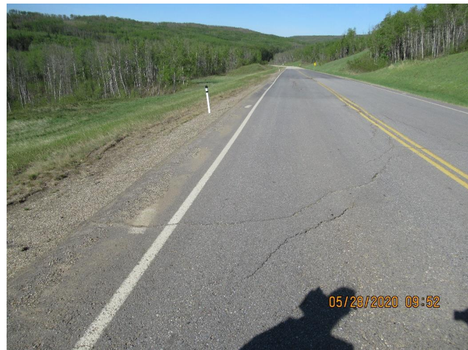
Photo 6. Looking southwest (former south slide).
