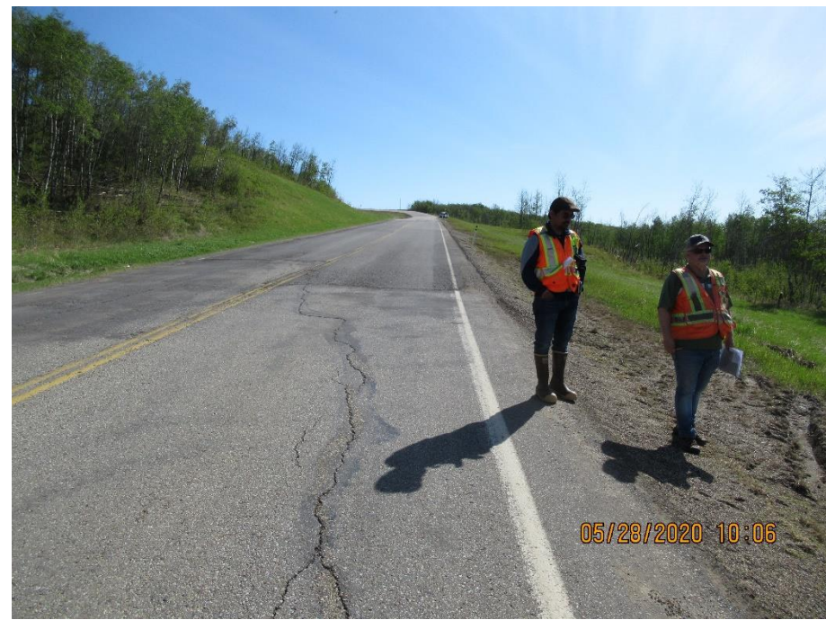
Photo 9. Looking northeast near the south end of the former south slide.
