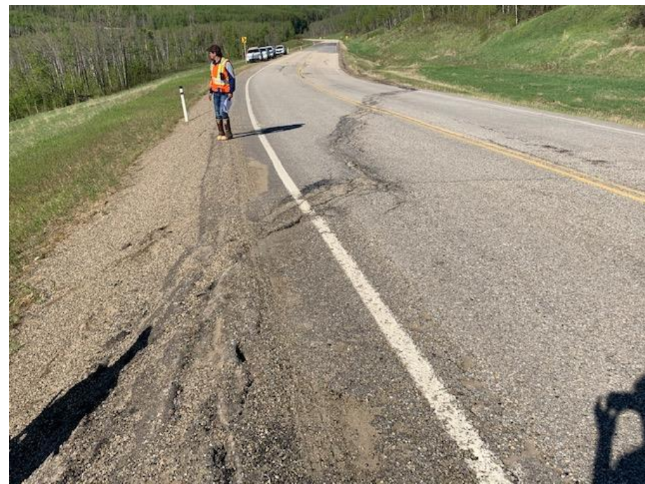
Photo 2. Looking southwest along Hwy 733 733 at sharp shoulder from successive overlays (former north slide).
