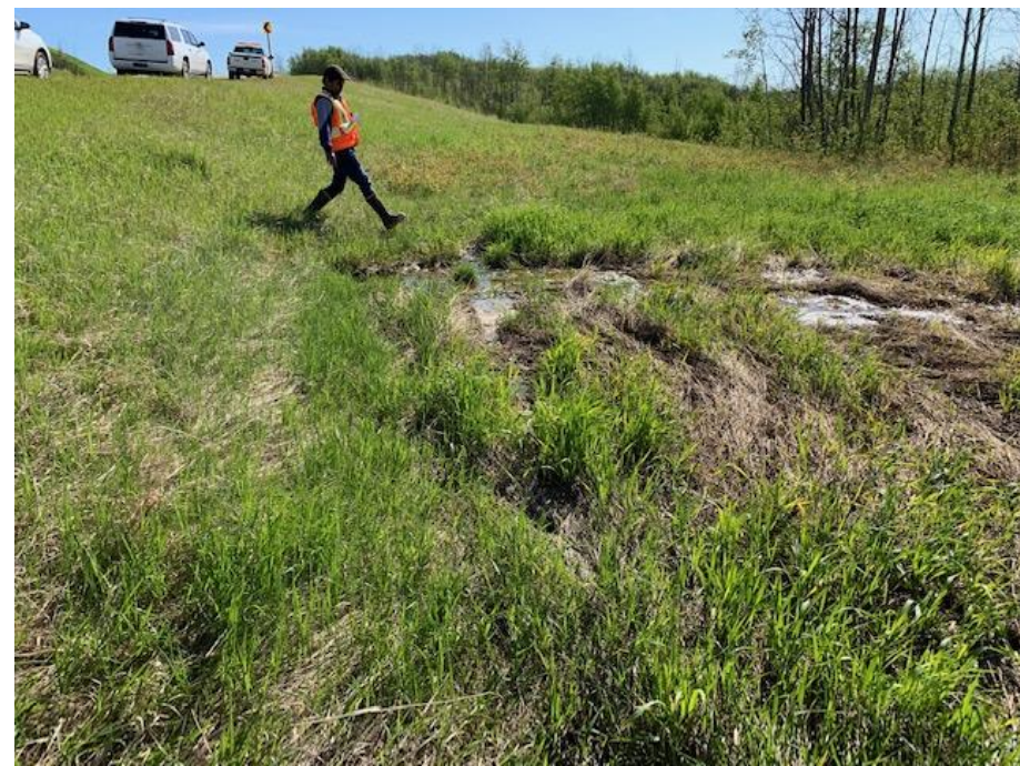
Photo 11. Looking east at ponded water in the south ditch.
