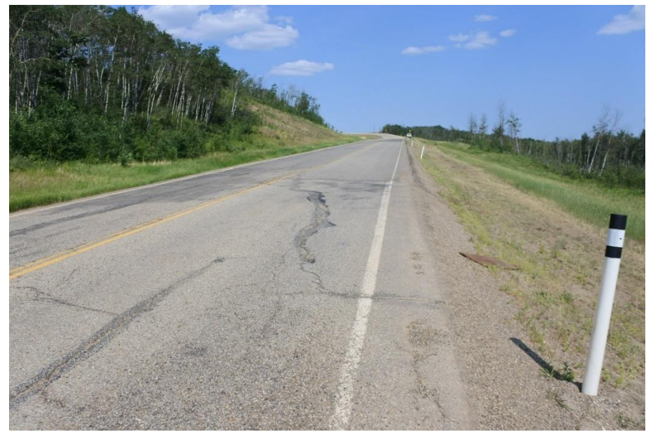
Photo 9. Looking northeast near the south end of the former south slide.
