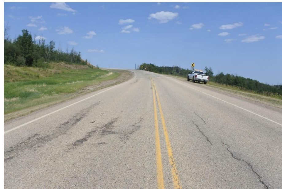
Photo 4. Looking northeast along Hwy 733 (former north slide).
