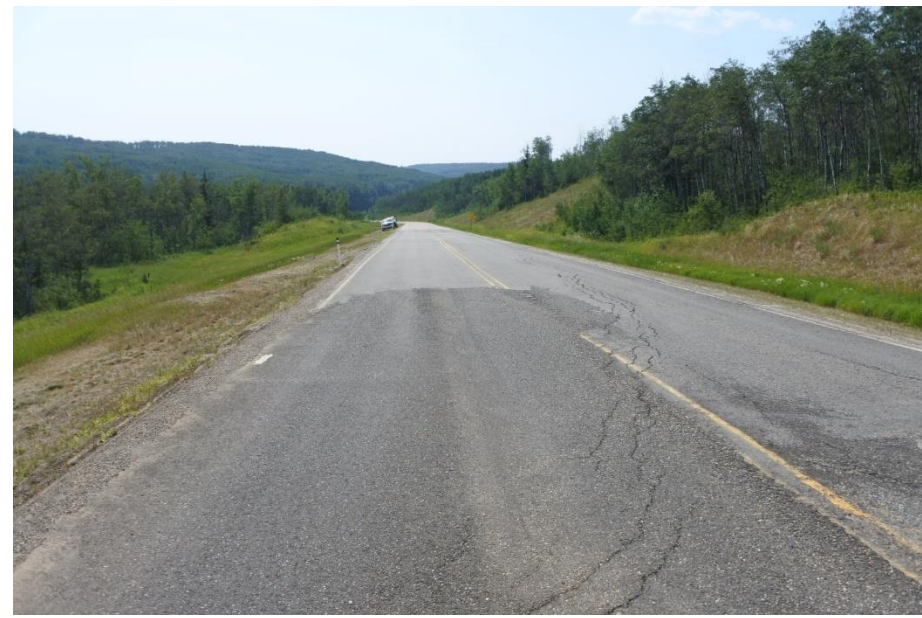
Photo 6. Looking southwest (former south slide).
