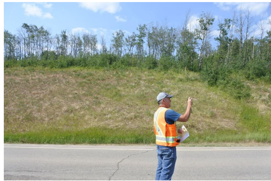
Photo 5. Looking northwest at backslope slump
