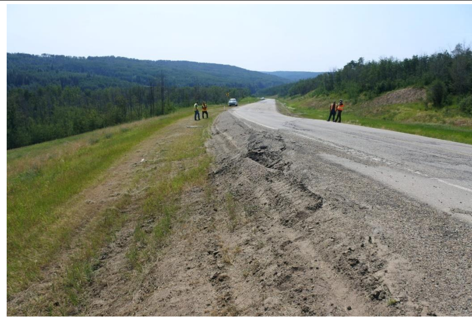
Photo 2. Looking southwest along Hwy 733 at sharp shoulder from successive overlays (former north slide).
