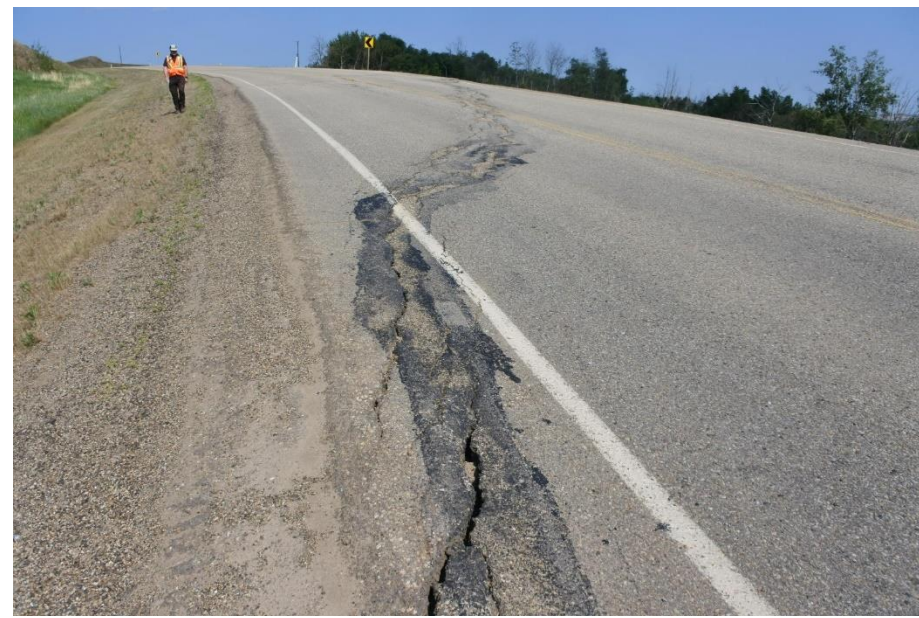
Photo 3. Looking northeast along Hwy 733 at scarp crack which extends into shoulder and embankment (former north slide)
