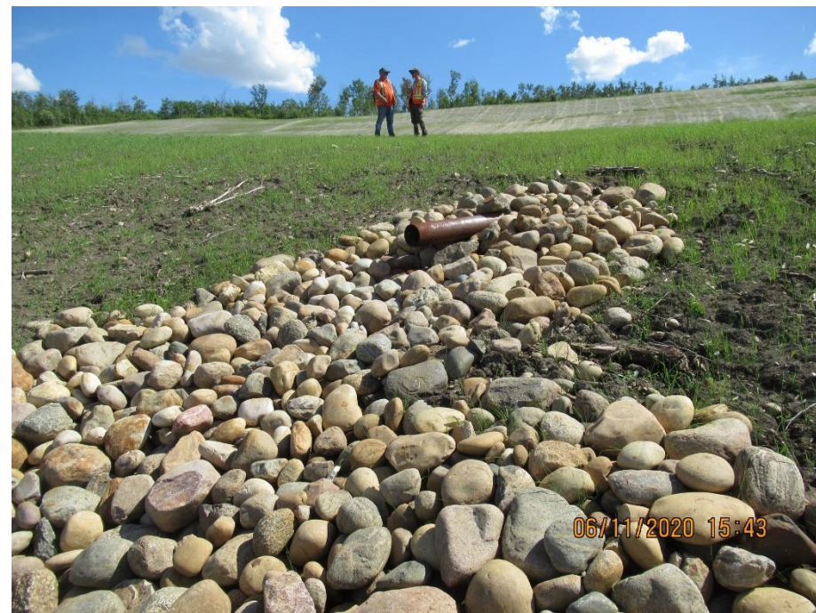
Photo 13. Drain outlet dripping water.
