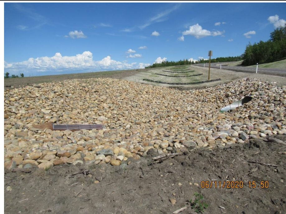
Photo 14. Looking east toward inlet of drop pipe and outlet of centreline pipe.
