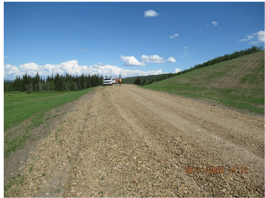
Photo 4. County road aligned over top of berm and finished with gravel surfacing.
