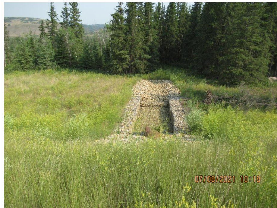
Photo 9. Looking north at gabion dissipation bowl at outlet of drop pipe.
