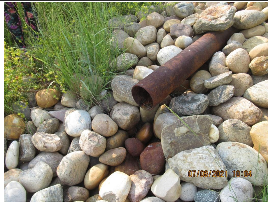
Photo 6. Seepage from drainpipe into West Riprap Channel.
