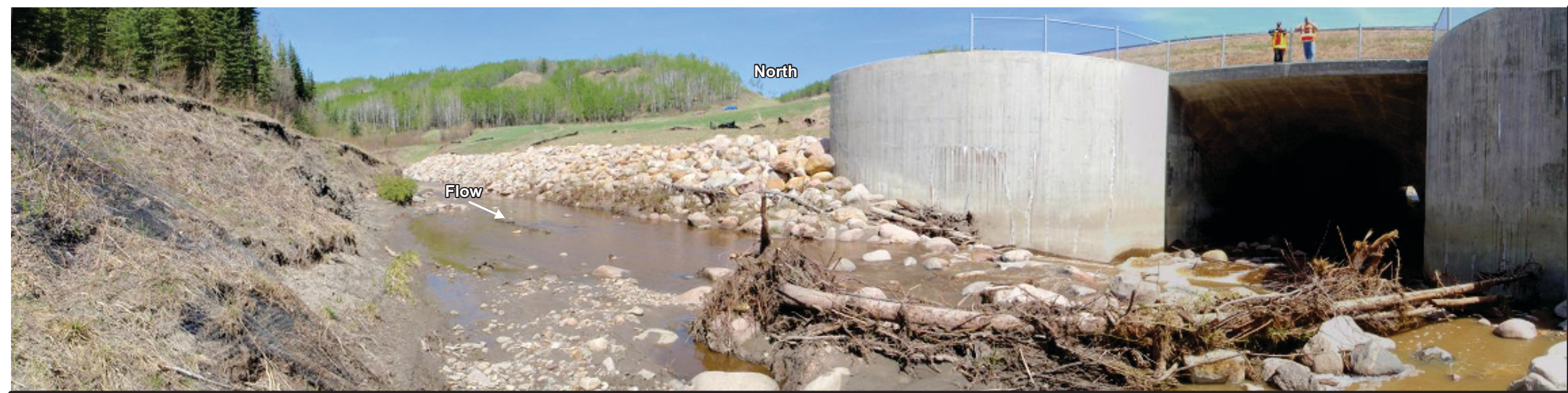
Photo 3b Looking upstream at Hamelin Creek and at Tributary Creek • Opposite bank and valley slope of Hamelin Creek was eroded steeply • Bank on highway side well protected by recent (2010) bank armouring • Previous (2010) repair work on upstream side of site still in good condition (right of photo) • Culvert Inlet and channel thorough-way looked unblocked
