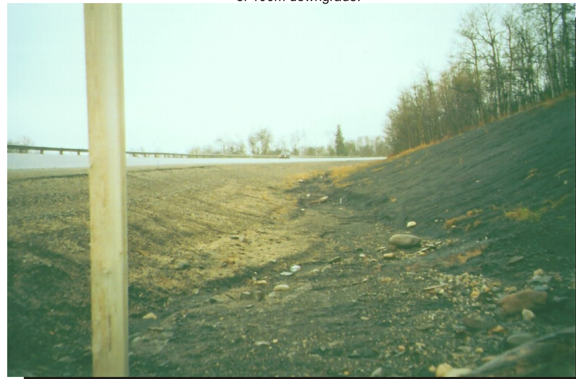
Photo 10 Looking upgrade north ditch erosion mildly severe along 3rd stretch
