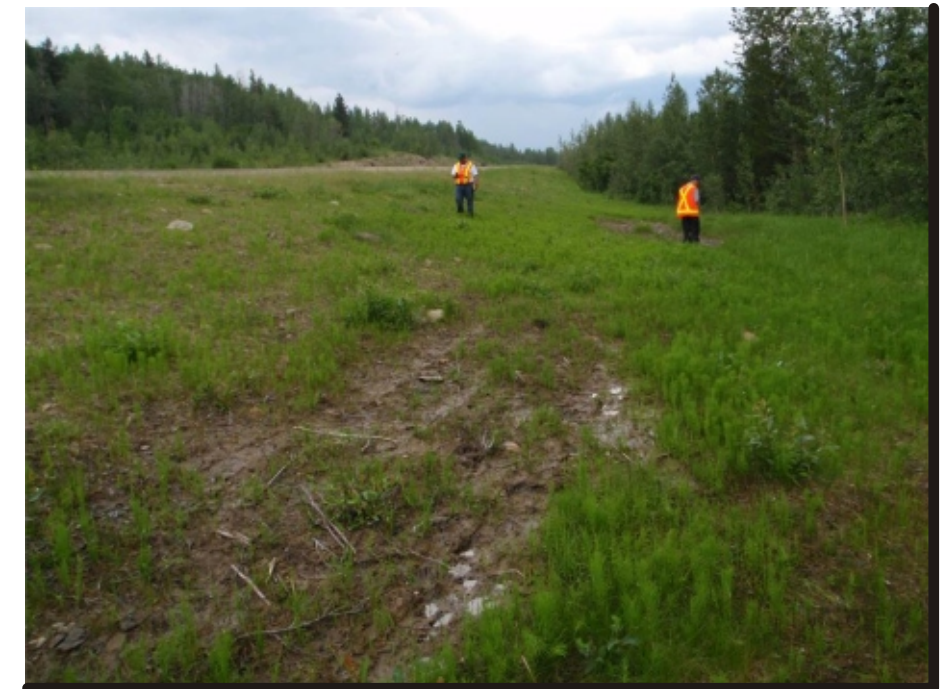
Photo 6 - Wet patches of sideslope fill adjacent to culvert outlet area can be observed. It can be indicative of seepage along base of fill - Need to check if potential severing or breakage of culvert maybe cause of seepage
