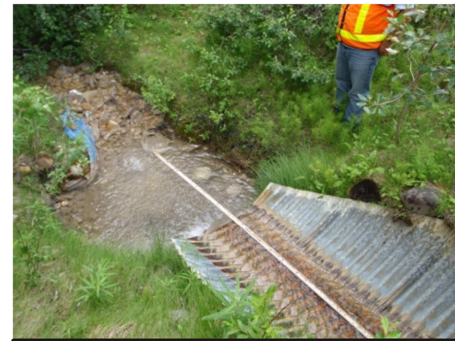
Photo 8 Culvert outlet - A drop of ground at culvert outlet will cause vertical erosion at outlet. Need to be infilled with adequate size granular fill to provide a smooth outflow apron. - De-icing pipe presnt
