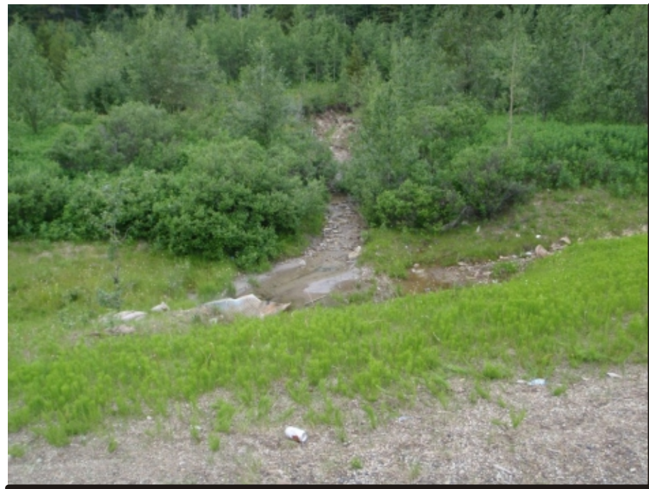
Photo 4 Centreline culvert inlet at south flank of slide - Steady water inflow from stream
