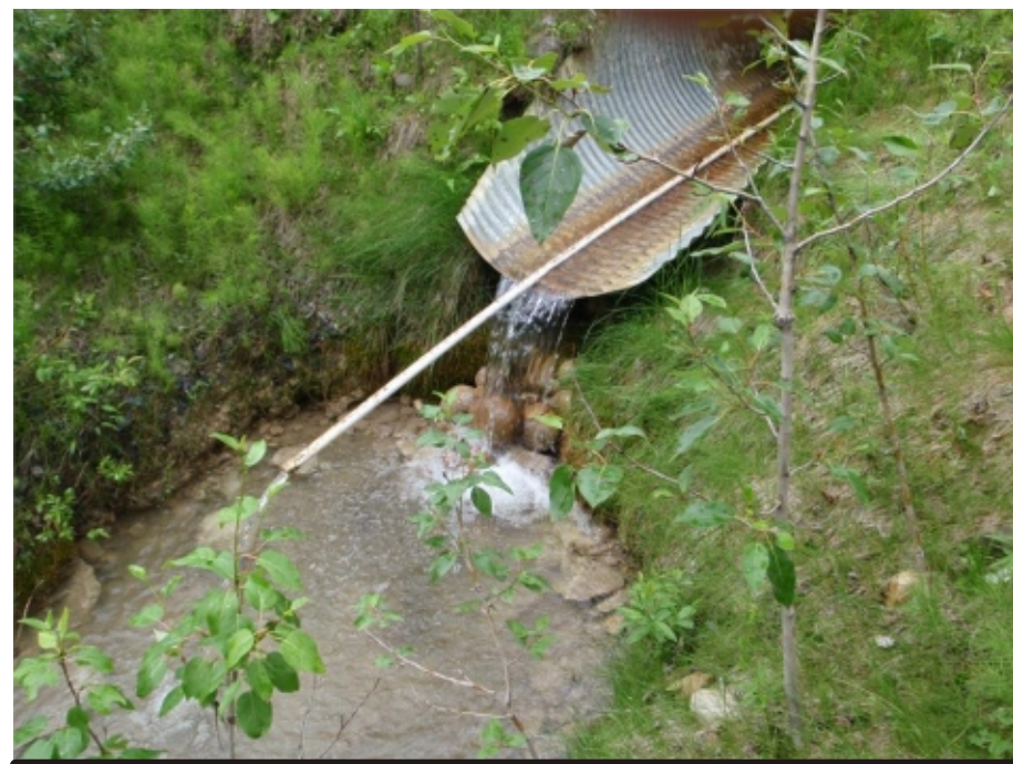
Photo 7 Culvert outlet - A drop of ground at culvert outlet will cause vertical erosion at outlet. Need to be infilled with adequate size granular fill to provide a smooth outflow apron. - De-icing pipe presnt
