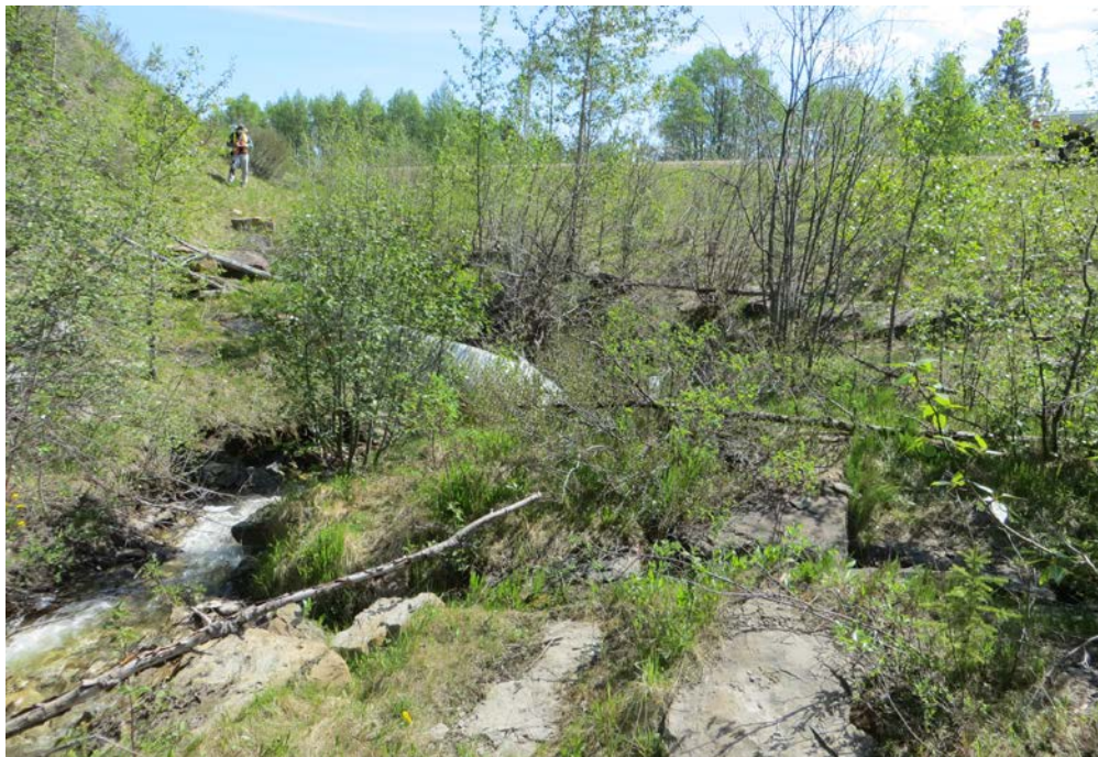
Photo 2 – Looking east at the lifted/undermined culvert inlet and highway embankment.
