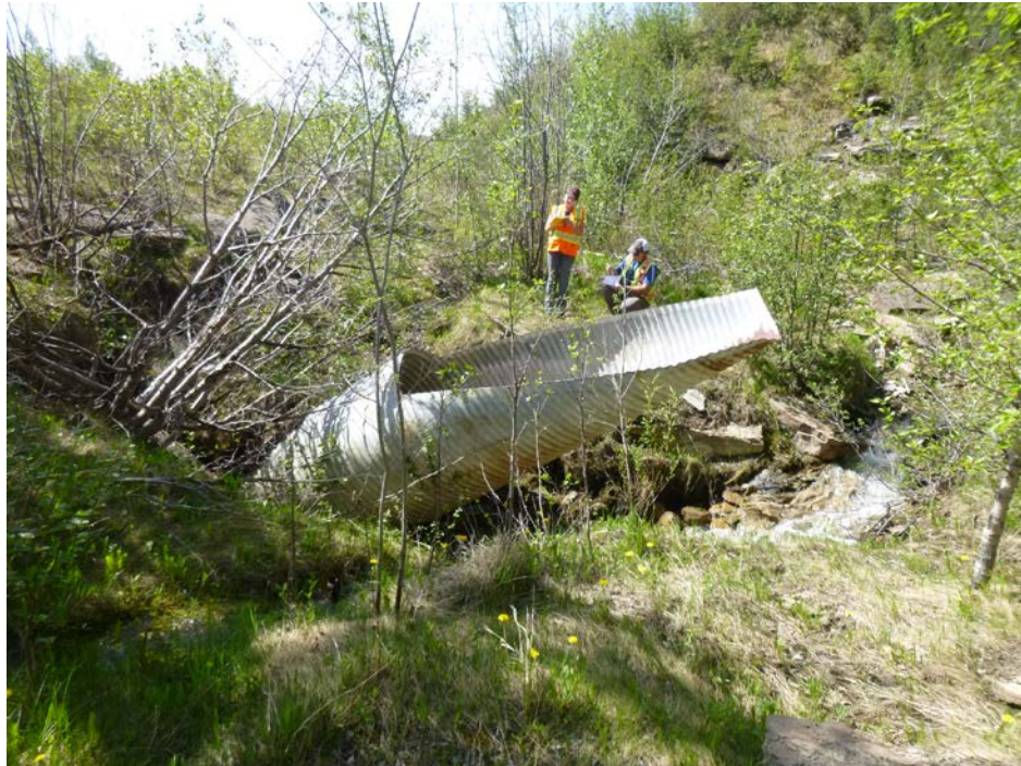
Photo 5 – Looking south at the lifted/undermined culvert inlet.
