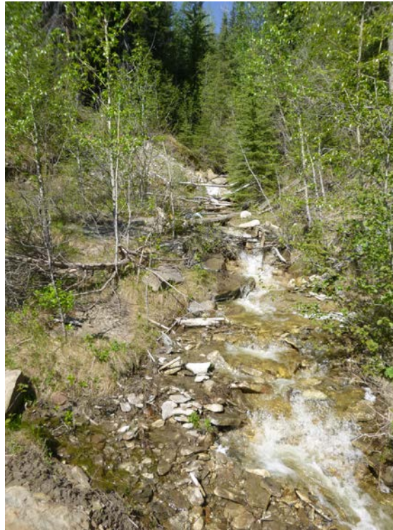
Photo 1 – Looking upstream (west) at the creek flowing into the culvert – no significant erosion.
