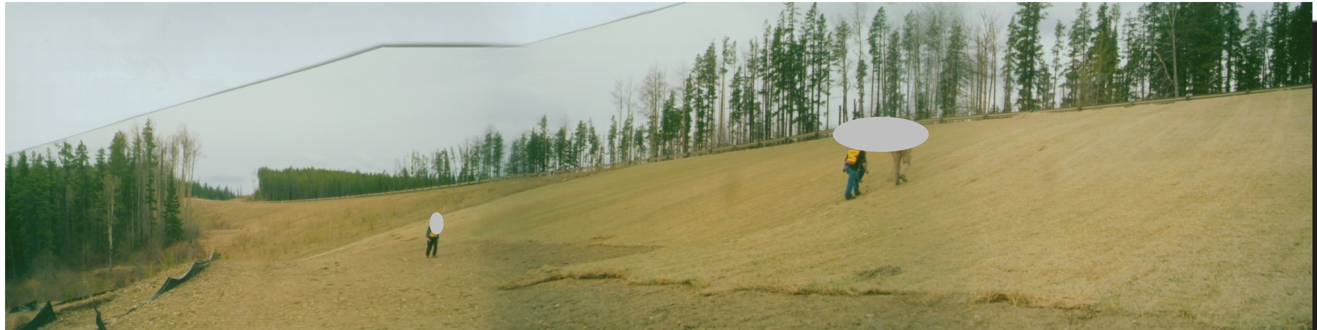
Photo 4 Looking south along toe of slope - Slope reconstruction to 3H:1V with pitrun material - Erosion control matting material with high intensity seeding (3 times normal rate) - toe drainage outlet at left corner of photo (at far end of silt fence)
