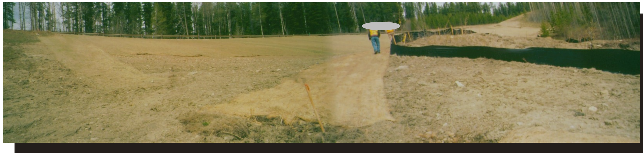
Photo 5 Looking north from south edge of toe area - First drainage outlet (of tile system at base of toe key at center bottom of photo) yield continuous flow - silt fence along perimeter at bottom toe edge of slope reconstruction
