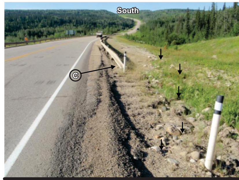
Photo 1d Propagation of headscarp crack • Headscarp crack has imprinted onto backslope ditch area
