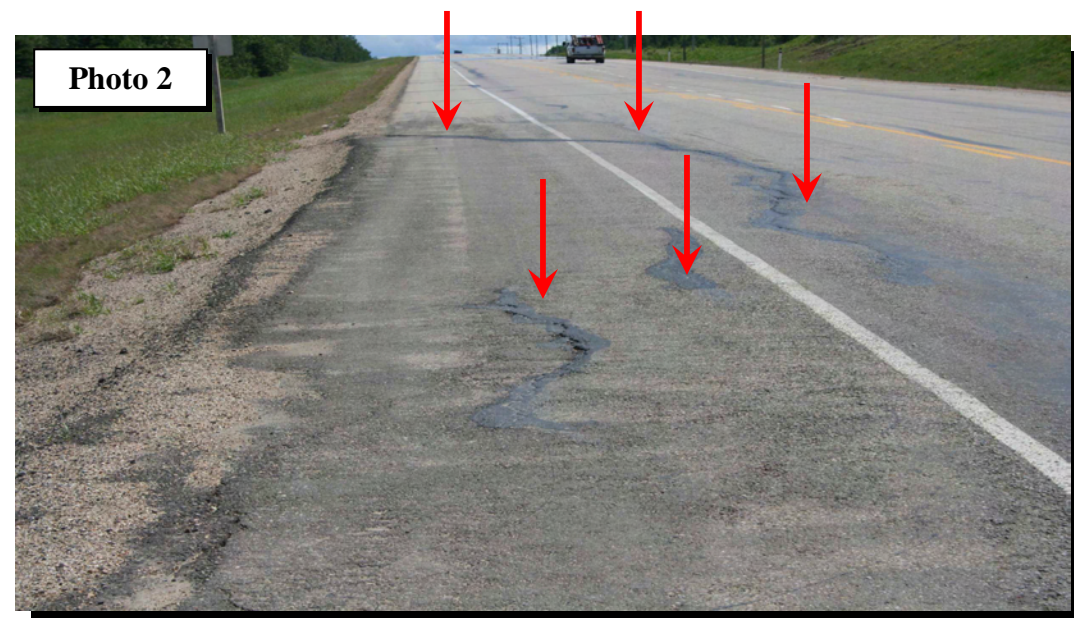
Another view of pavement crack
