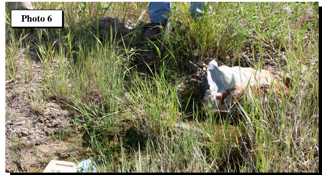
Outlet for exist of groundwater through a culvert spout at edge of toe key berm
