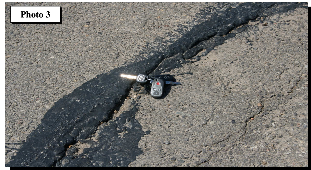
Close up view of crack
