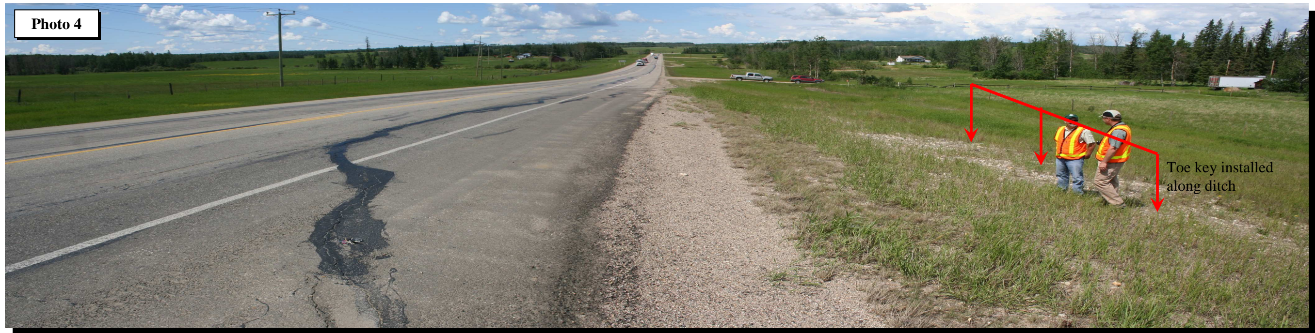
Looking west (away from valley-view) - Reflective crack of pavement - Another view
