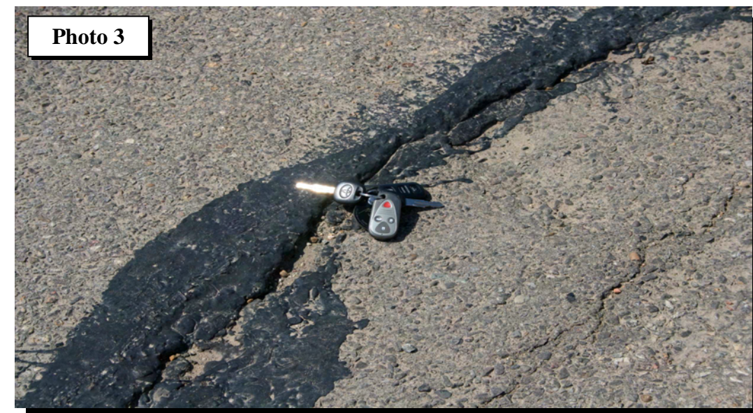
Close up view of crack
