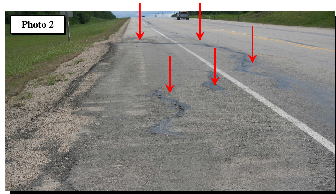
Another view of pavement crack
