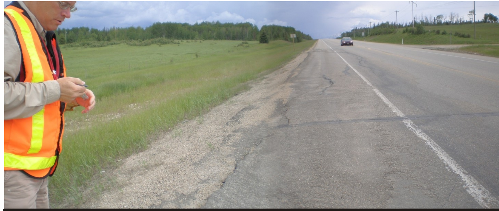
Photo 1 Looking East (towards Valleyview) along westbound lane - Pavement crack from headscarp from sliding of low embankment. The crack extended about 1m beyond shoulder line - Breadth of headscarp crack about 30m in length along roadway - Pavement cracking and minor subsidence has progressively stabilized since 2001 (granular toe key with woven geotextile underlay) Continual operation of roadway is acceptable to maintenance forces
