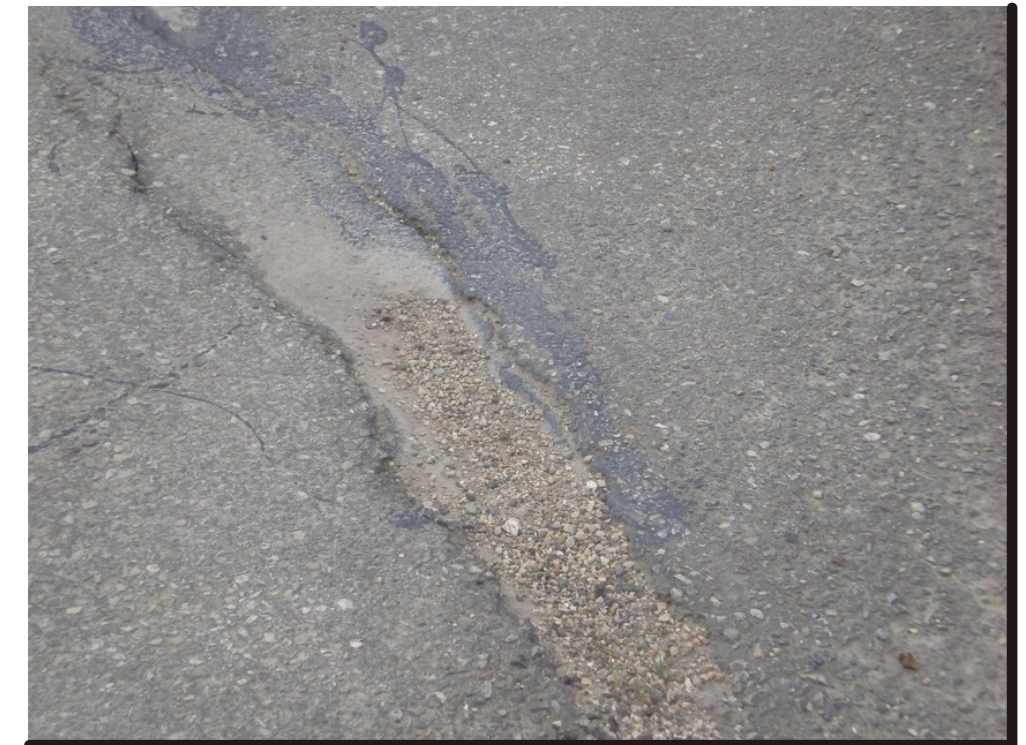
Photo 2a Minor reflection of cracks that was patched over and sealed
