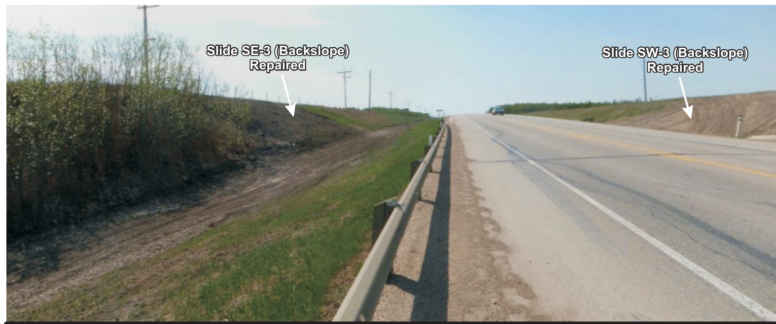
Photo 3a Looking south (at top of upland) along east ditch Repaired (SE-3) Slide at upland verge Repaired (SW-3) Slide at upland verge at opposite ditch
