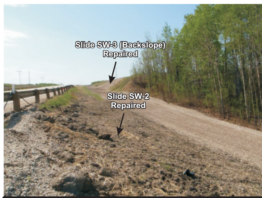
Photo 5c Looking south along west ditch SW-2 along sideslope SW-3 along verge of valley wall
