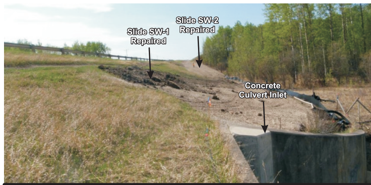
Photo 5 Looking south along west ditch (upstream side of culvert) culvert inlet A view of SW-1, SW-2 Repaired Slides
