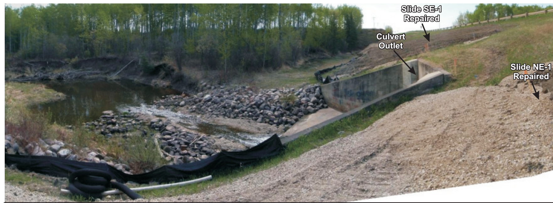
Photo 2a Another view at top elevation of culvert outlet Repaired Slides NE-1 & SE-1
