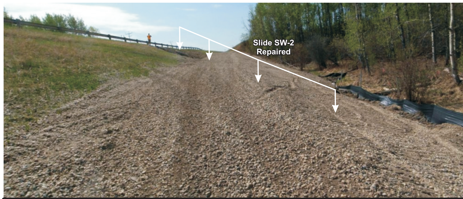
Photo 5b Looking south along west ditch SW-2 along sideslope SW-3 along verge of valley wall
