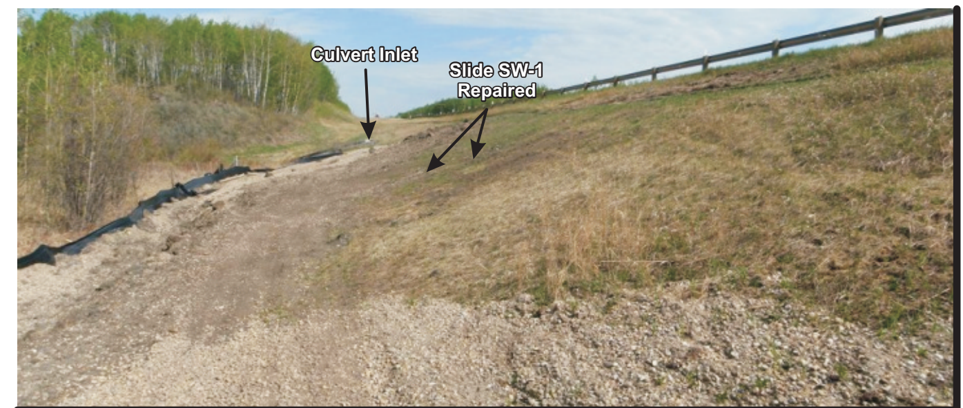
Photo 5a Looking north along west ditch (upstream side of culvert) culvert inlet SW-1 just adjacent to Wing-wall of culvert
