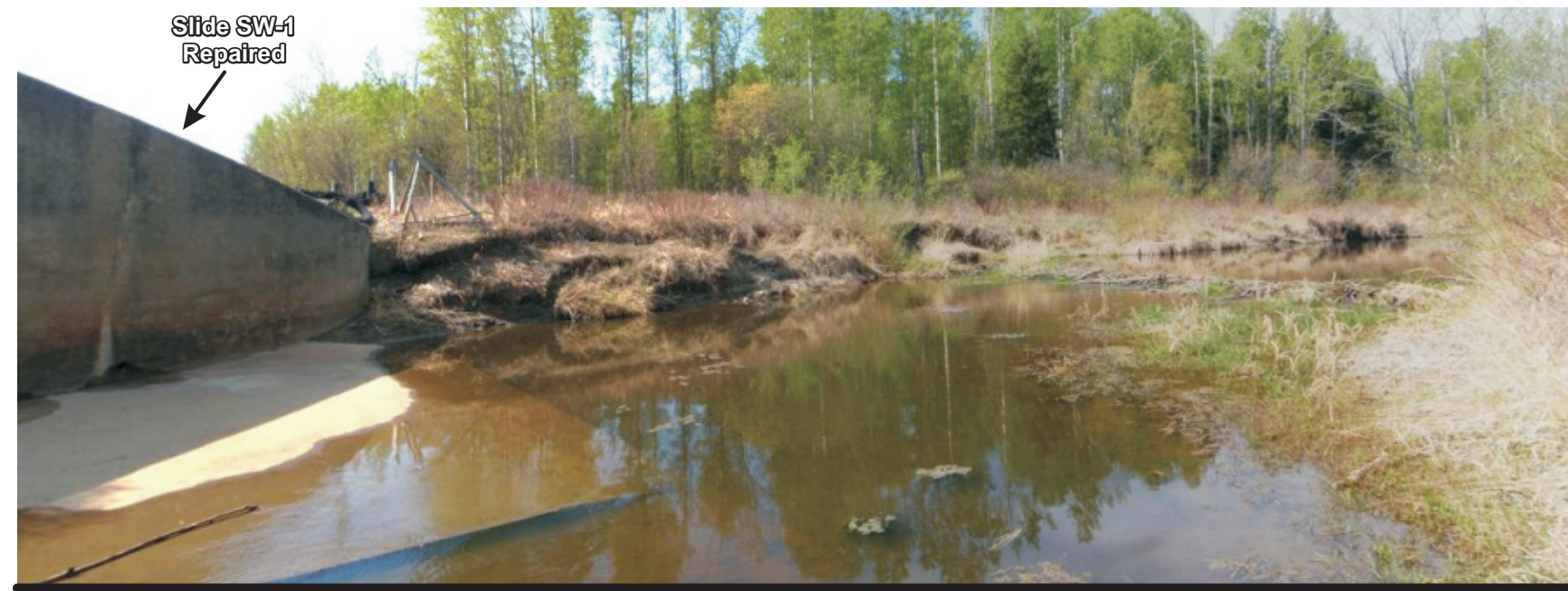
Photo 4 Looking west at upstream (south) bank adjacent to culvert inlet Repaired Slide (SW-1) just adjacent to bank and above headwall
