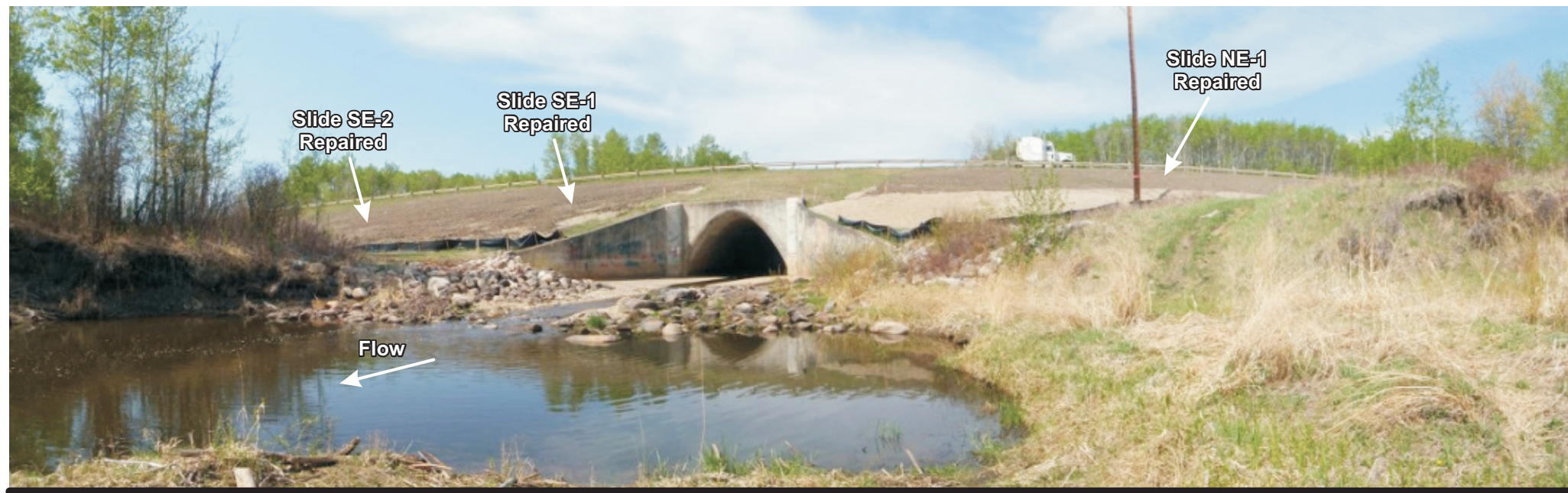
Photo 2 Looking west at outlet of culvert (downstream) and sideslope Another view of Repaired Slides NE-1, SE-1 and SE-2
