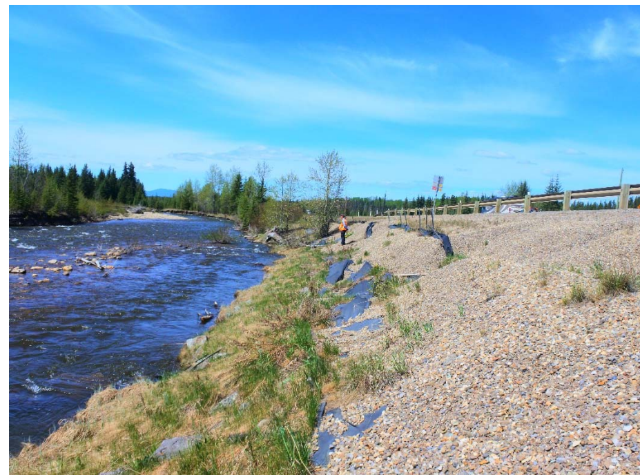
Photo 5. Looking west along the toe of the embankment. Note the grass covered riprap and the gully in the crushed gravel embankment that is overtop woven geotextile.
