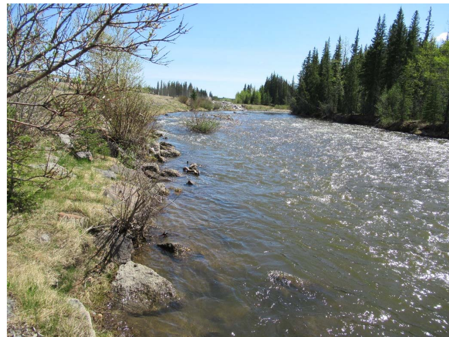
Photo 6. Looking east along the toe of the south highway. No significant toe erosion here.
