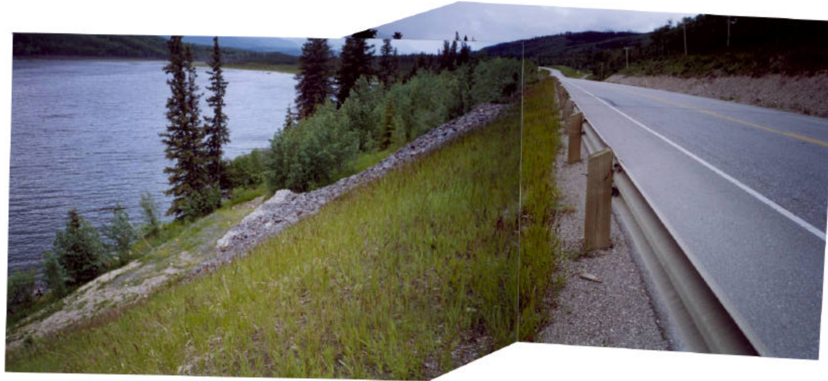
Photo 1 Looking north towards Grande Cache - Repaired slope in relation to roadway
