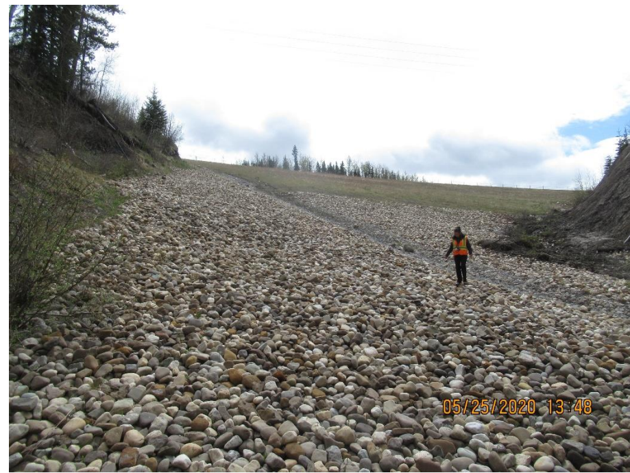
Photo 21. Looking south at beginning of crotch ditches and gabion mattresses on the north side of the highway.
