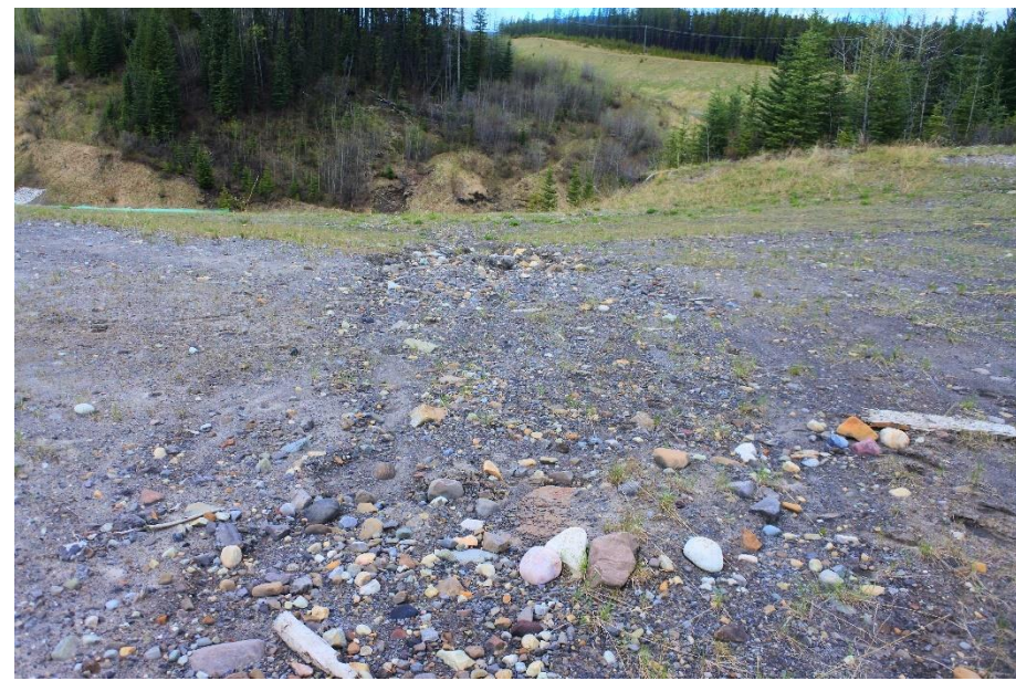
Photo 5. Looking west at area eroded by surface water which appears to have been from an overflow over the rip rap due to the culvert being frozen/blocked.
