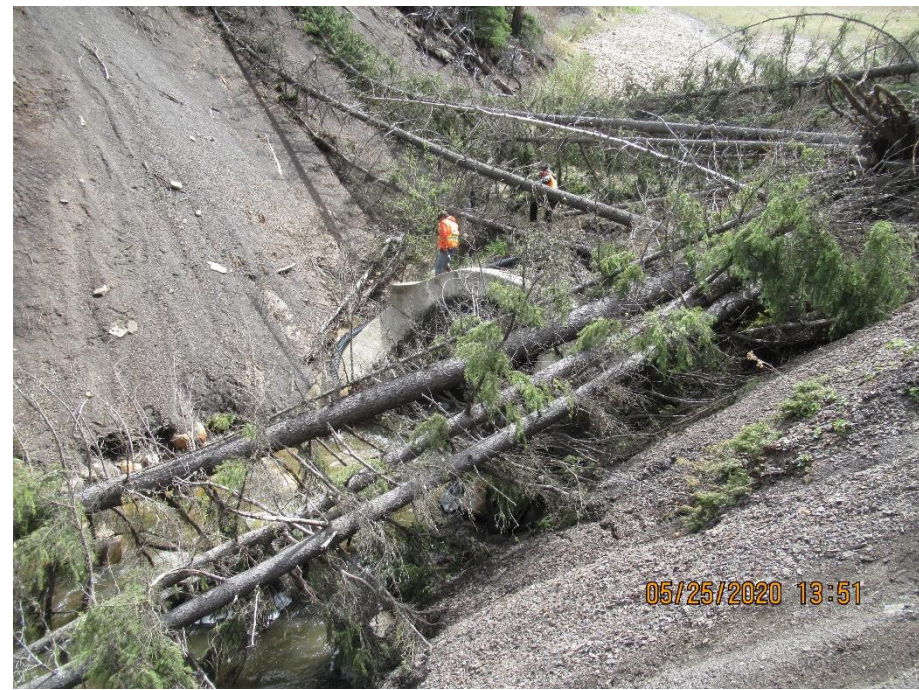
Photo 22. Looking southeast at the culvert outlet covered by fallen trees.
