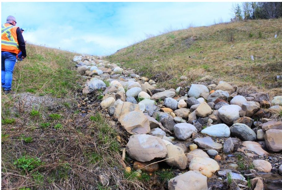
Photo 18. Looking northeast at the east crotch ditch that has some erosion along its sides.
