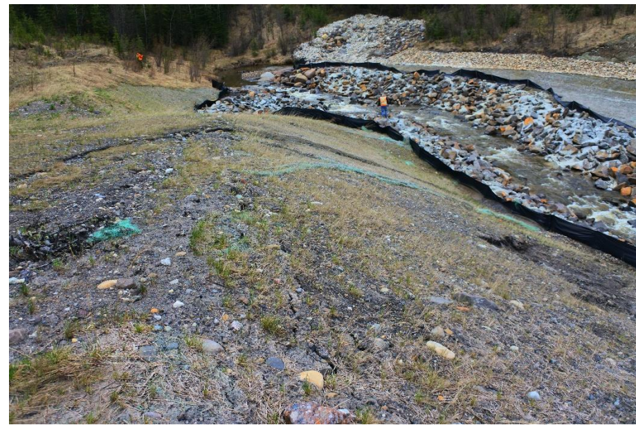
Photo 10. Looking southwest towards dissipation bowl, some slight surficial erosion.
