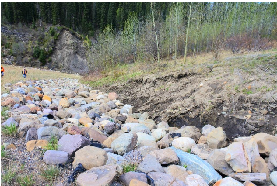
Photo 24. Looking northwest at erosion occurring on the north side of the east crotch ditch.
