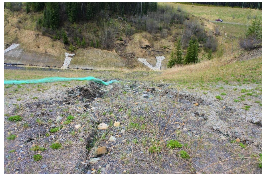
Photo 6. Looking south at slope east of main channel where erosion control covering had been swept off from wind.
