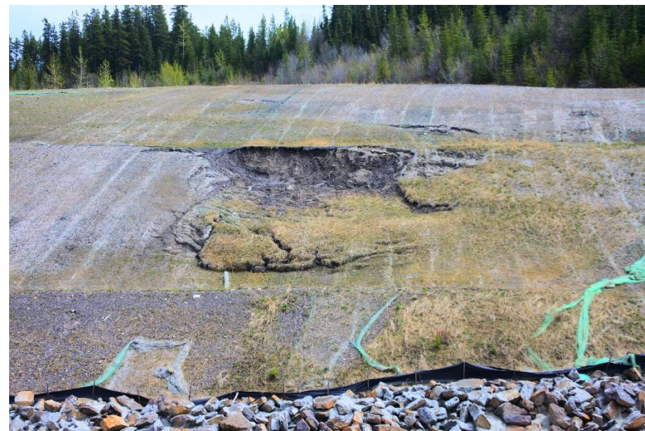
Photo 15. Looking east at a slump on the east slope.
