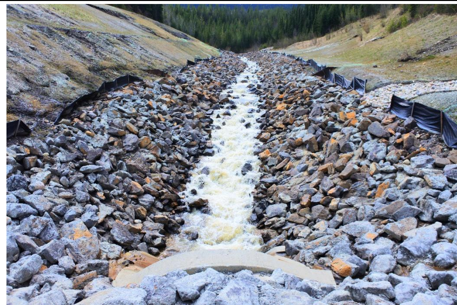
Photo 16. Looking south at the main channel standing on top of the culvert inlet.
