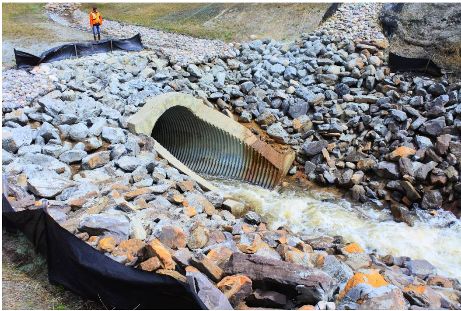
Photo 17. Looking northeast at the main channel culvert inlet and east crotch ditch.
