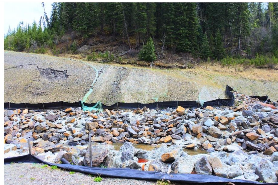
Photo 12. Looking east at small slump.
