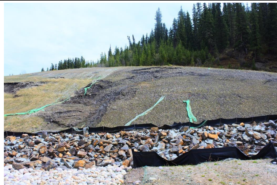
Photo 13. Looking east at the slumped areas on the east side slope of the main channel.
