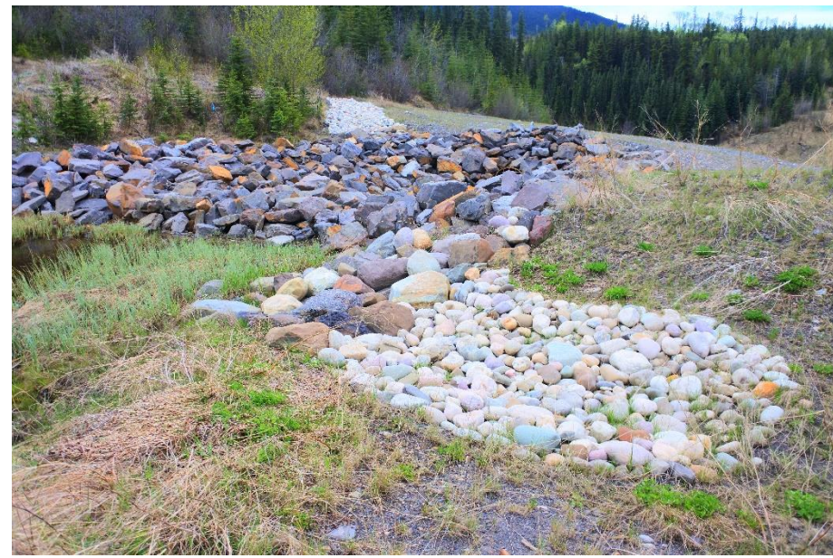
Photo 4. Looking southwest at the added swale adjacent and downslope of the culvert inlet.
