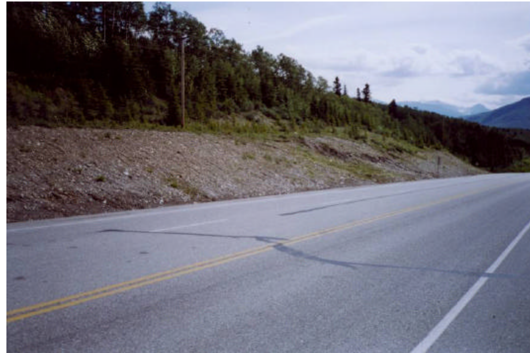
Photo 1 Looking downgrade (away from Grande Cache) - Seepage noted along backslope
