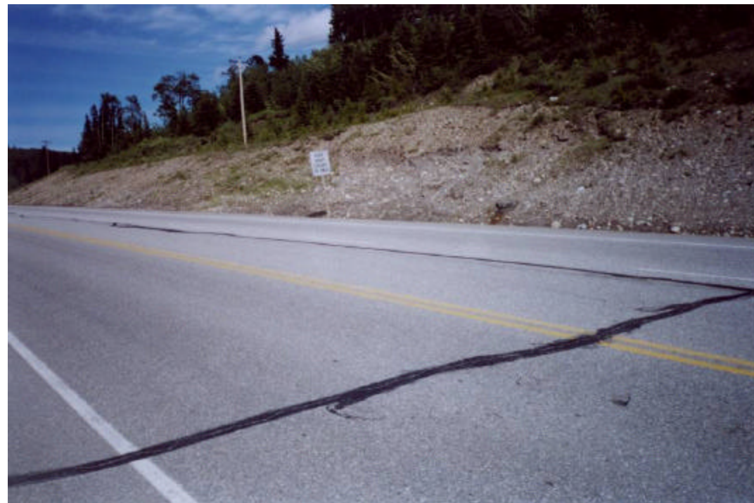
Photo 3 Looking upgrade (towards Grande Cache) - Seepage noted along backslope
