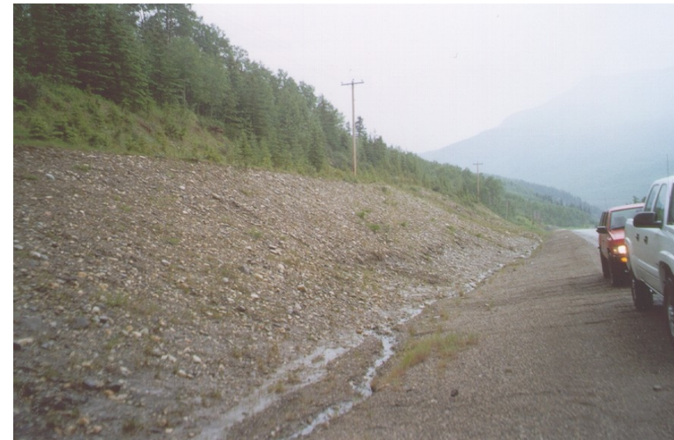
Photo 4 Looking south and downgrade. 1) Minor Toe bulging and sloughing toward ditch
