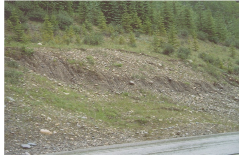
Photo 2 Close-up at slumping area.
