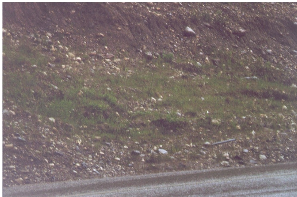
Photo 3 Close-up 1) Minor sloughing at horizontal drain pipe (possibly severed)
