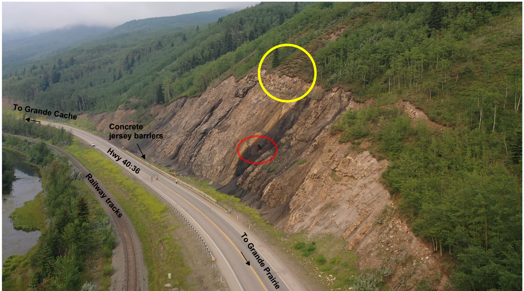
Photo 1 Overview of the GP036 site, indicating Hwy 40, railway tracks, concrete lock blocks, and decommissioned coal mine shaft entrance (indicated by red circle). Note the overburden above the brow of the rock slope is failing (yellow circle). Photo taken July 21, 2021 facing south.
