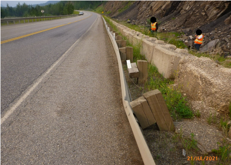
Photo 2 Deflection in guardrail caused by a particle falling down the slope. Photo taken July 21, 2021 facing south. Note some lock blocks are deteriorating.
