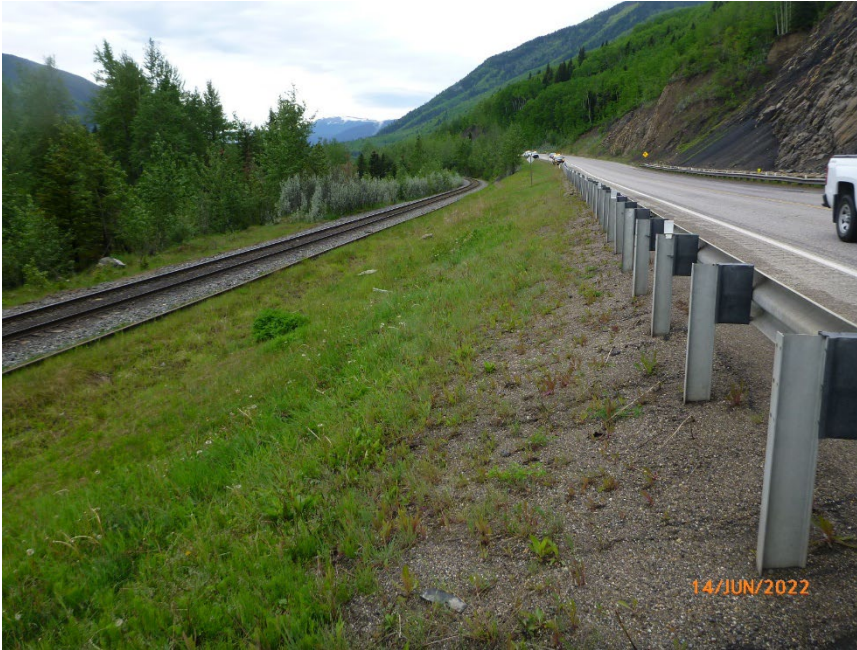
Photo 9 Some rockfall particles on east side of Hwy 40:36 between guardrail and railway tracks. These particles may have been cleaned off highway, but AT has reported rockfall particles making it across highway. Photo taken June 14, 2022, facing southwest.
