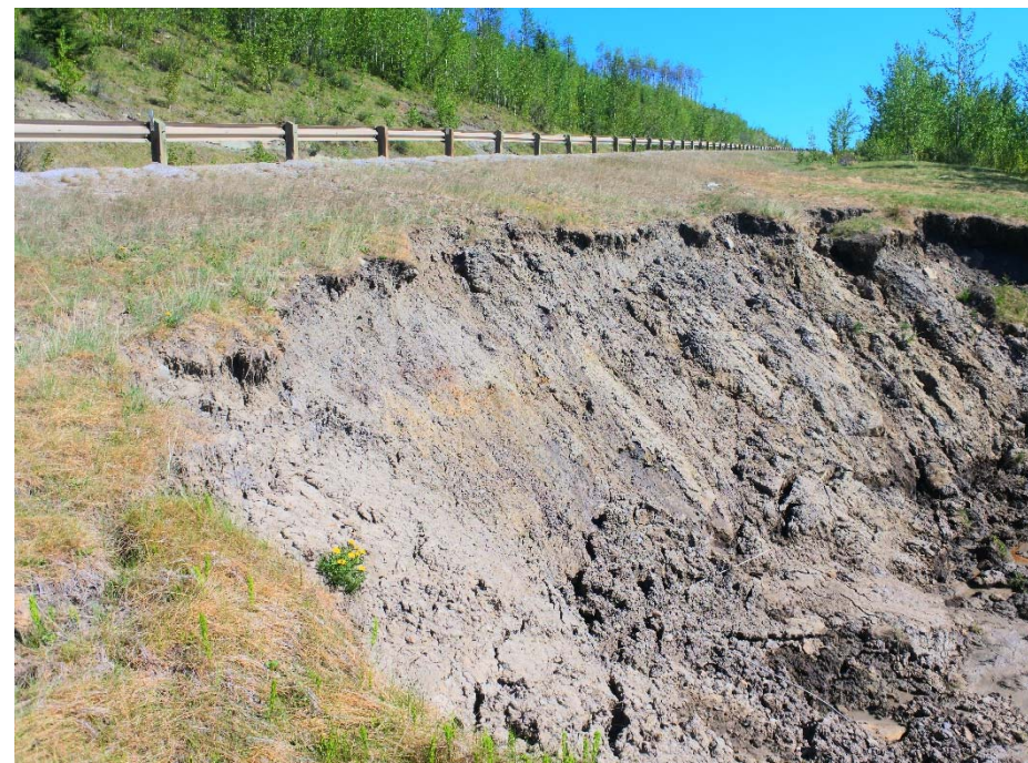
Photo 1. Looking northeast at the main scarp.
