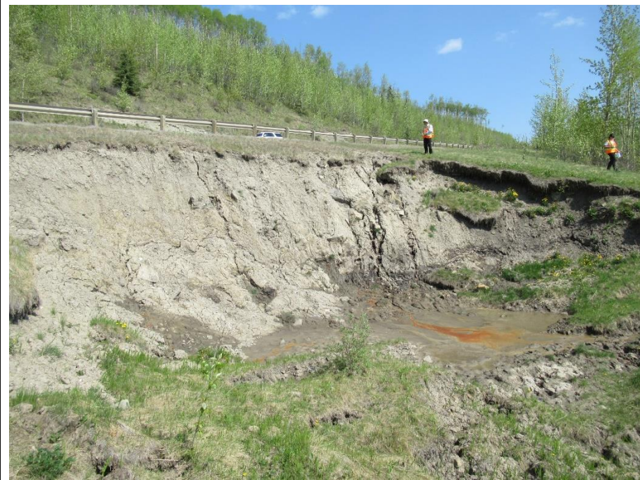
Photo 1. Looking northeast at the main scarp.
