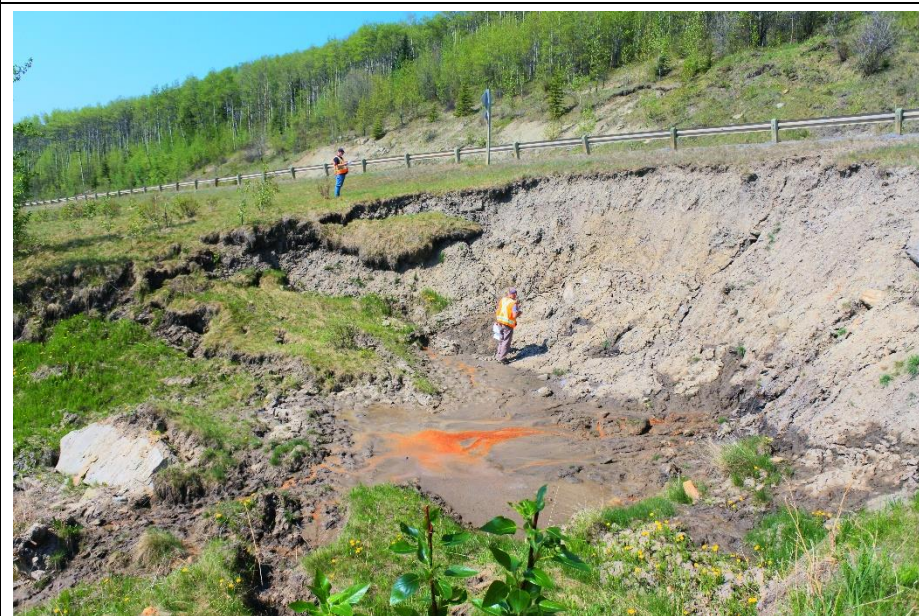
Photo 6. Looking northwest at the main scarp.
